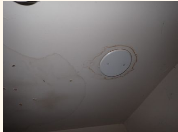
Moisture Stains in Ceiling of Furnace Closet
