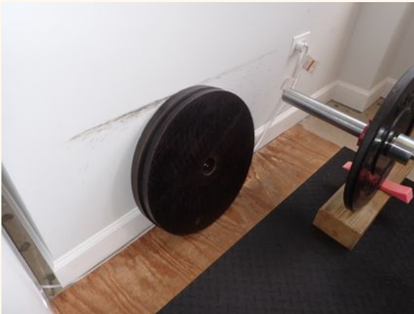
Damaged Wall Finishes
