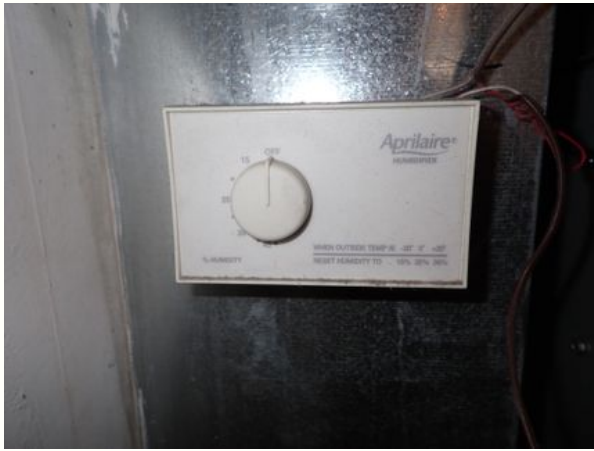
Humidistat Located in Furnace Closet
