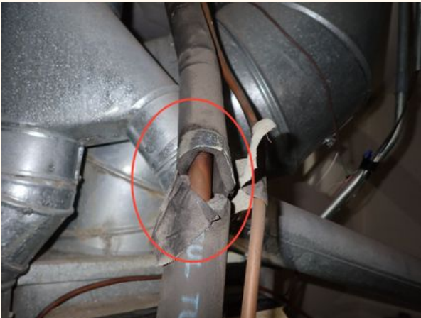
Interior Gap in Insulation
