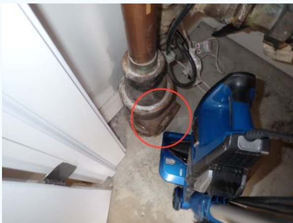
Clean-out in Unit
