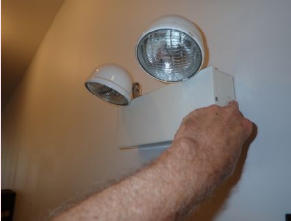
Non-operational Lights in Unit
