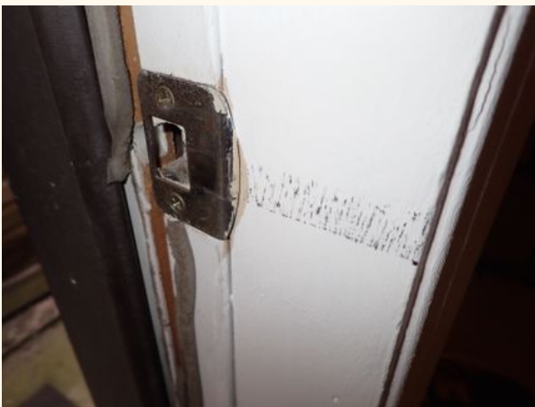
Damaged Side Doorframe
