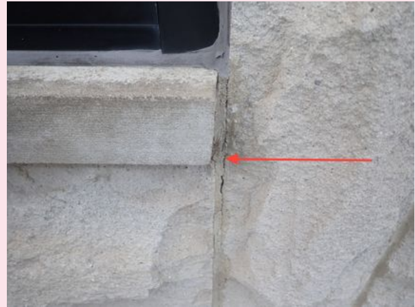
Cracked Mortar Joints and Damaged Masonry Below Stone Sill
