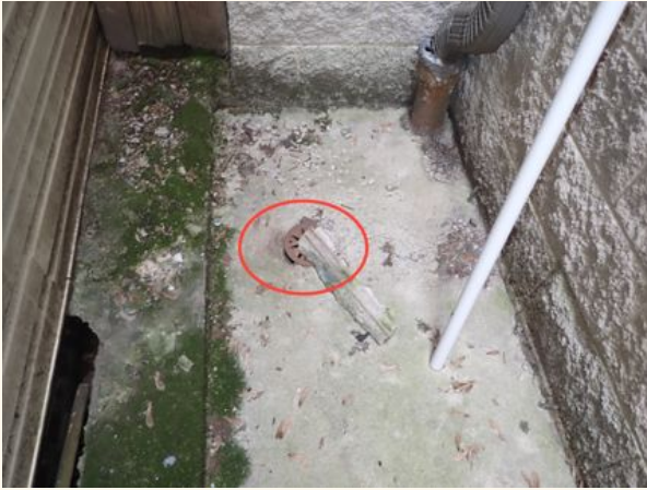
Domed Style Cover Needed on Side Drain
