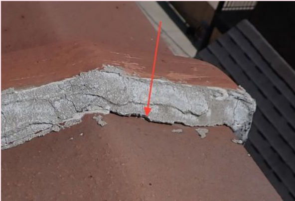
Unsealed Cap Joints
