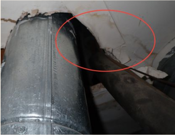
Stains by Piping in Ceiling of Furnace Closet
