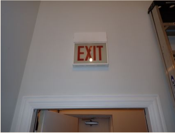
Unlit Exit Sign
