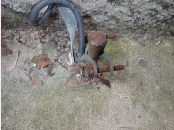
Improper Clamp on Ground Rod
