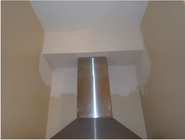
Unfinished Walls in Kitchen Area
