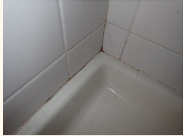
Mold Noted in Joints
