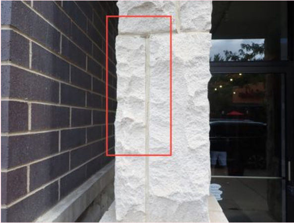
Cracking in Front Column Joints
