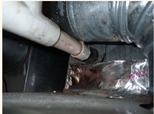
Air Noted Leaking from Gaps in Condensate Drain Penetration
