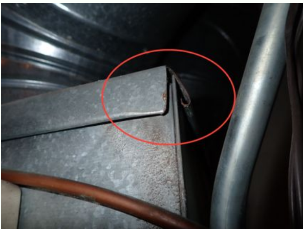
Air Noted Leaking from Gaps in HVAC Ductwork
