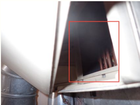
No Water Pad Inside Humidifier
