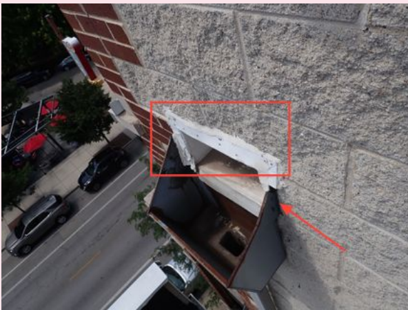
Newer Sealant on Top - Older Sealant and No Flange on Sides
