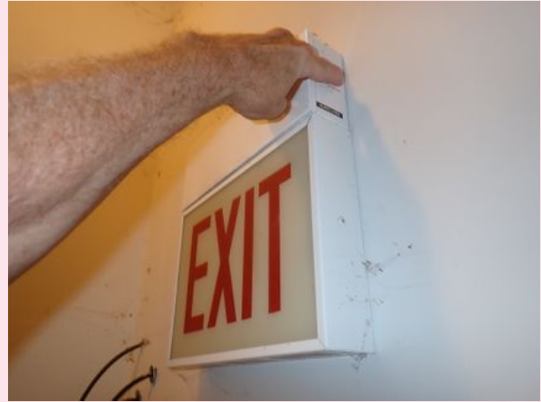
Non-operational Lights on Exit Sign
