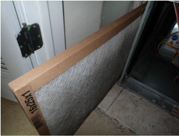
One Inch Thick Filters used in HVAC System
