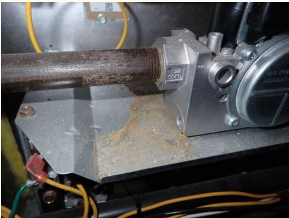
Leakage Stains in Furnace
