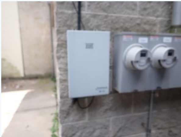
Low Voltage Communication Equipment
