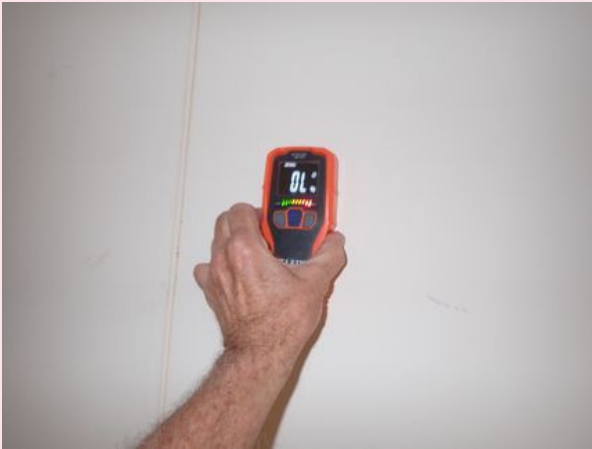
Saturated Humidity Levels in Walls
