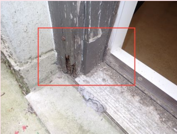
Deteriorated Side Doorframe
