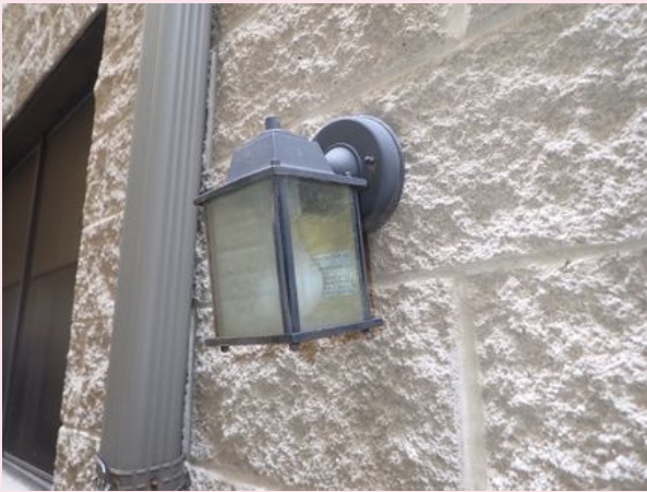
Loose and Unsealed Fixture
