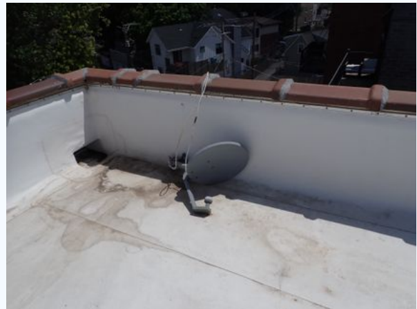
Loose Satellite Dish on Roof
