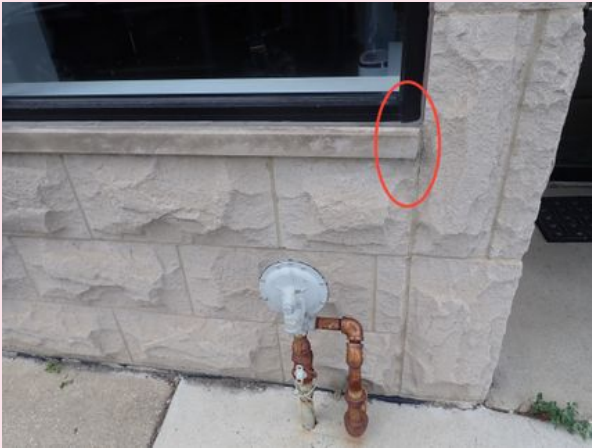
Cracks in Corners of Stone Sills
