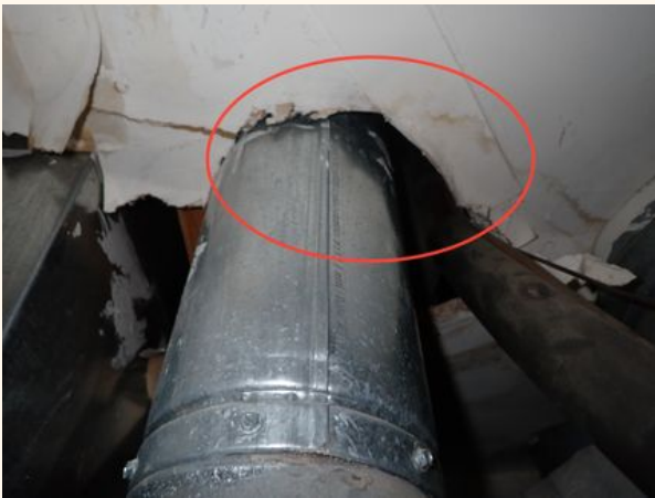
Unsealed Gaps in Furnace Closet
