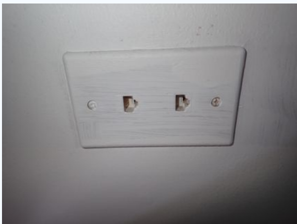
Low Voltage Communication Equipment
