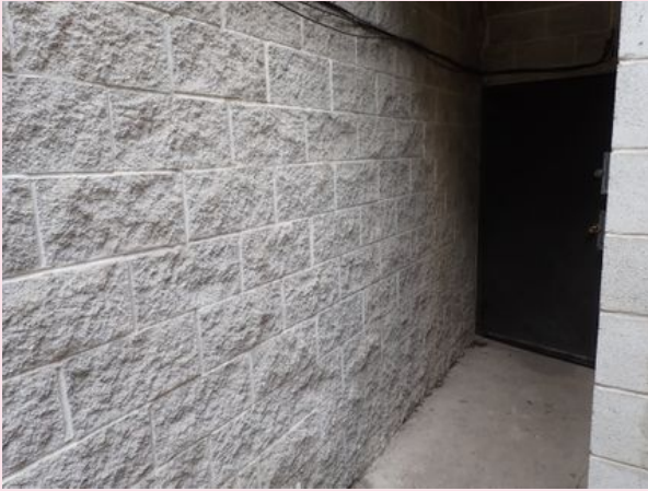
Unsealed Block Walls
