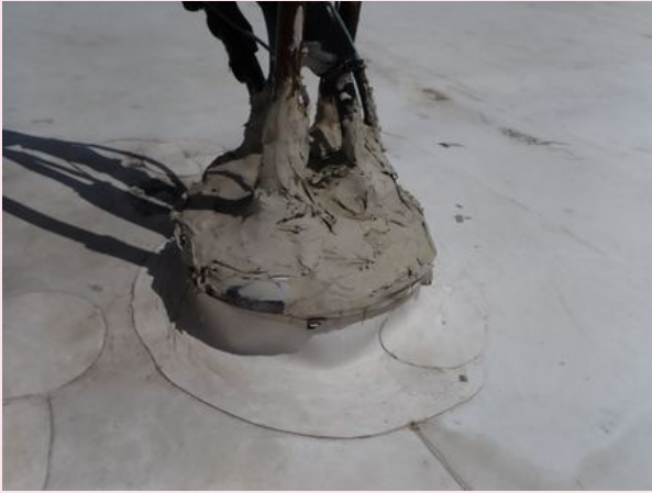
Multiple Layers of Sealant on Roof Boots
