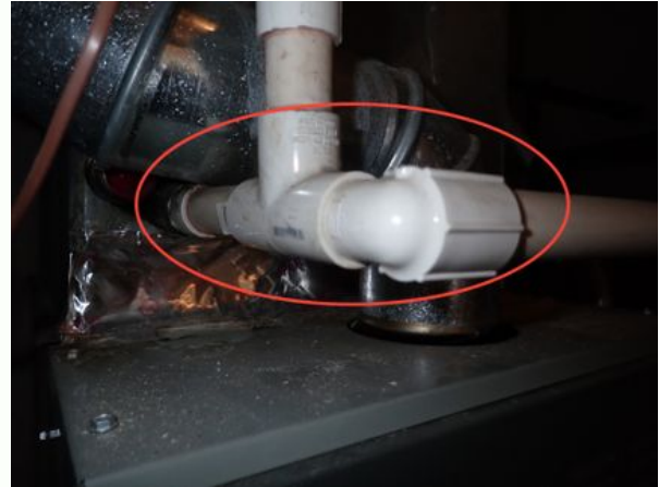
Trap Missing on AC Condensate Drain
