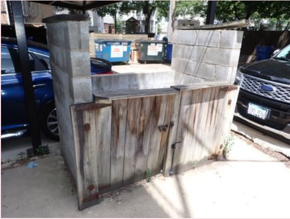
Deteriorated Refuse Screen
