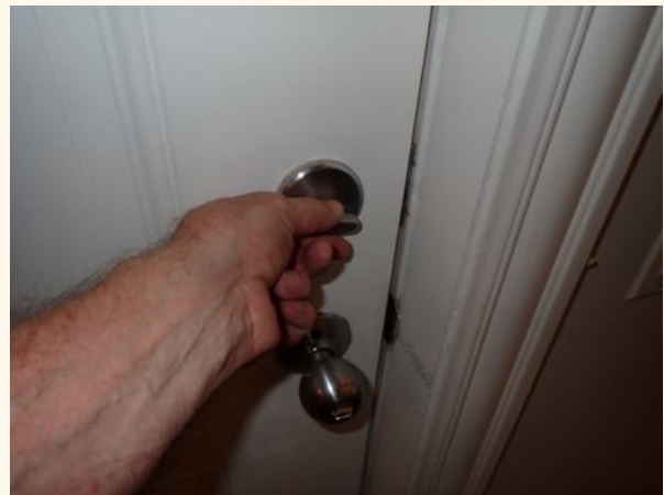
Difficult to Latch Side Entry Door
