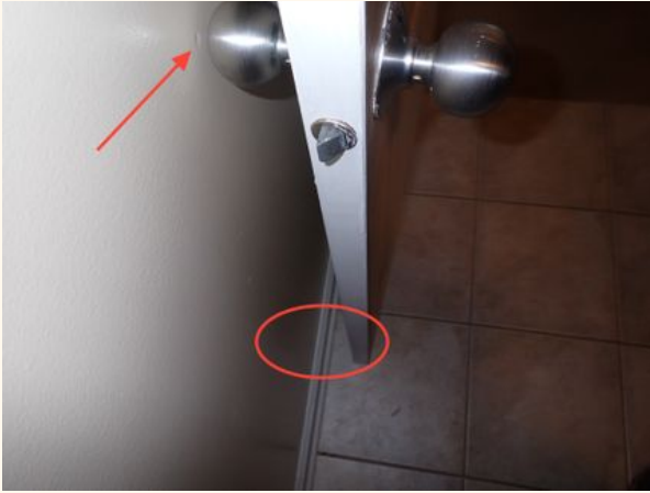
Damaged Wall - Missing Doorstop
