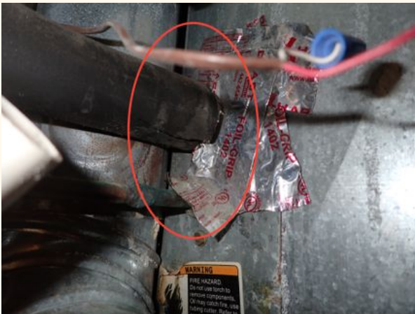
Air Noted Leaking from Gaps in Lines Set Tubing Penetration
