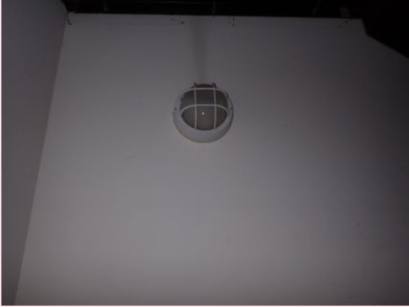
Dark Lights in Rear Stairwell
