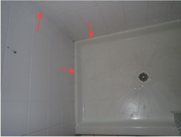
Corner Tile Joints Prone to Cracking
