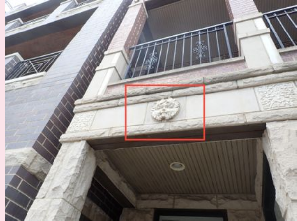
Cracking Around Medallions
