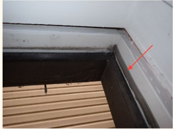
Low Quality and Missing Weatherstripping
