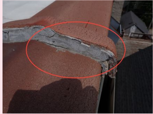
Cracked and Open Joints with Caulk Smears
