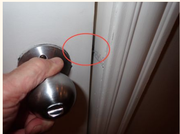
Latch Damaging Doorframe
