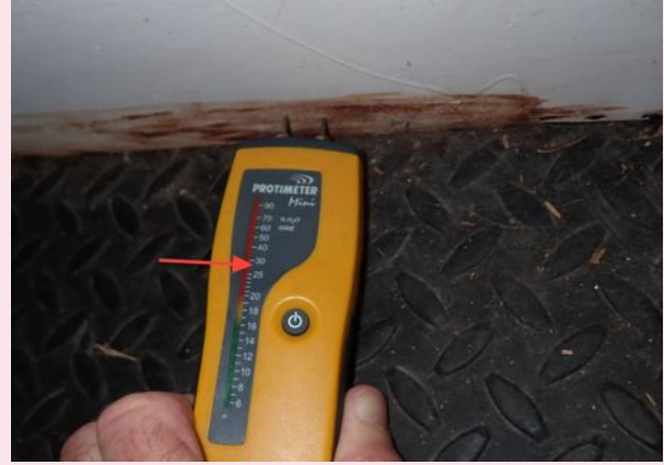
Active Moisture Levels in Stained Trim
