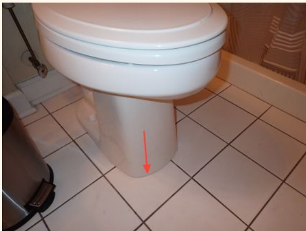
Unsealed Base on Toilet
