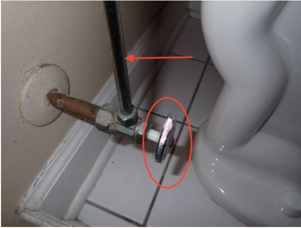
Older Gate Valve and Solid Supply on Toilet
