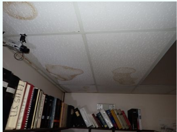
Stained Ceiling Tiles in Office Areas
