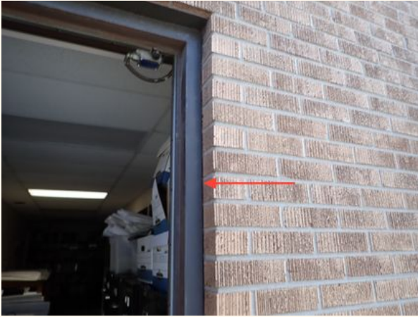
Uncaulked Edges Around Door Openings
