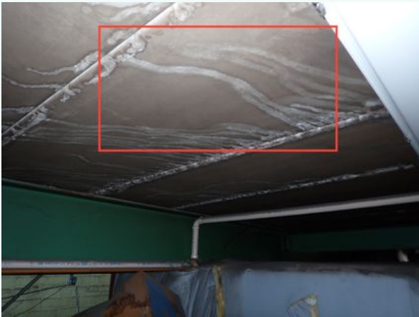
Leakage Stains on Underside of Roof Decking
