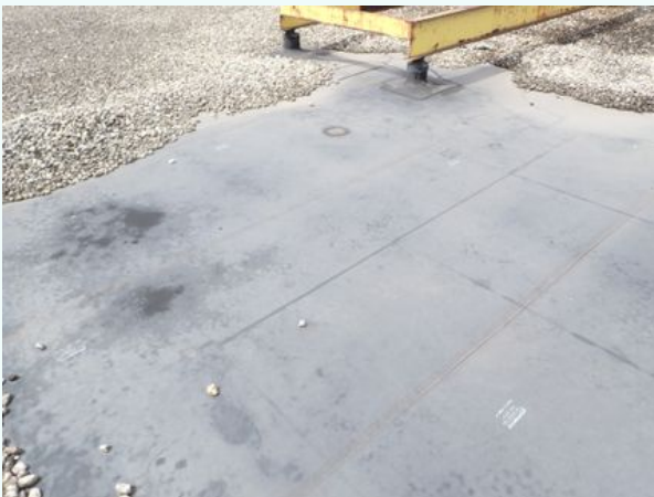
Missing Ballast on Roof
