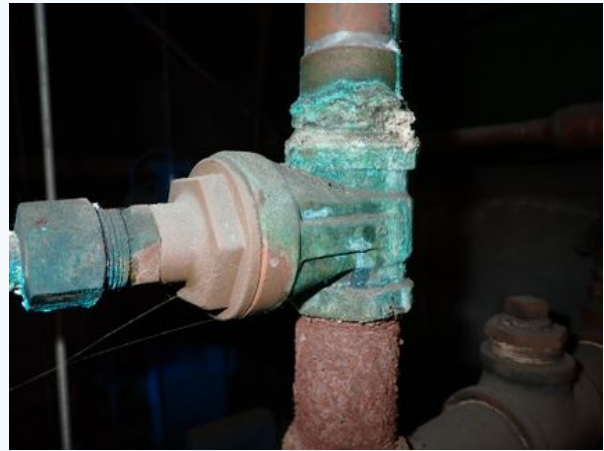
Incipient Leakage on Boiler Piping
