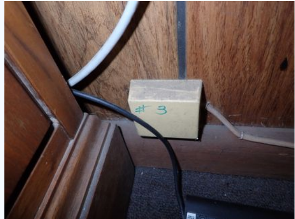
Low Voltage Communication Equipment
