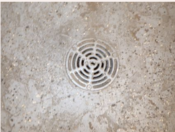
Floor Drains in Rest Rooms
