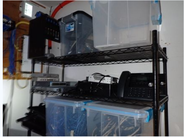
Low Voltage Communication Equipment
