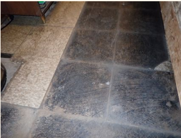
Potential Asbestos Tile and Black Mastic on Floors
