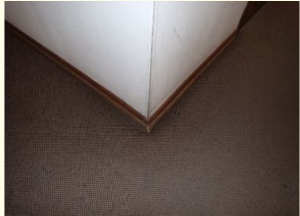
Worn Wall Areas
