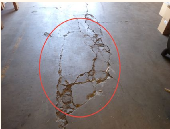
Cracked and Damaged Shop Floor
