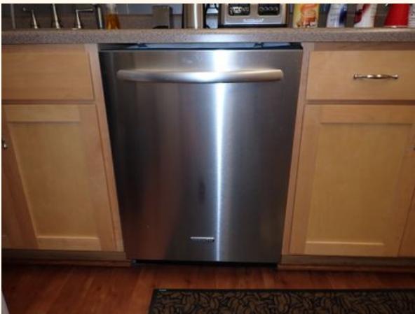
Shut-off Switch Missing on Dishwasher
