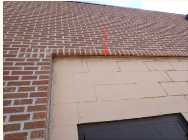
Unpainted and Corroding Lintels
