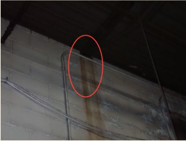
Leakage Stains on Interior
