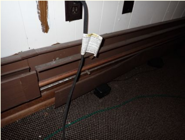
Loose Cover on Baseboard Heater
