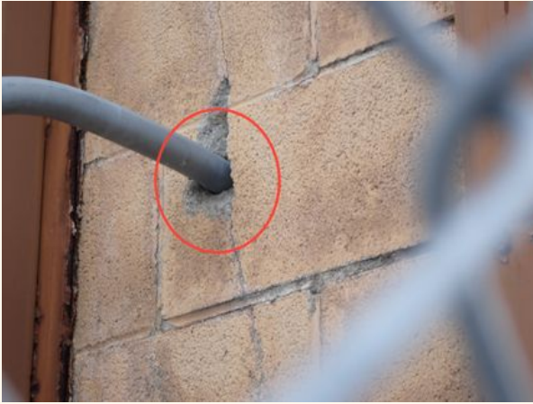
Unsealed Wall Penetrations
