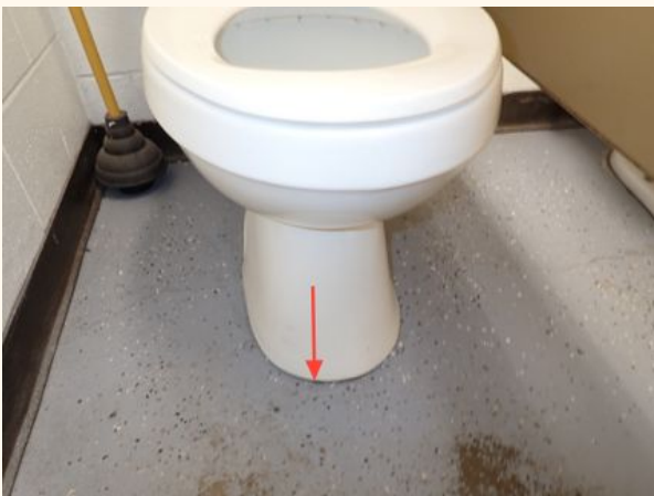
Unsealed Toilet Base
