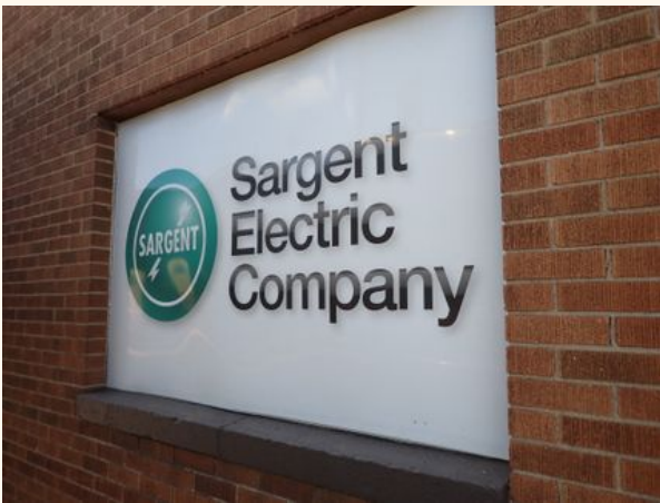
Sign Covers Broken Blocks
