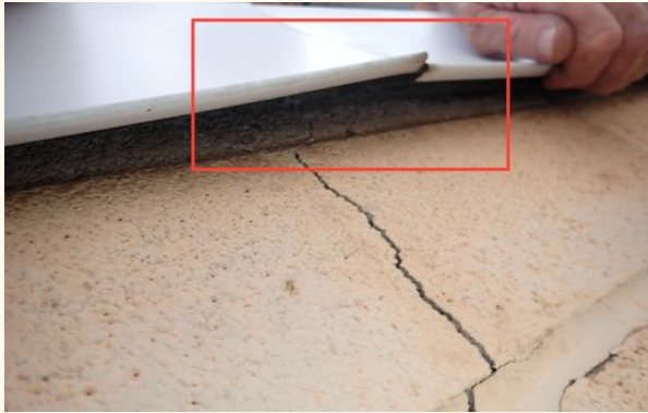
No Splice on Cap Joint
