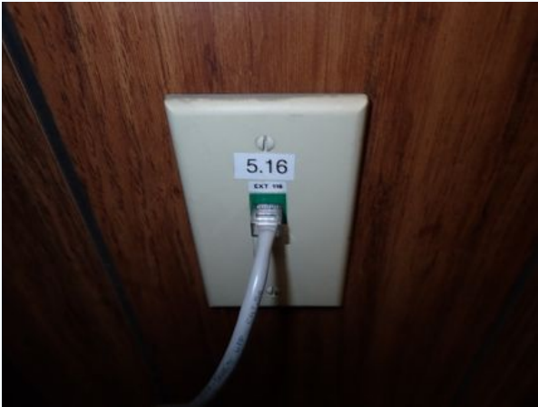
Low Voltage Communication Equipment
