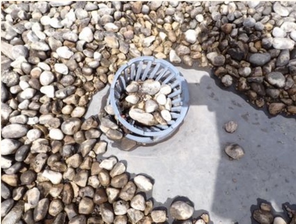
Blocked Roof Drain
