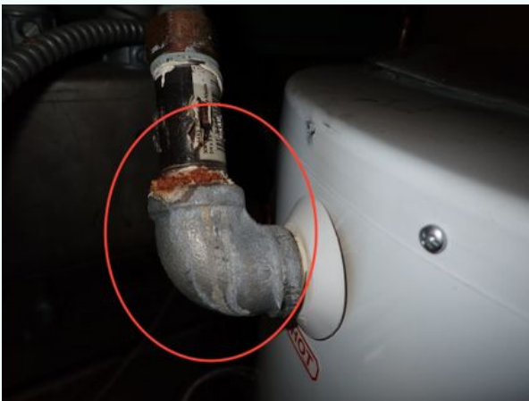
Incipient Leakage on Water Heater Piping
