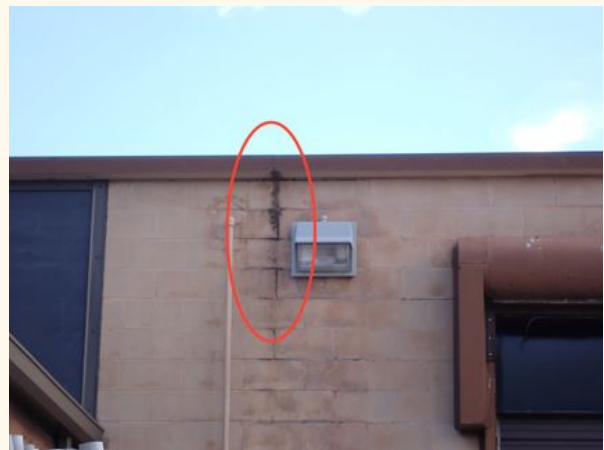
Leaking Gutter Joints
