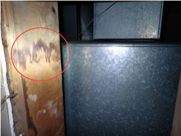
Moisture Stains on Framing Below Ductwork
