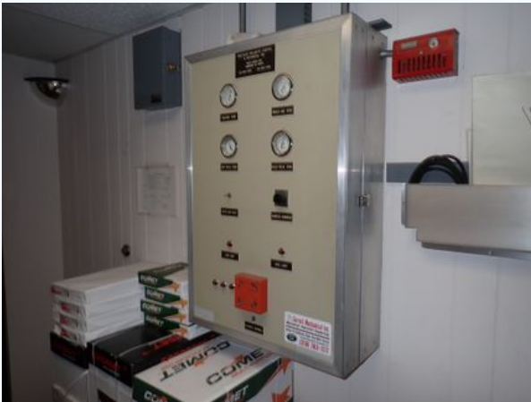
Pneumatic Control System
