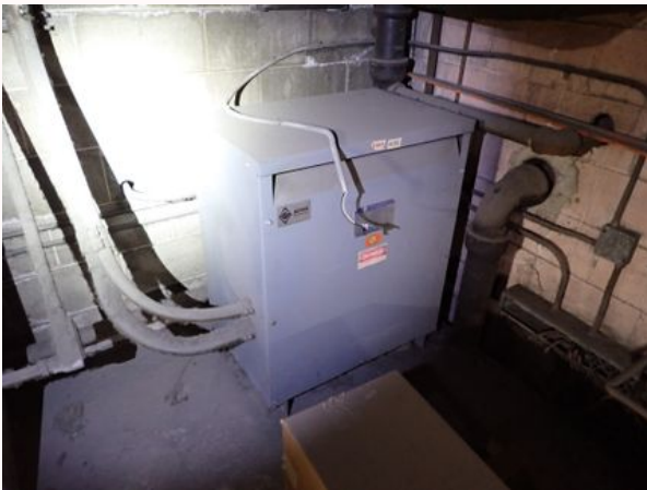
Live Wring By Transformer
