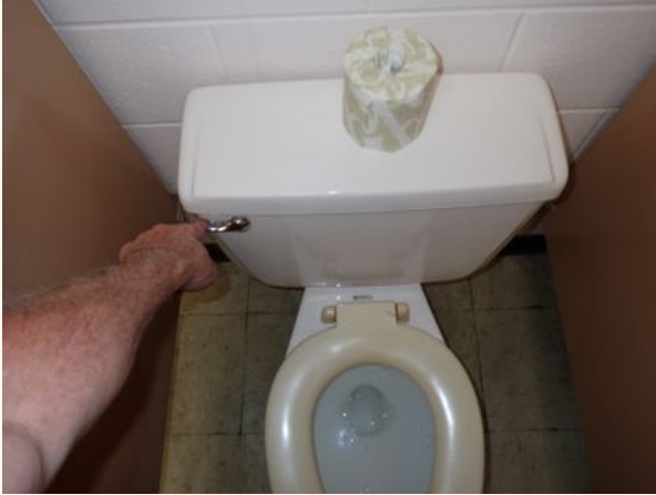
Non-flushing Toilet in Men's Room
