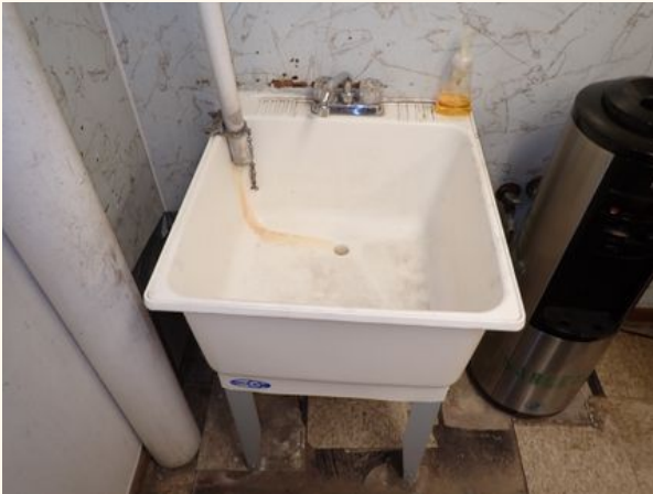
Loose Utility Sink
