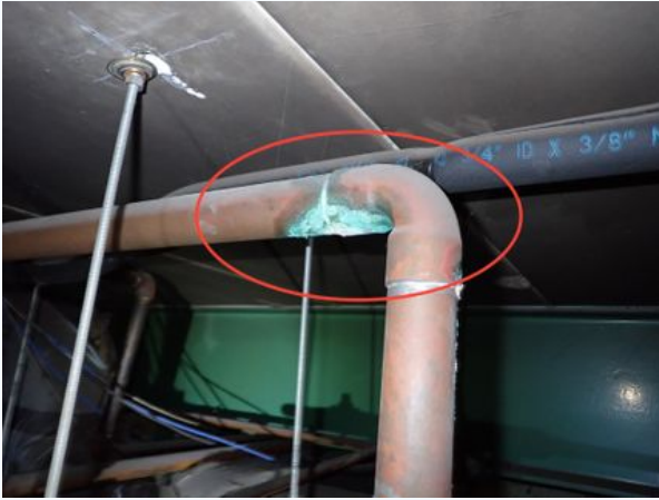
Incipient Leakage on Boiler Piping
