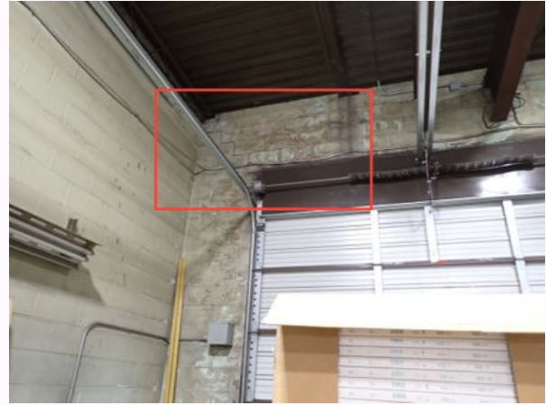
Significant Cracking and Efflorescence Near Garage Door
