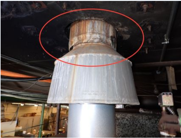
Corrosion on Vent Piping
