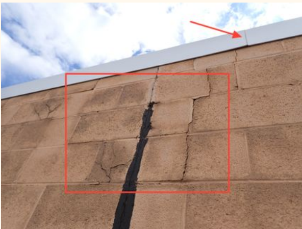
Cracked and Damaged Masonry Below Cap Joint
