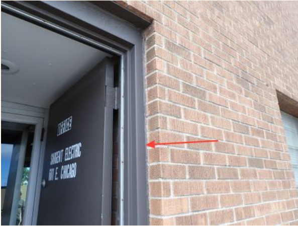
Cracked and Open Caulk Joints
