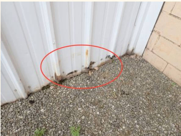
Corroded Holes in Exterior Metal Siding
