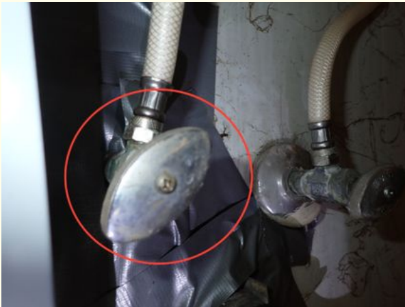
Gate Shut-off Valves
