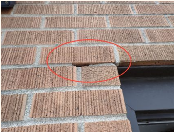
Cracked and Open Mortar Joint by Lintel
