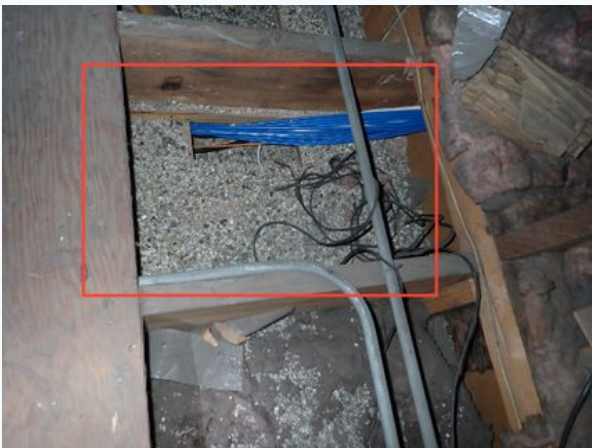
Vermiculite in Attic Area
