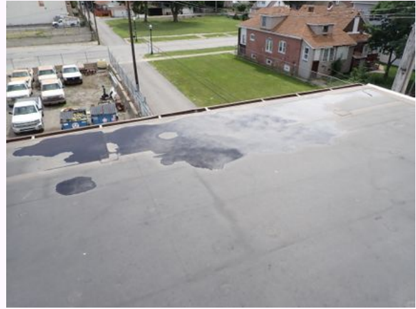
Ponding on Upper Roof
