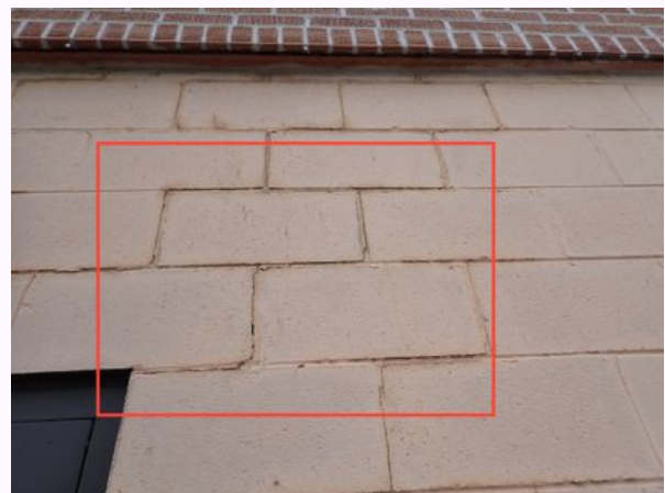
Significant Cracking by Garage Door Lintel
