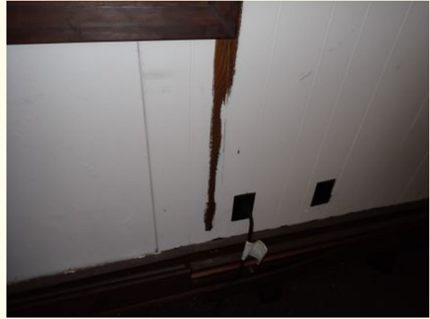
Missing Paint on Wall Finishes
