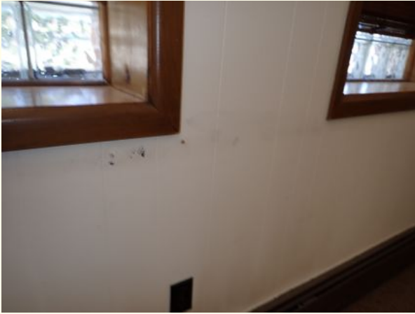
Damaged Wall Finishes
