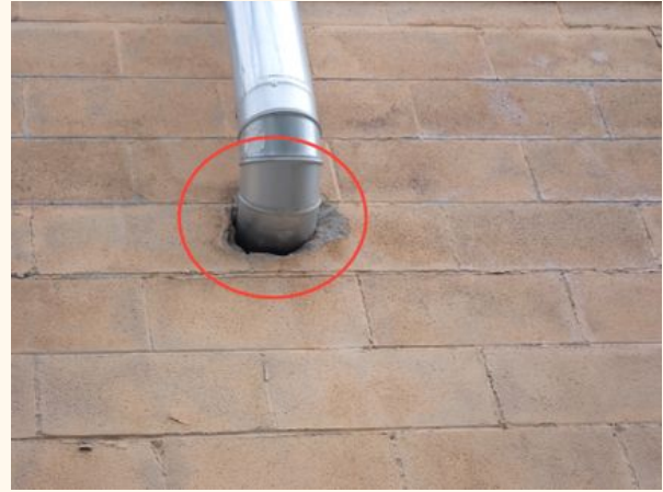
Unsealed Wall Penetrations
