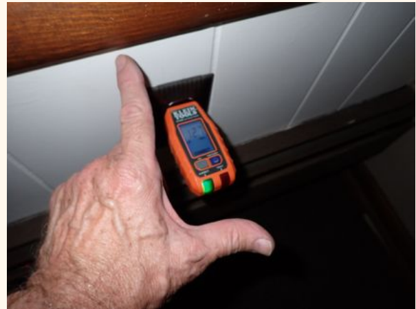
Loose Receptacle in Office
