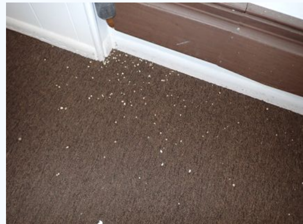
Loose Insulation Fragments in Office
