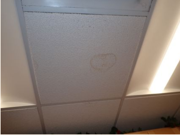
Stains on Ceiling Tiles in Kitchen
