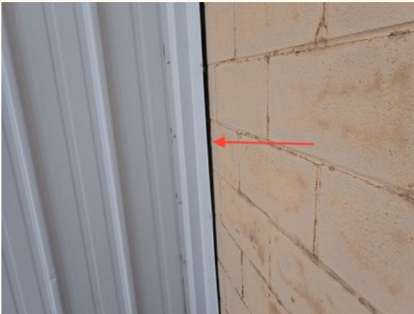
Unsealed Gap by Metal Siding
