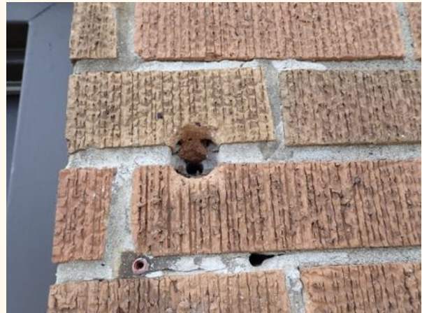
Open Holes in Walls
