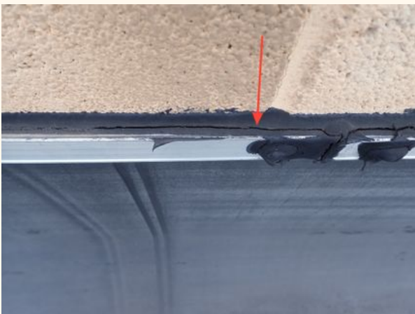
Old Cracked Sealant
