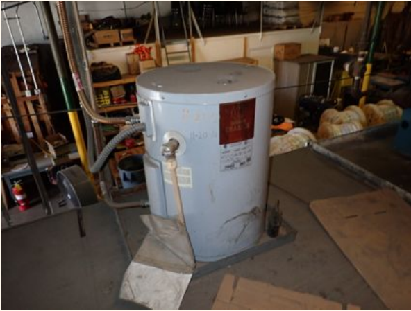
No Shut-off on Water Heater
