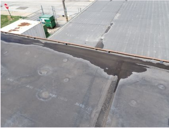
Ponding on Bare Roof Areas
