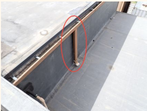
Loose Downspout on Roof
