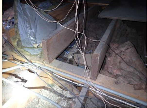
A Variety of Insulation Including Vermiculite
