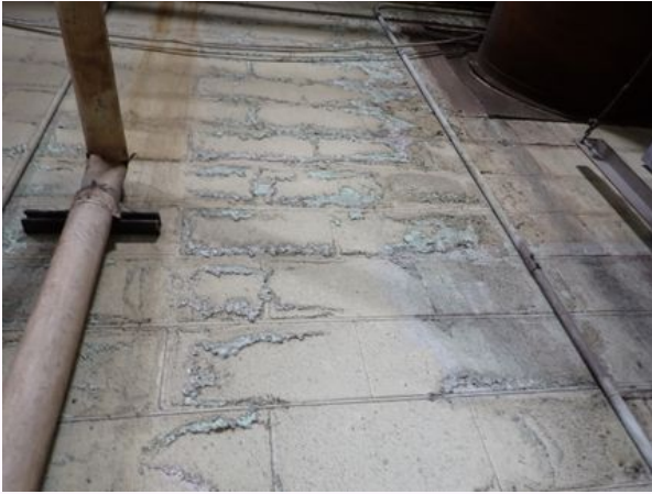
Efflorescence on Interior of Building
