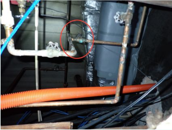
Leakage Stains on Piping
