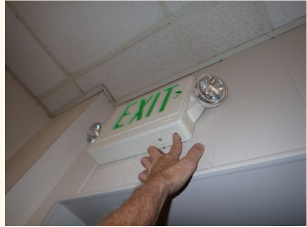
Non-functional Emergency Lighting
