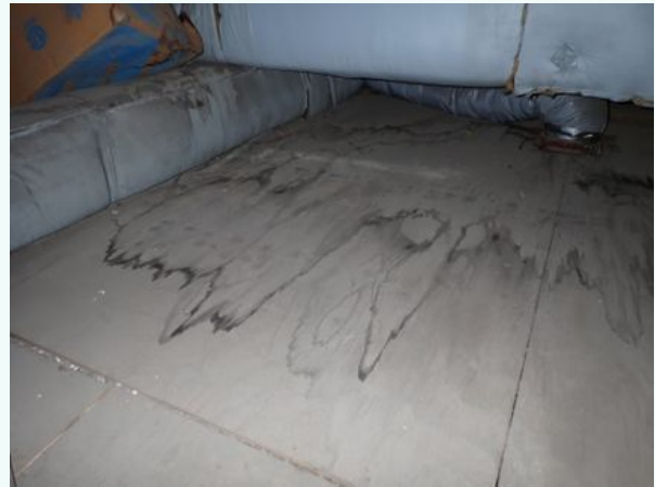
Stains on Mezzanine Flooring
