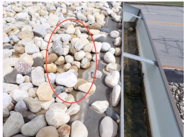
Non-draining Areas Near Gutters
