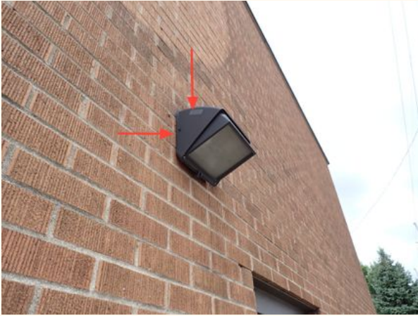
Caulking Needed Around Exterior Light Fixtures
