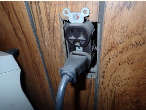
Uncovered Receptacle in Office
