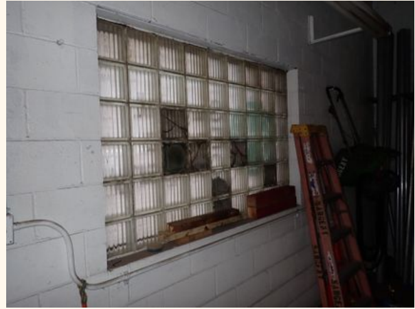
Broken Block Windows in Shop Area
