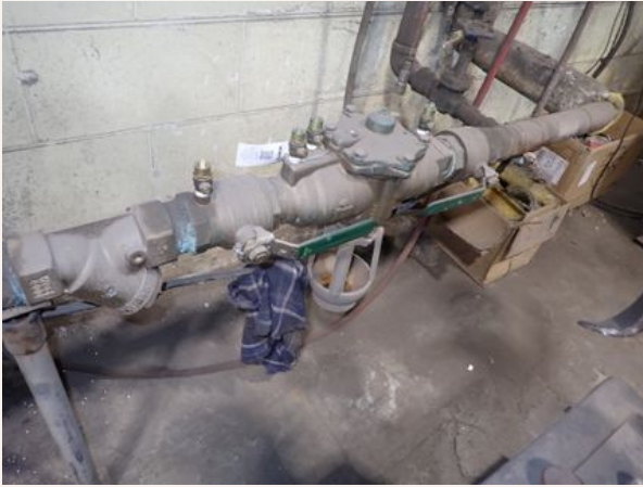
Backflow Prevention Device
