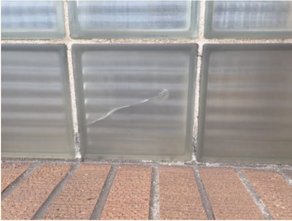
Broken Glass Block - BB Hole
