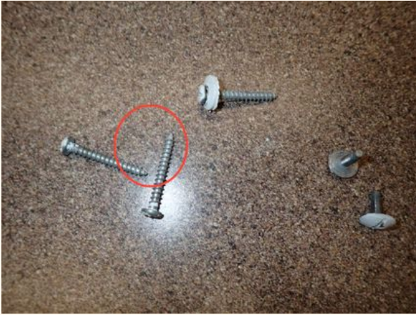
Pointed Tipped Screws Securing Electric Service Panel
