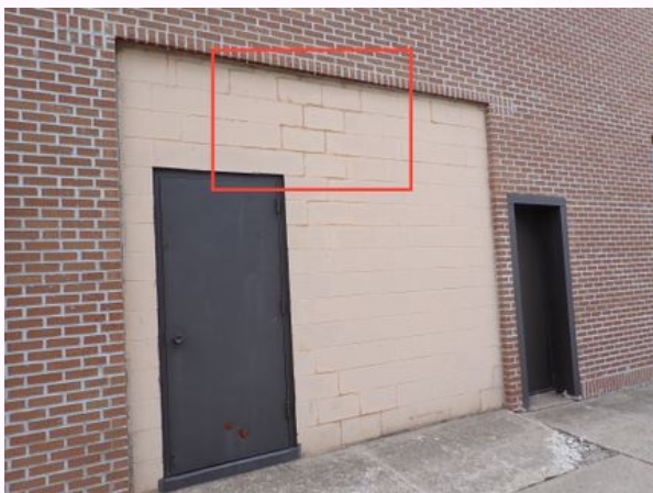
Cracks in Block Wall Areas
