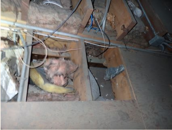
Areas of Minimal and Missing Insulation
