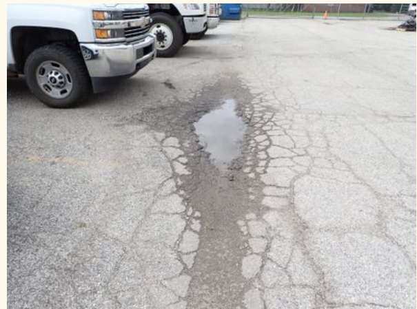
Deteriorated Pavement in Yard Area
