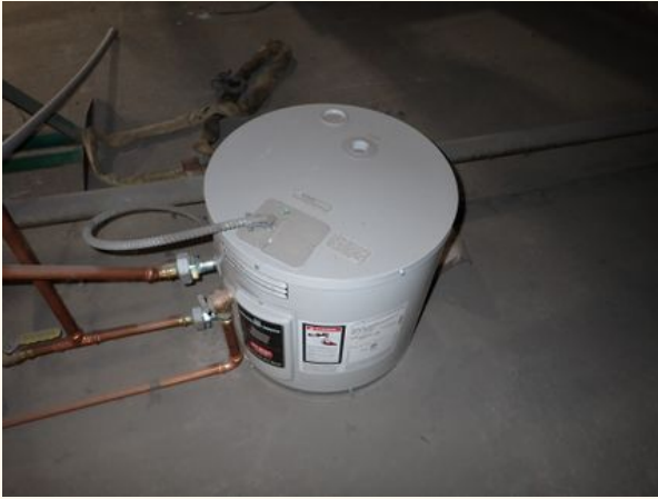
Drip Pan Missing on Water Heater
