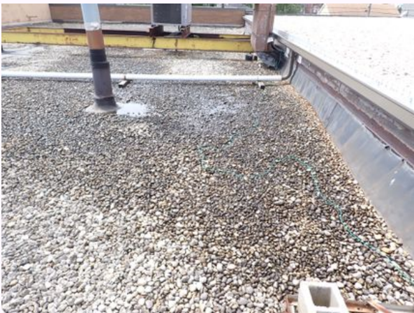
Large Area of Standing Water
