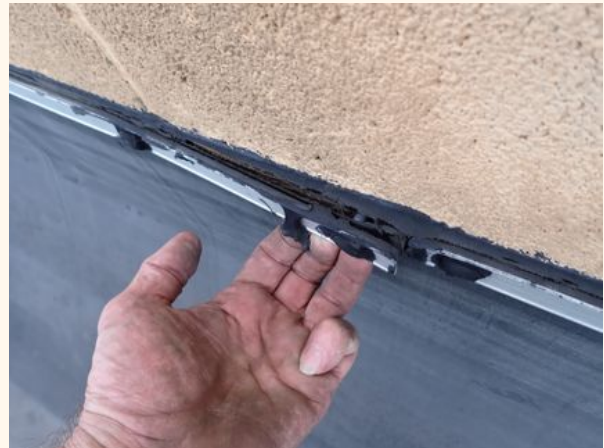
Loose and Unsealed Flashing
