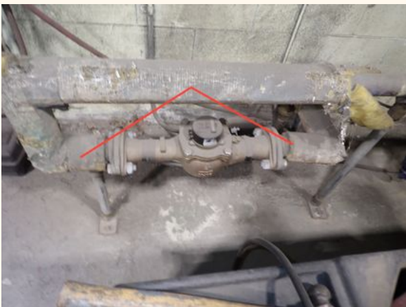
Jumper Missing Across Meter
