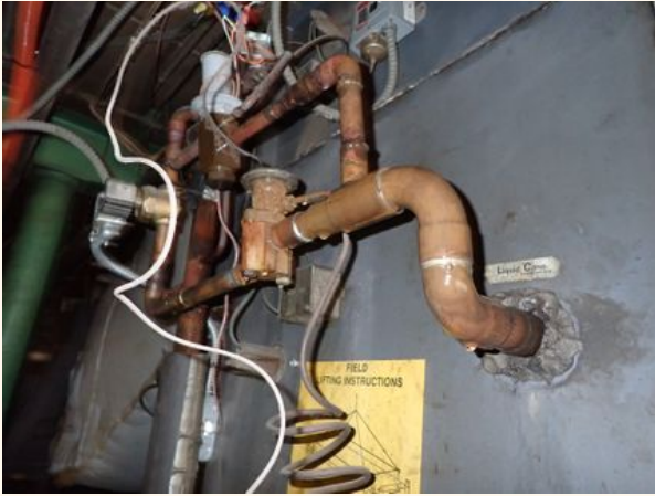
Leakage on A/C Lines
