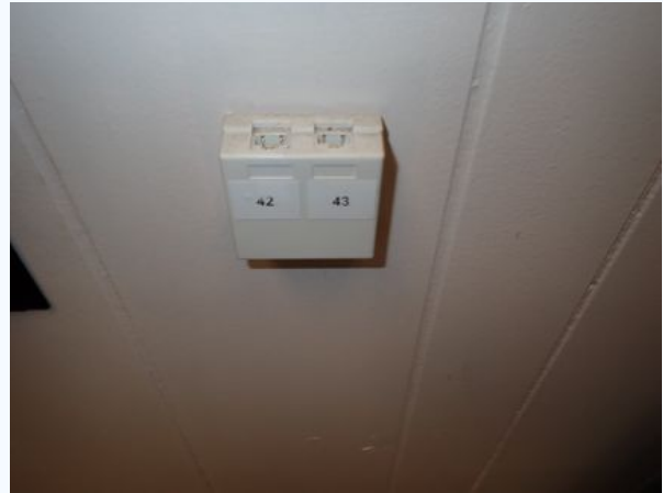
Low Voltage Communication Equipment
