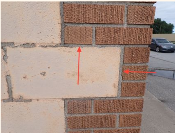
Cracks Noted in Dissimilar Materials Joints
