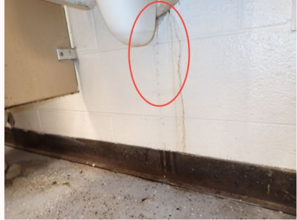
Leakage From Urinal
