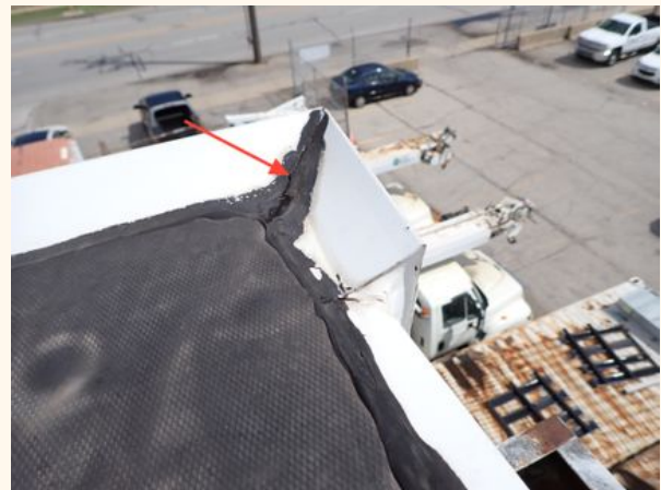
Cracked and Open Corner Joints in Capping
