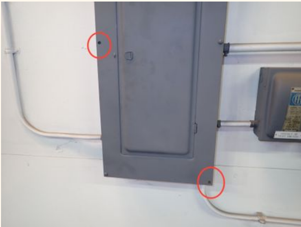
Missing Screws in Panel Cover
