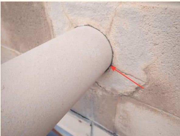
Unsealed Wall Penetrations
