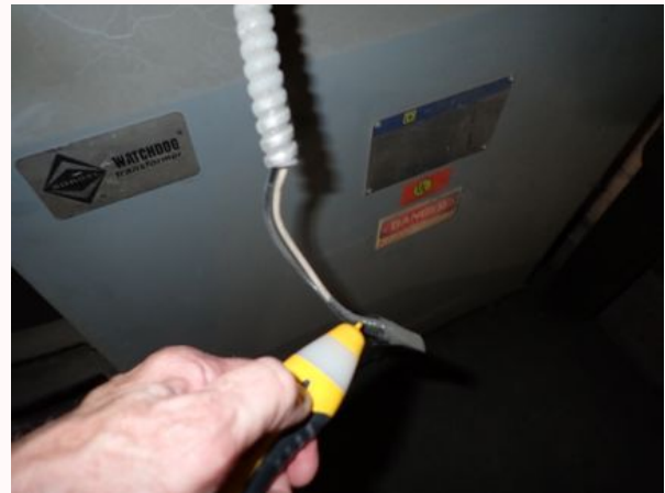
Taped Live Wires
