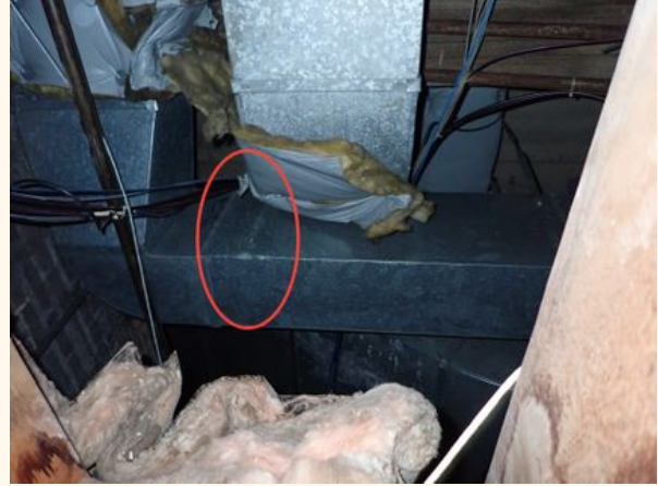
Missing Insulation and Moisture Staining on Ductwork
