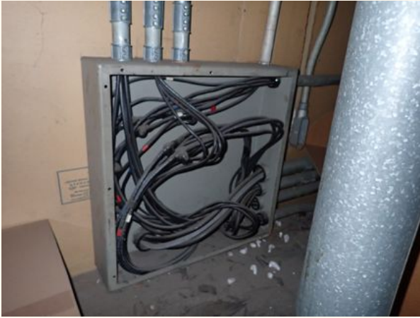
Exposed Wiring in Mezzanine
