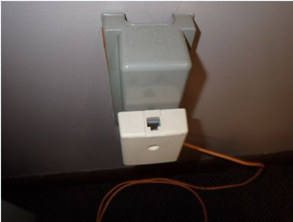
Low Voltage Communication Equipment
