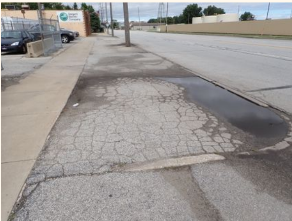
Cracked and Deteriorated Parkway Areas
