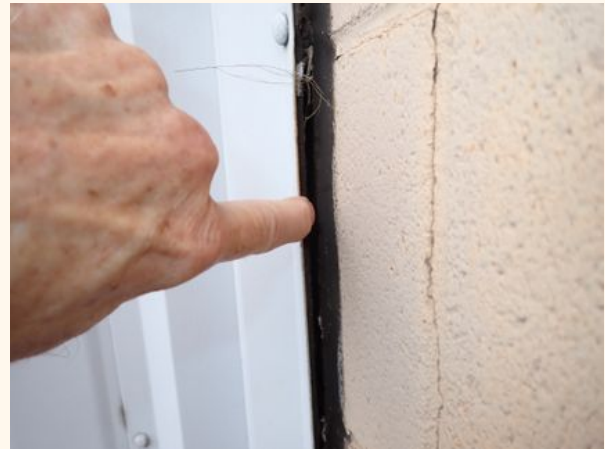
Close-up of Large Open Gap
