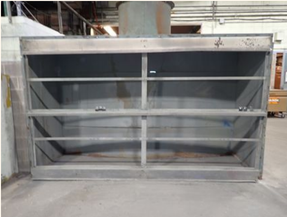
Massive Interior Vent Fan
