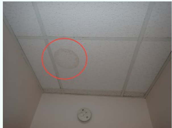
Stain on Ceiling Tile in Hallway
