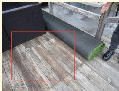
Carpeting Trapping Moisture and Damaging Deck
