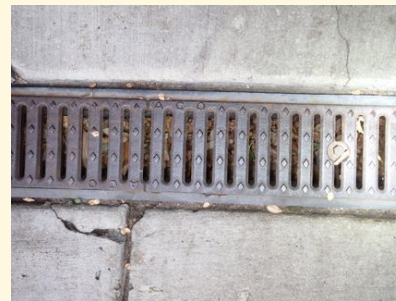
Trench Drain Clogged with Leaves
