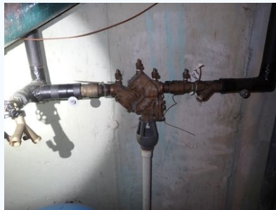
RPZ (if for sprinkler) Requires Annual Servicing
