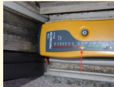
Elevated Moisture Levels in Doorframe
