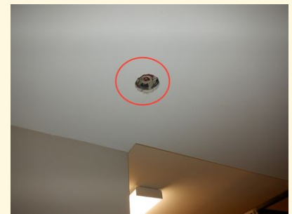
Open Junction Box in Basement Ceiling
