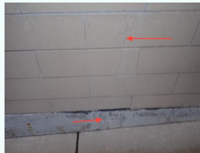
Cracking in Masonry by Crack
