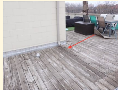
Damaged Noted by Downspout Discharge
