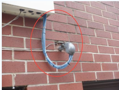
Low Voltage Communication Equipment
