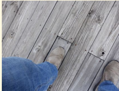
Protruding and Weathered Deck Boards
