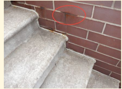
Corrosion on Stairwell Walls
