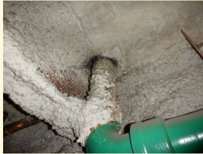
Unsealed Pipe Penetrations
