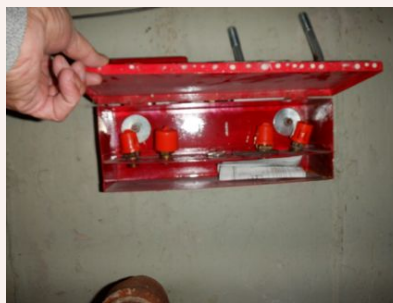
Sprinkler Equipment Box in Mechanical Room
