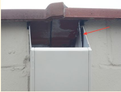
Unsealed Roof Edge on Side of Scupper
