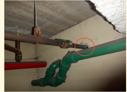
Unsealed Pipe Penetrations
