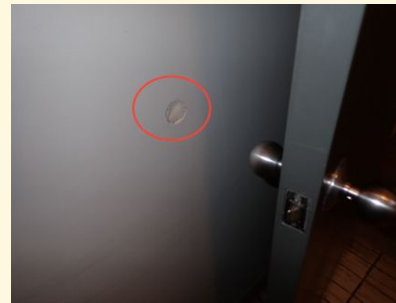
Damaged Walls by Doors
