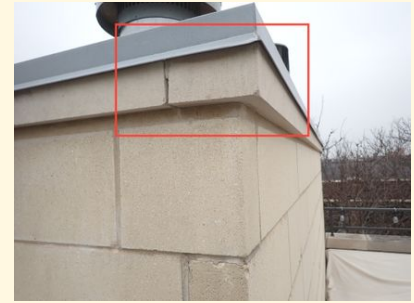
Cracked and Damaged Masonry Below Metal Caps
