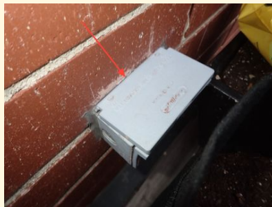
Unsealed Wall Penetrations
