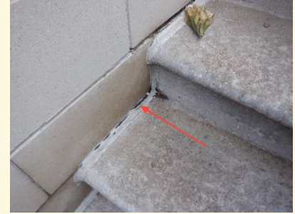
Cracked and Deteriorated Caulk on Edges of Stairs
