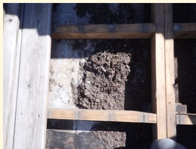
Dirt and Debris Beneath Deck
