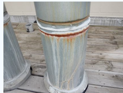
Close-up of Corrosion on Vent Pipe
