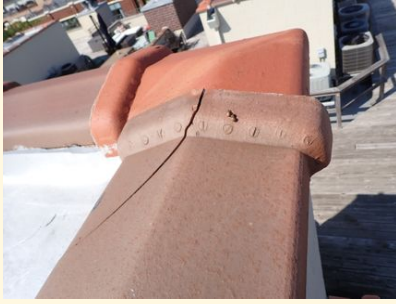
Damaged Clay Tile Cap
