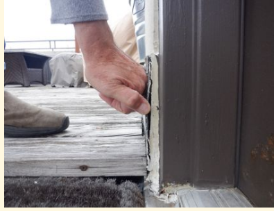
Unsealed Edges on Vertical Roof Edges
