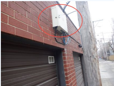
Low Voltage Communication Equipment
