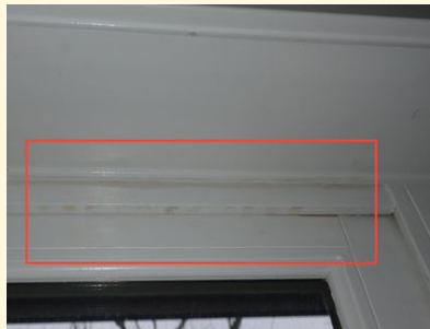
Moisture Stains Noted in Trim Above Sliding Door in Upper Level Unit
