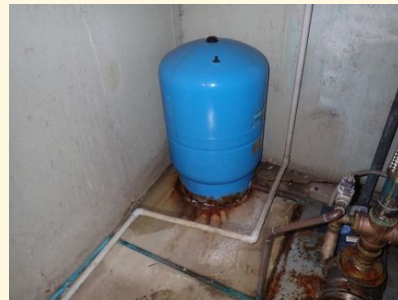
Small and Waterlogged Pressure Tank
