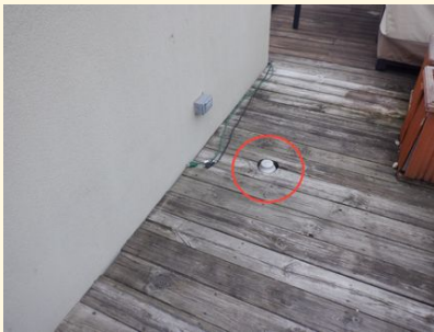
Rooftop Breather Vents
