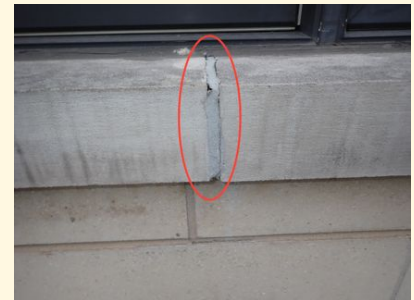
Gaps and Openings in Caulk Smear
