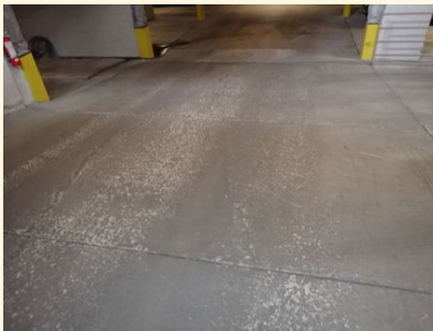
Spalled Driveway Surface
