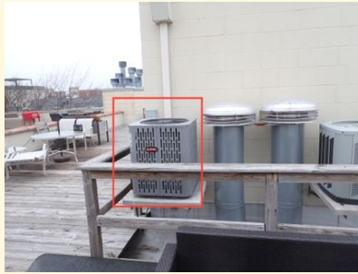
New A/C Condensers Noted in These Locations
