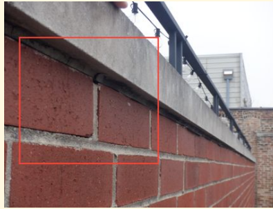
Cracked Mortar Joints Below Cap
