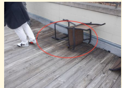
Sagging and Unstable Deck Area
