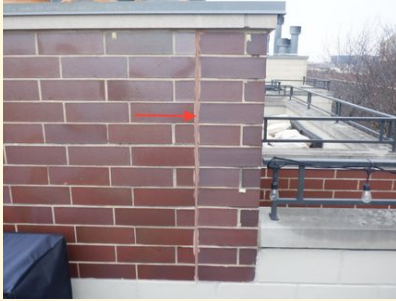
Failing Caulk Joints Noted
