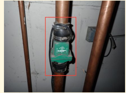
Non-reinforced Coupling on Sump Discharge in Garage
