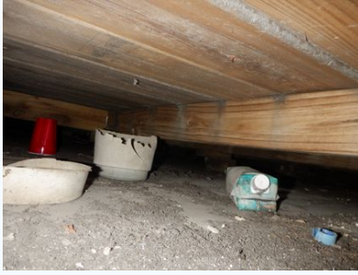
Dirt and Debris Noted Beneath Rooftop Decks
