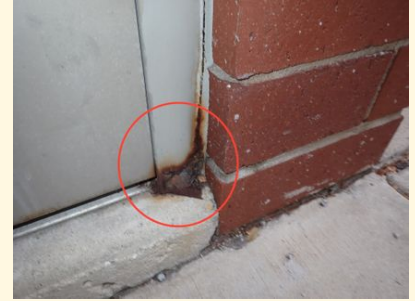
Corrosion on Metal Entry Doors
