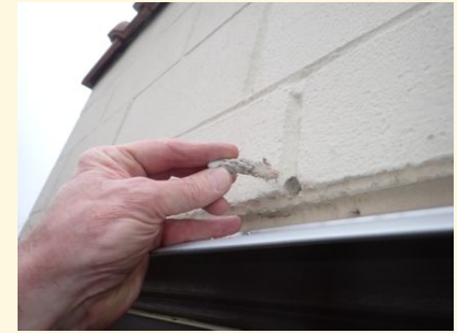
Loose and Improper Weep Ropes
