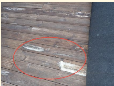
Wood Rot on Deck Areas Below Carpet
