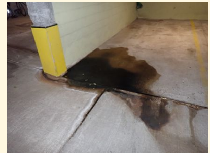
Standing Water in Garage
