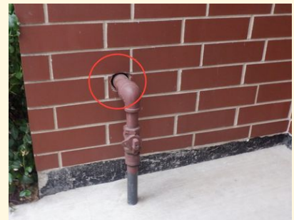
Unsealed Wall Penetrations
