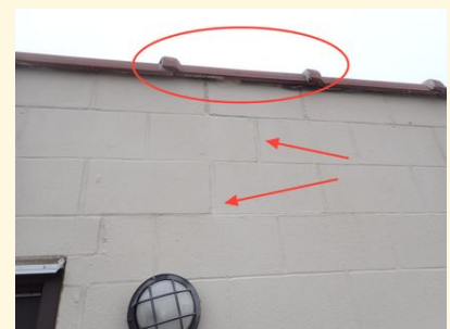
Cracks in Masonry Below Cracked and Open Cap Joints
