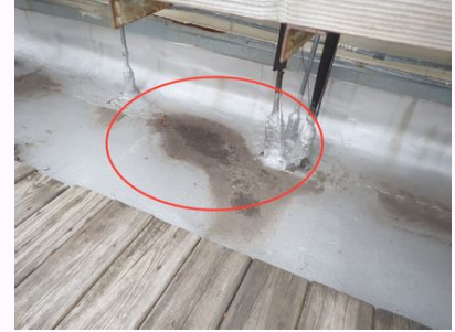
Ponding Areas on Roof
