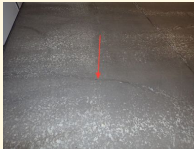
Cracks in Driveway
