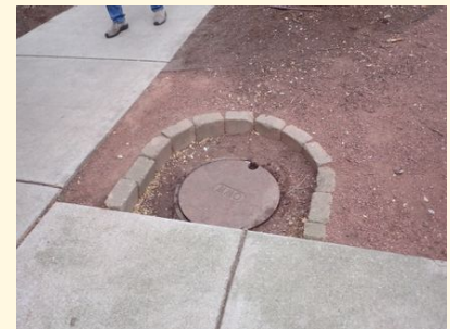
Below Grade Shut-off
