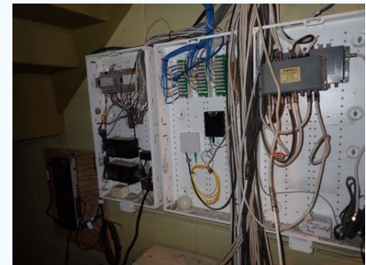
Low Voltage Communication Equipment
