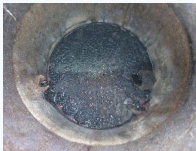
Manhole Full of Sludge
