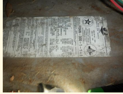
Data Plate on Heaters
