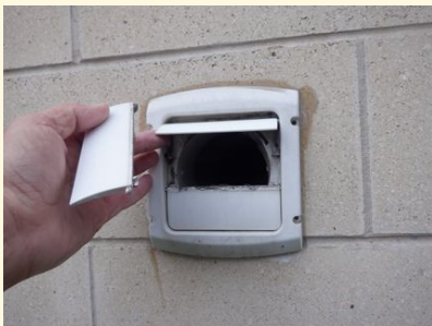
Broken Vent Damper
