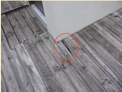
Deteriorated Deck Board
