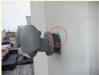
Unsealed Junction Box on Upper Deck Light
