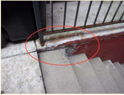
Deteriorated Concrete on Wall
