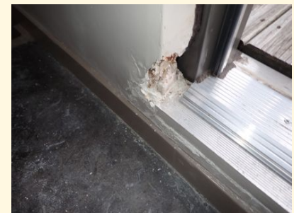
Damaged Wall Areas by Rooftop Access Doors
