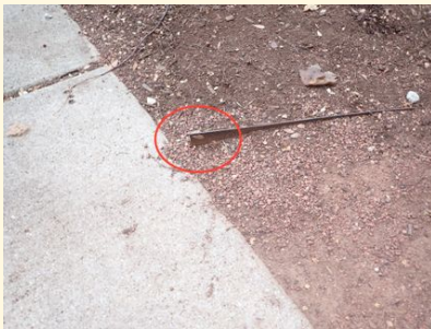
Exposed Metal Edging
