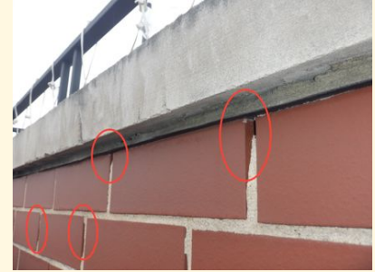
Numerous Poorly Formed Joints
