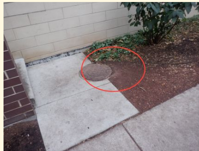
Areas of Ponding Water
