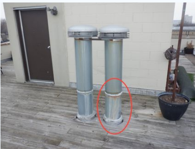
Heavy Corrosion on Vent Pipe
