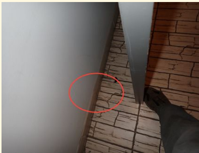
Doorstops Missing on Some Doors
