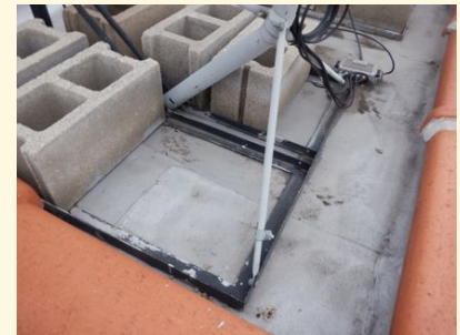
Metal Frames on Roofs
