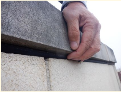
Thin Membrane Flashing and Open Gaps on Edges of Caps
