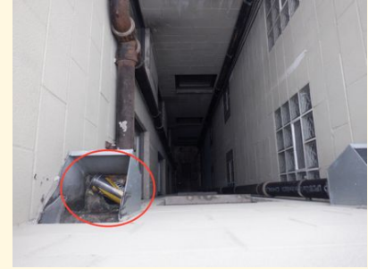
Debris Noted in Scupper
