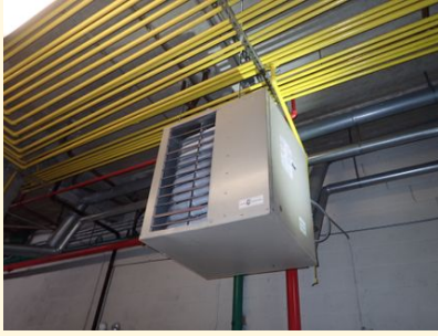
Space Heaters in Garage
