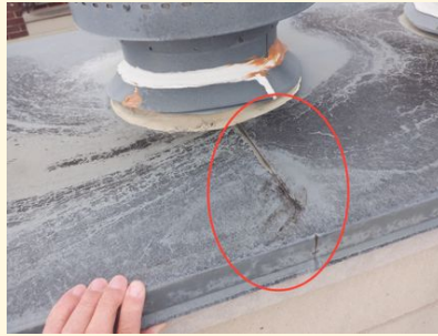
Open Seam Joints Prone to Leakage
