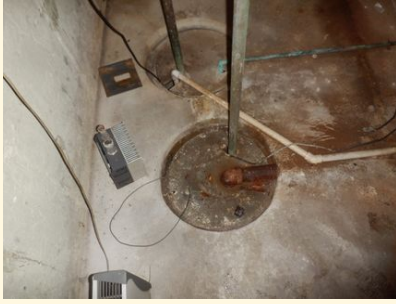
Unsealed Sump Pits
