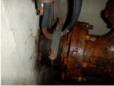
Loose and Improperly Clamped Bonding Wire
