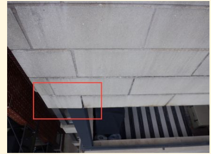
Displaced Blocks by Steel Framing
