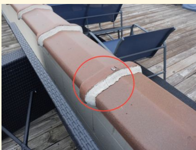
Cracked and Open Joints on Clay Tile Cap
