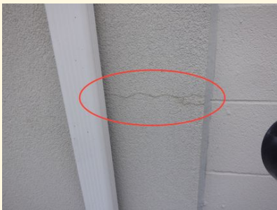
Cracks in EIFS
