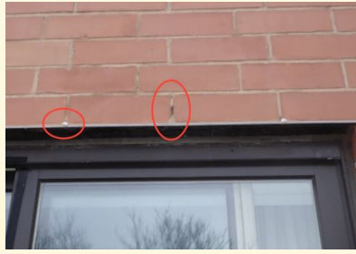
Blocked Weep Hole and Potentially Improper Weep Ropes
