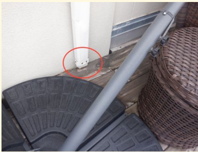
Downspout Discharging onto Roof Deck
