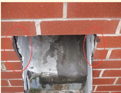
Open Gaps Between Scuppers and Masonry Openings
