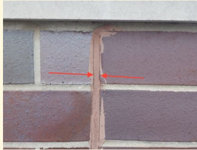
Cracks Noted on Sides of Caulk Joint
