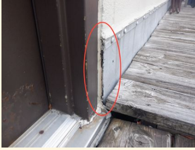
Missing Termination Bar Flashing
