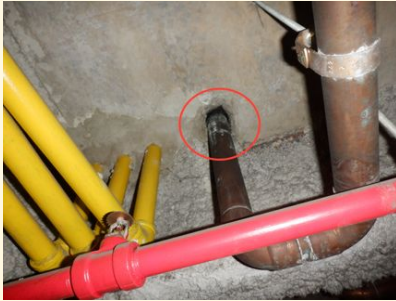
Unsealed Pipe Penetrations
