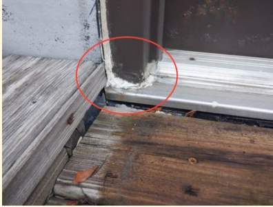
Sloppy Caulk by Doorframes
