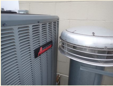
Vent Pipe Discharging Next to A/C condensers
