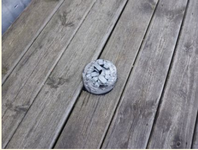
Flush and Blocked Vent Pipes
