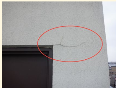
Cracks in EIFS
