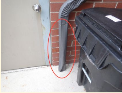
Damaged Downspout Surrounded by Sidewalk
