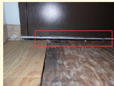
Daylight Observed Beneath Entry Doors
