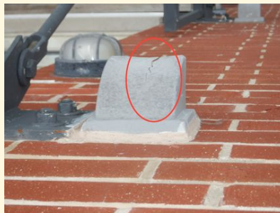
Cracked Vent Damper
