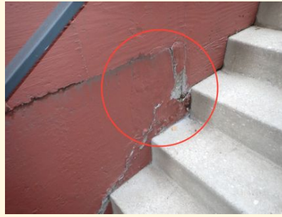
Deteriorated Concrete on Retaining Wall
