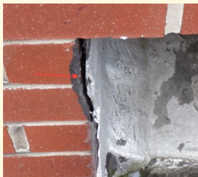
Close-up of Large Open Gaps on Scuppers
