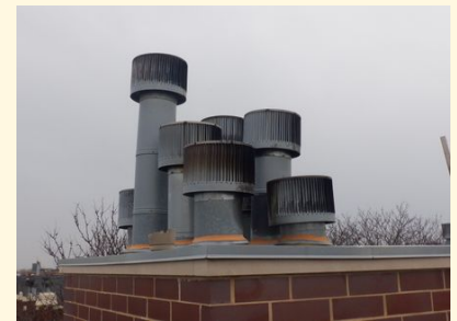
Inadequate Spacing of Fireplace Vents
