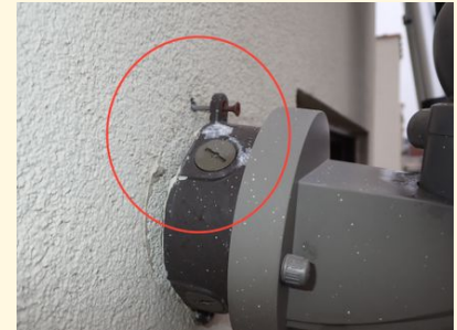
Loose Light on Rooftop Deck
