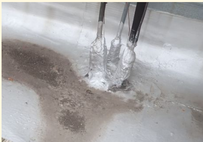
Multiple Layers of Sealant Materials on Rooftop Penetrations
