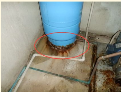
Heavily Corroded Expansion Tank
