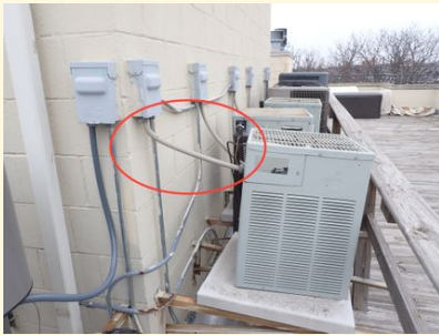
Power Feed Under Tension
