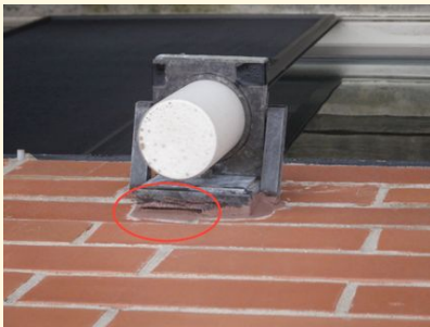
Unsealed Edge on Balcony Light
