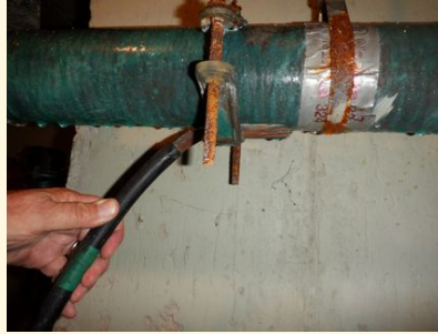
Loose and Improperly Clamped Bonding Wire
