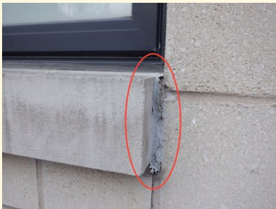
Caulk Smeared Joint on Stone Sill
