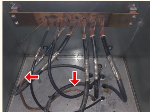
Bare Conductor Connected to Bus
