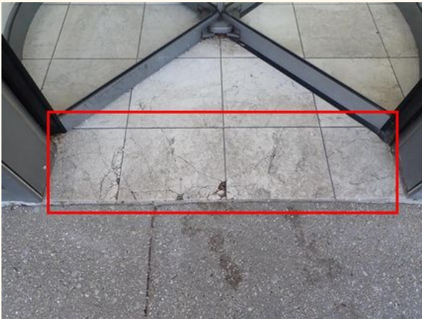
Cracked Tile by Front Entrance
