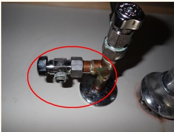
Active Leakage From Abandoned Valve
