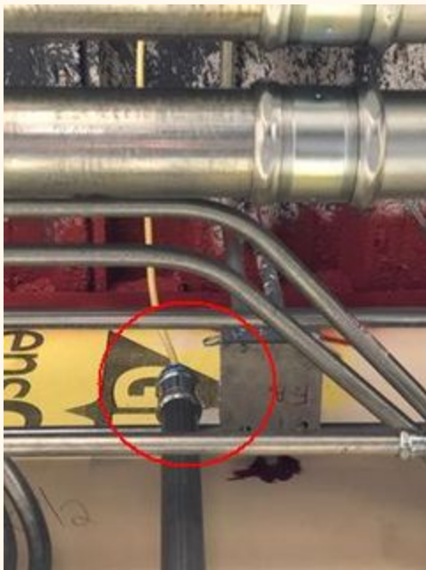
Open Raceway in Unfinished Area
