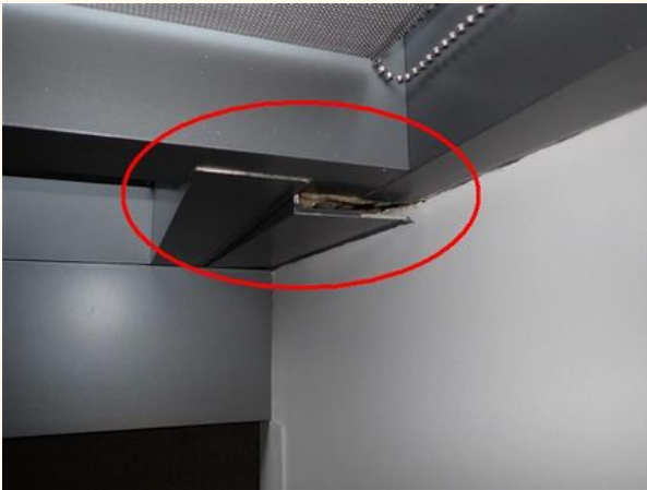
Loose Window Trim
