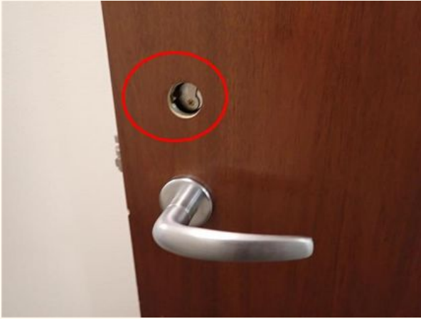
Missing Hardware on Doors
