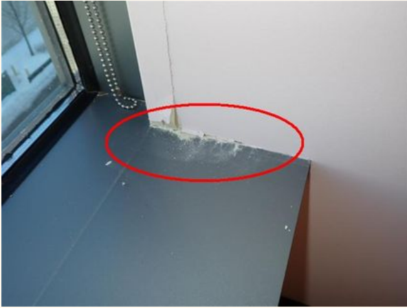
Potential Moisture Related Damage Noted on Numerous Wall Surfaces
