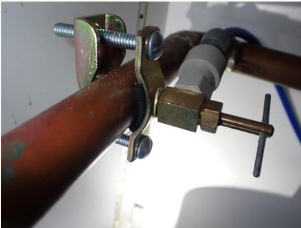
Unreliable Saddle Valve for Filter Water Supply
