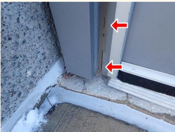
Gaps in Caulking Noted Around Windows
