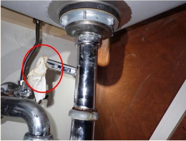
Leakage Noted From Improperly Abandoned Dishwasher Drain
