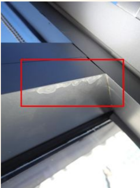
Moisture Stains on Interior Corners
