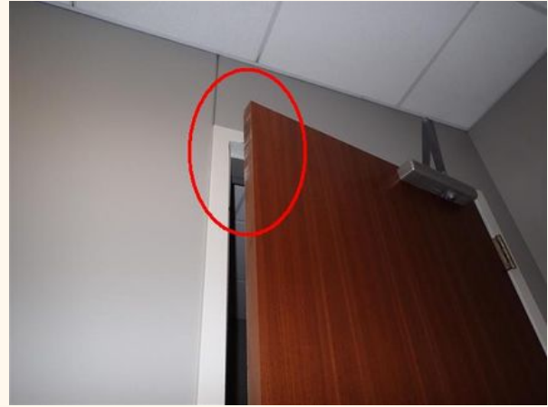
Doors Rubbing on Doorframes
