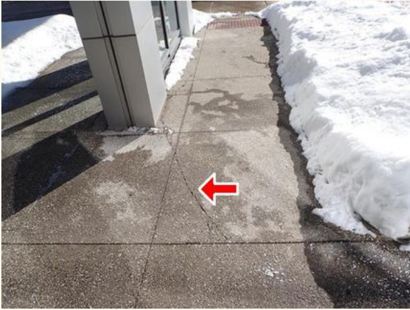
Cracks Noted in Exterior Walks
