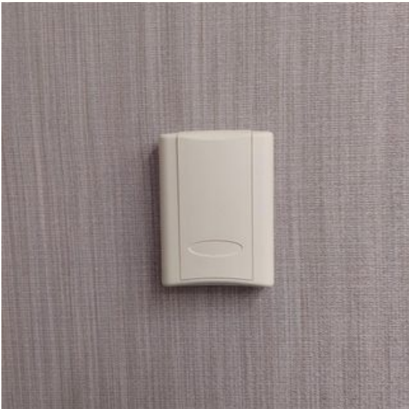
Typical Wall Mounted CO 2 Monitor
