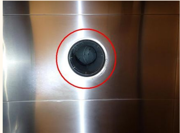
Vent Pipe Open to the Exterior - Cold Air Noted
