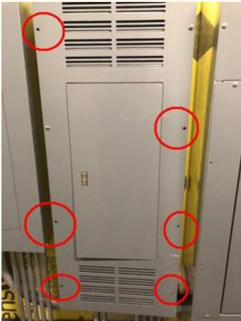
Missing Screws on Panel 2-rr-1
