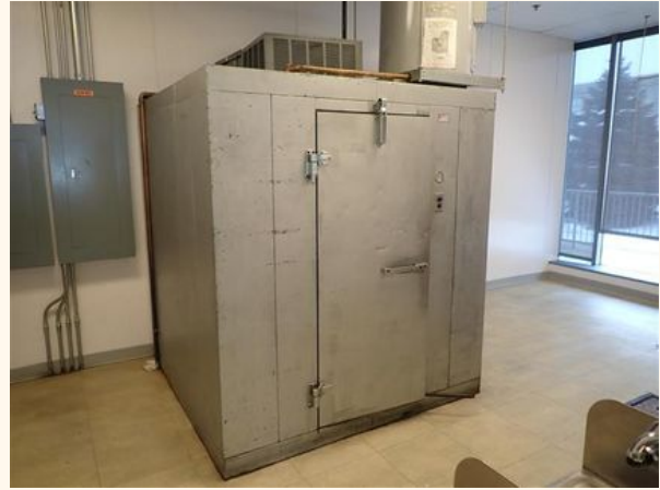
Large Refrigerator Unit
