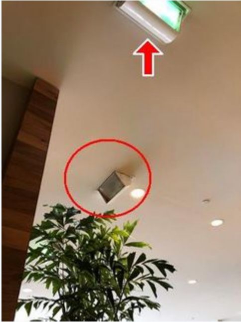
Flickering Exit Signs and Non-functional Halogen Fixtures
