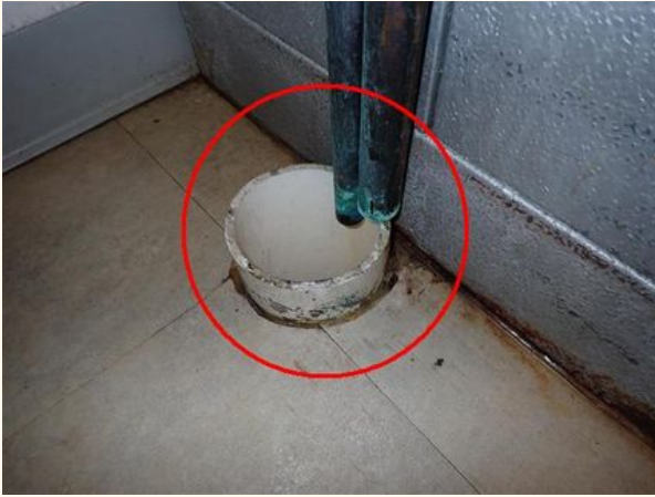
Fridge Drain Line Discharging Outside of Floor Drain
