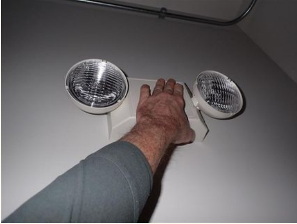
Non-functional Emergency Lights Noted
