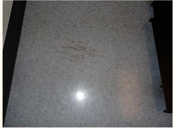
Damaged Floor Finishes
