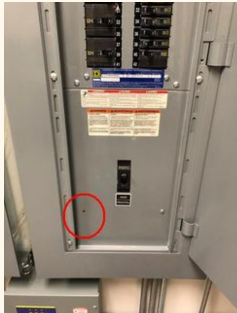
Missing Screws on Panel Cover in Electrical Room 110
