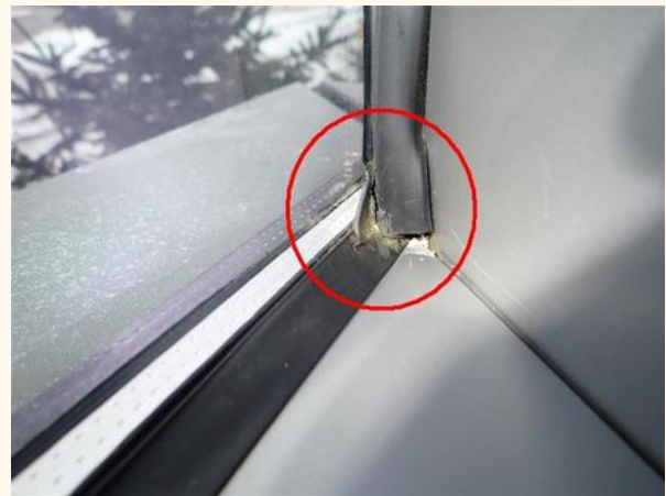
Potentially Improper Corner Seal - Staining or Dirt in Corner?
