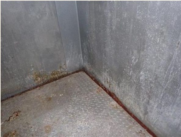
Corrosion Noted on Interior of Fridge
