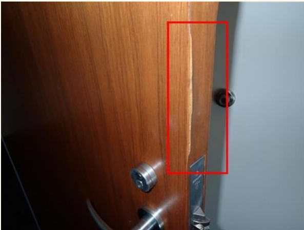
Peeling Veneer on Several Doors Noted
