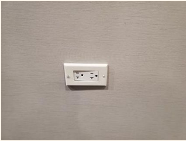
Loose Covers on Receptacles
