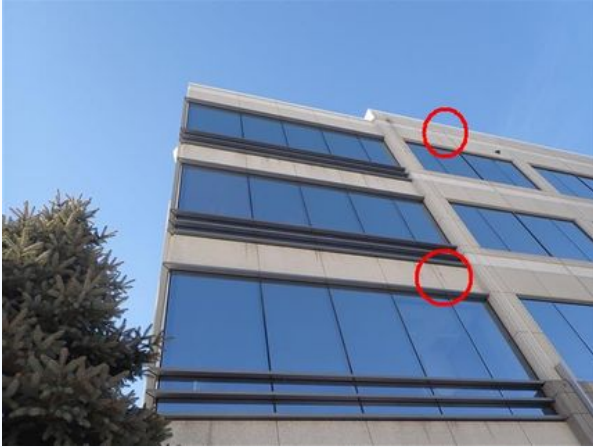
Corrosion Noted on Pre-cast Panels
