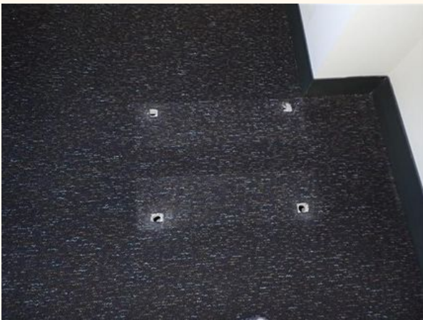
Holes in Floor
