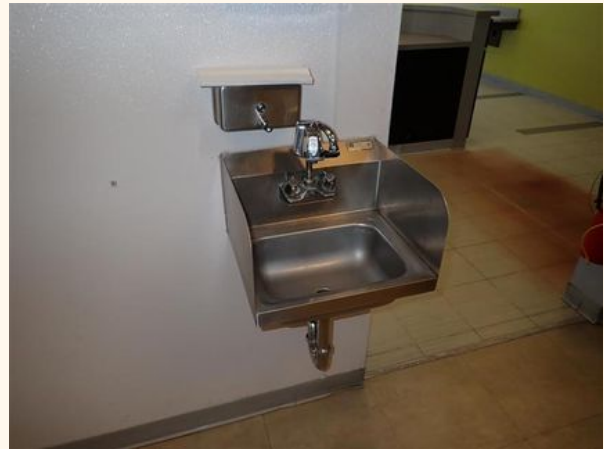
Non-functional Hand Washing Sinks
