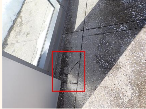
Cracked Walks Noted
