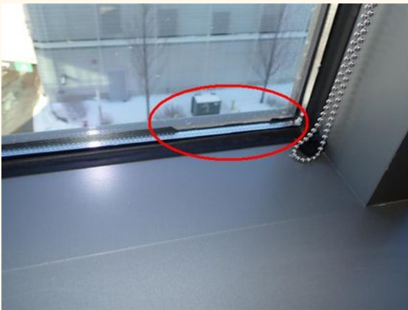
Irregular Sealant Installation
