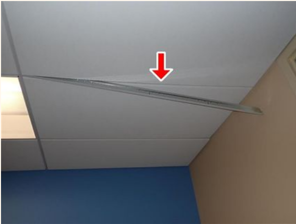
Loose Ceiling Tile Grid Members
