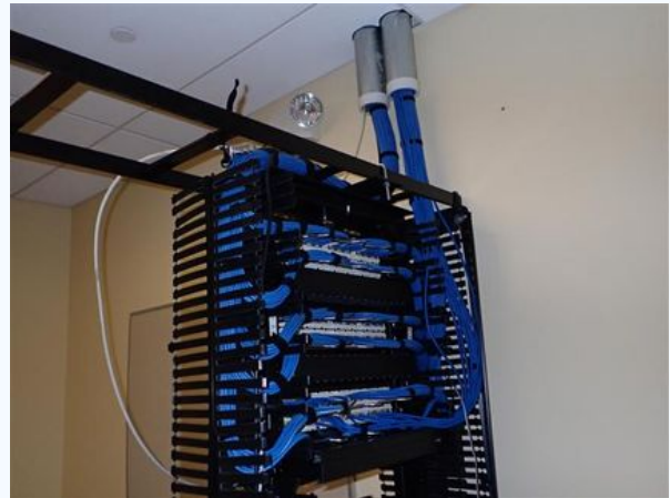
Abandoned Wiring and Racks
