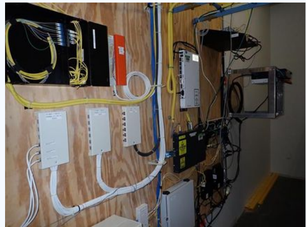
Low Voltage Communication Equipment
