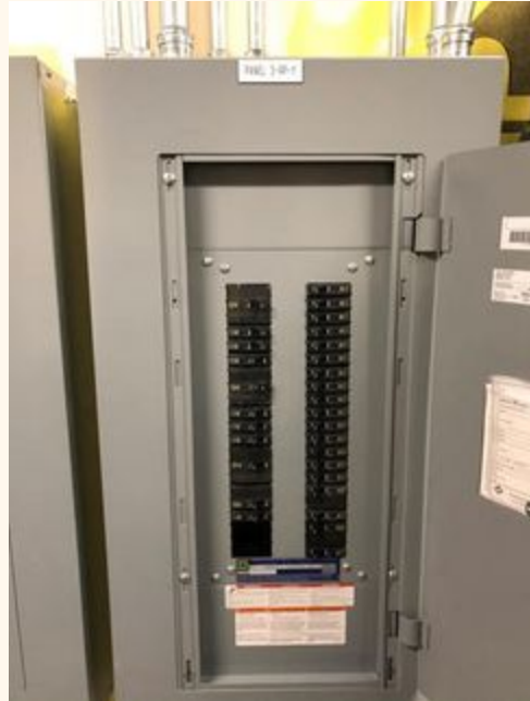
Unlabeled Circuits in Panel 3lp-1
