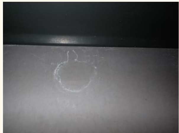
Moisture and Staining on Floor Below Connection
