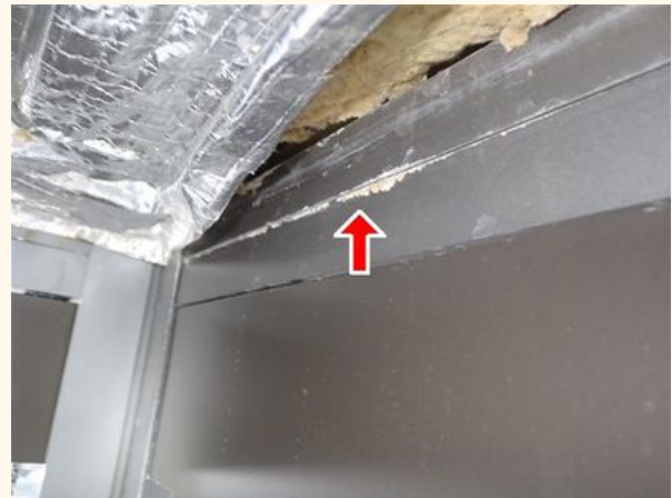
Incipient Leakage Stains Below Insulation
