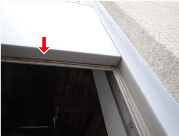
Corrosion and Deterioration Around Door Seals
