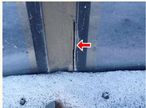
Gaps Noted in Caulking Around Windows
