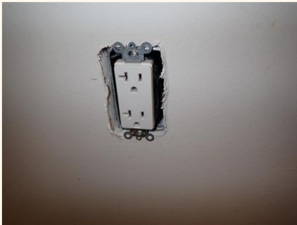
Receptacles Missing Covers
