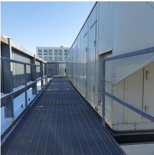
AAON Roof Mounted HVAC Air Handler System.
