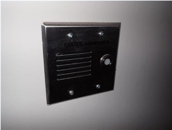
Low Voltage Communication Equipment
