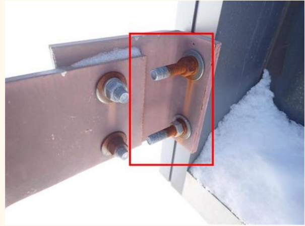
Corroding Connecting Bolts
