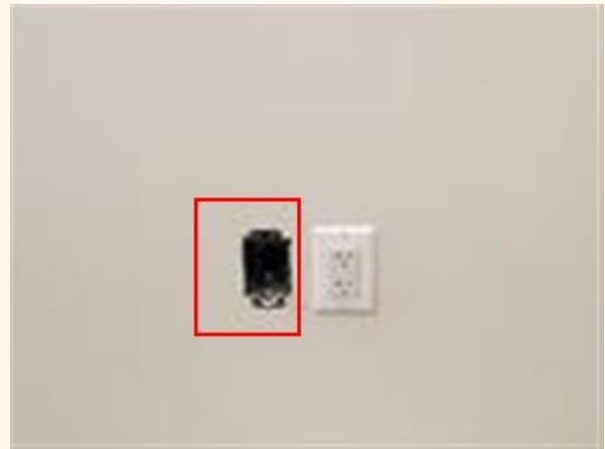
Open Junction Boxes
