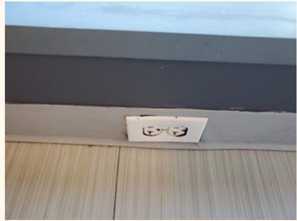
Loose Receptacle with Damaged Cover
