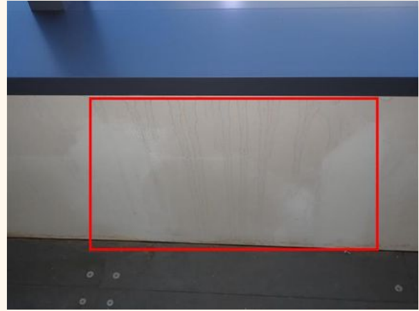
Moisture Stains on Wall Areas Below Windows
