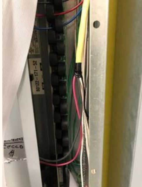
Romex Noted in Panel 3lp-1
