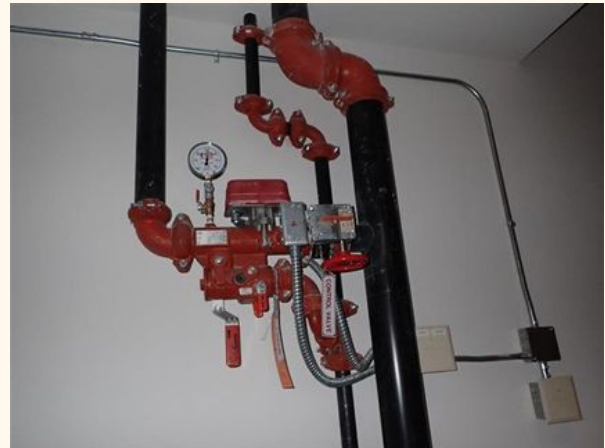
Fire Suppression System in Building
