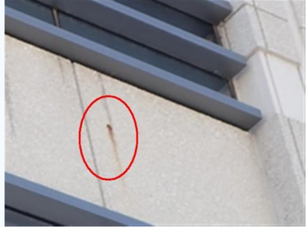
Corrosion Noted on Panels
