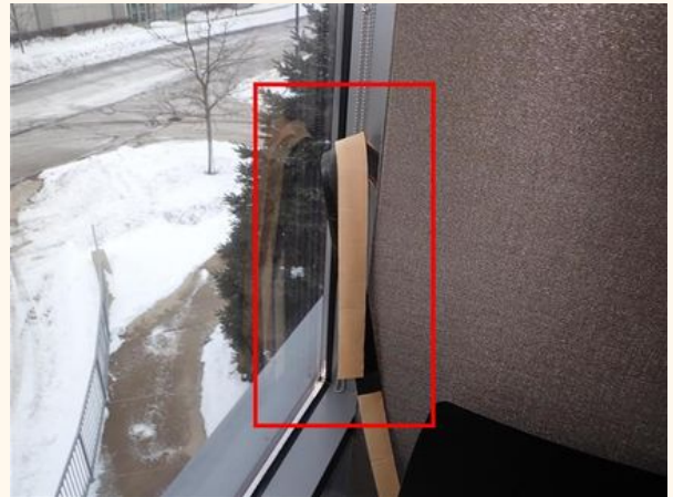
Loose Material on Workspace Enclosure
