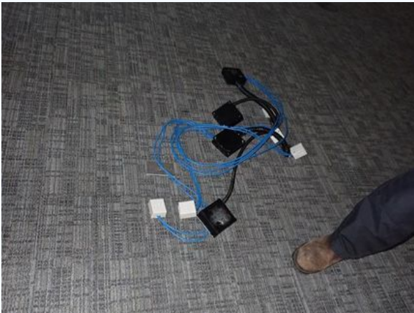
Numerous Abandoned Low Voltage Communication Wiring
