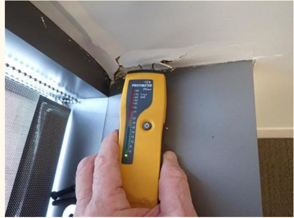
No Active Moisture in Badly Damaged Area
