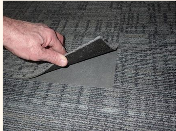
Loose Carpet Squares that Present Trip Hazards
