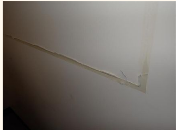
Damaged Wall Finishes Noted
