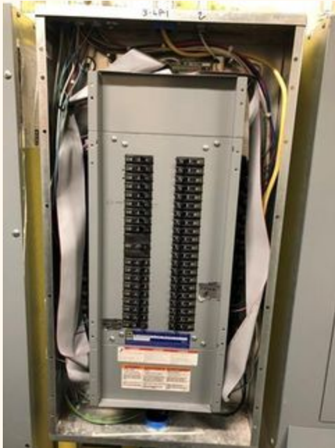
Unlabeled Circuits in Telecom Electric Room
