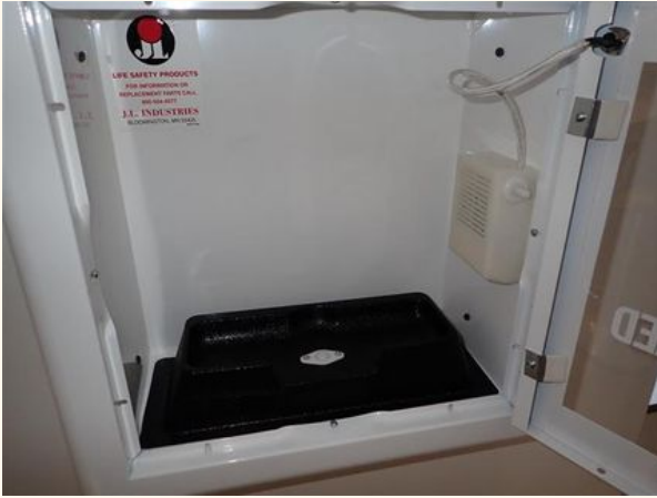
Missing Extinguishers in Some Enclosures
