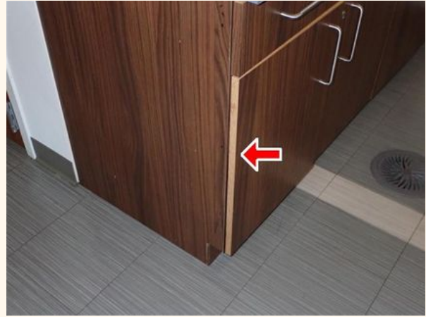
Missing Edges on Cabinets
