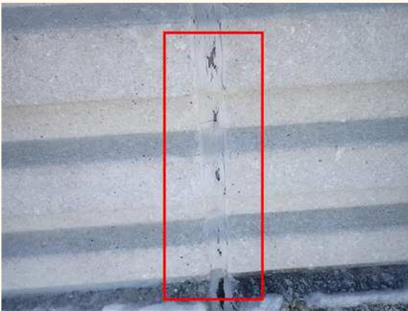
Deteriorated Caulk Between Pre-cast Cladding Panels
