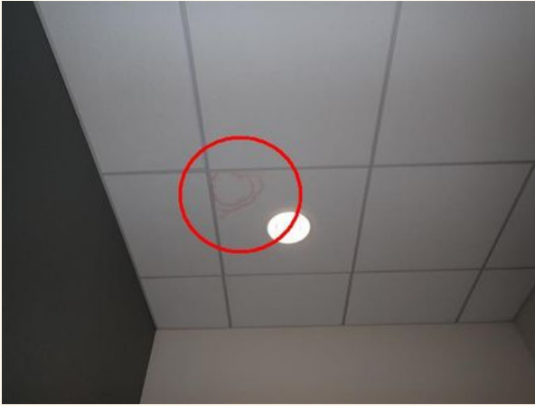
Ceiling Stains Noted in at Least Two Locations
