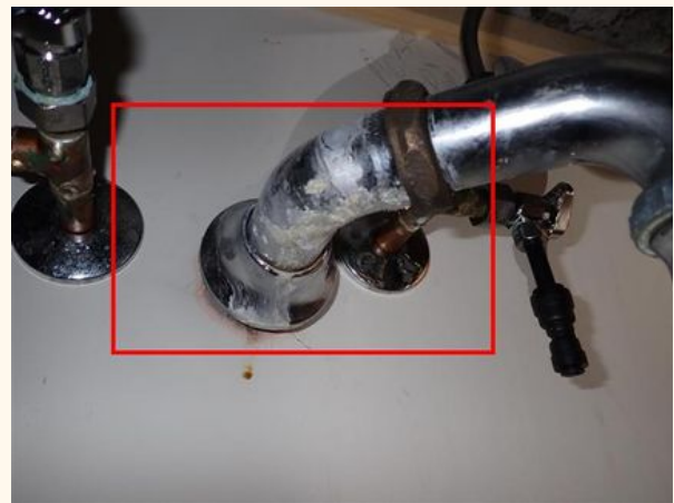
Incipient Leakage Stains on Sink Drain Piping
