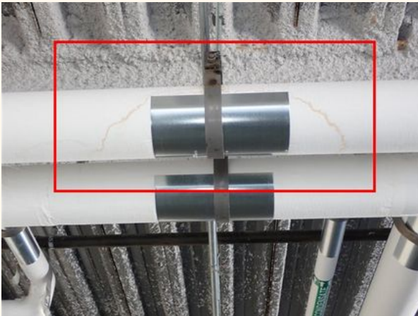
Potential Moisture Stains on Insulation for Suppression System Piping
