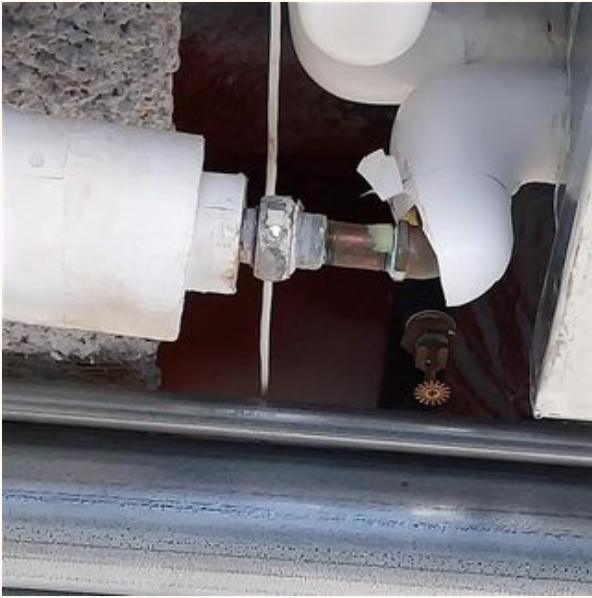
Missing Pipe Insulation.
