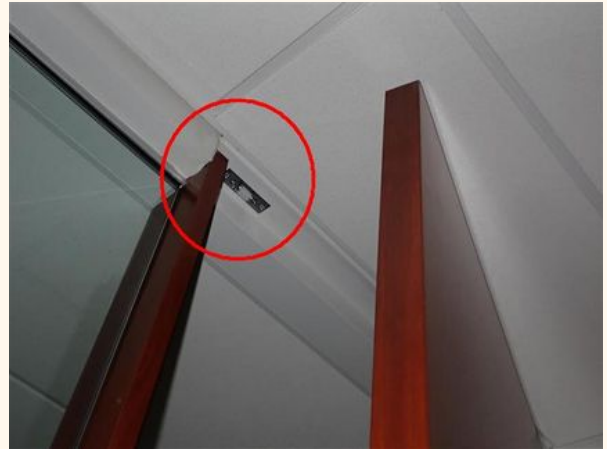
Several Non-latching Roller Top Doors Noted
