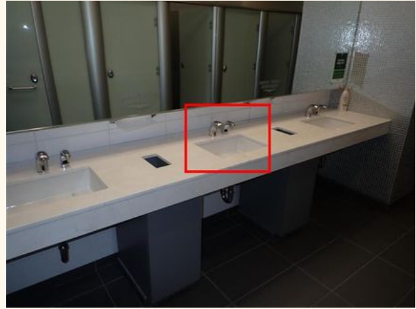
Non-responsive Sink in Upper Level Bathroom
