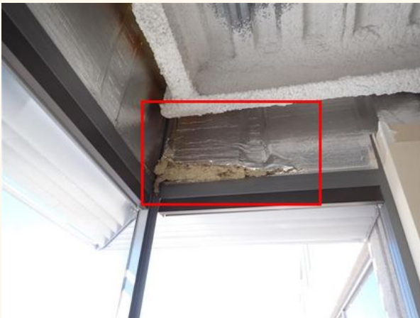
Loose Insulation Above Window
