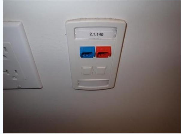
Low Voltage Communication Equipment
