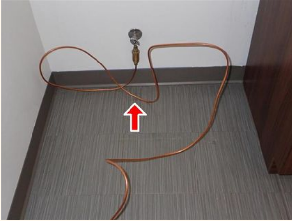
Copper Water Supply Utilized for Removed Refrigerator
