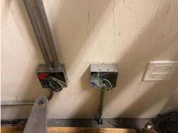
Uncovered Junction Boxes in Telecom Electric Room
