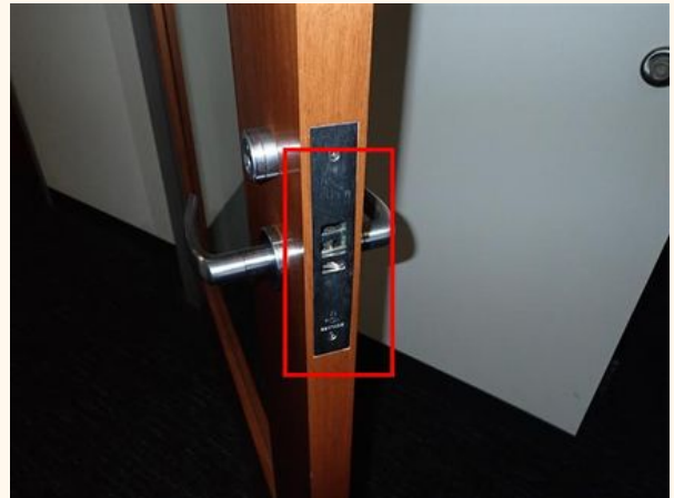
Non-operational Catch on Door
