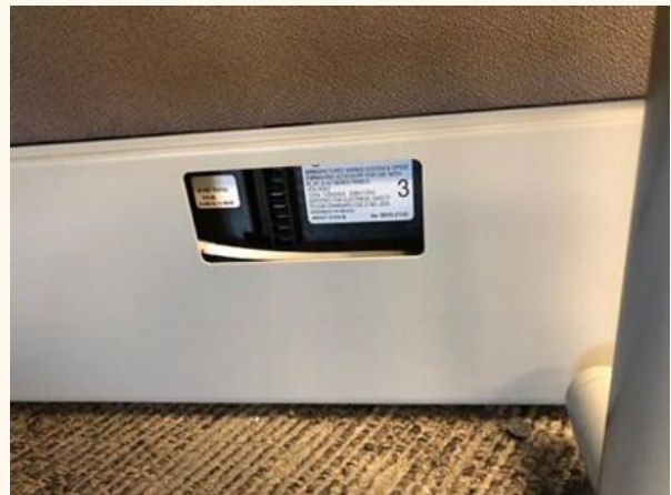
Open Power Bar in Cubicle in Room 290
