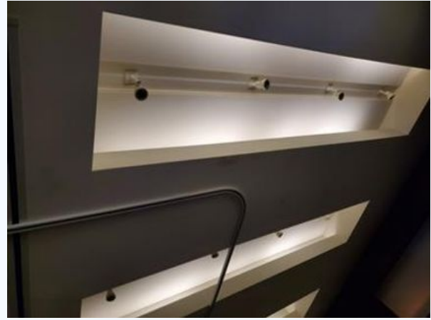
Non-functional Track Lighting
