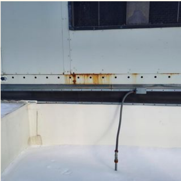
Rust and Corrosion on Evaporative Condensing Section (West unit)
