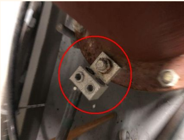
Missing Tag and Jumper Wire on Water Service Ground Connection
