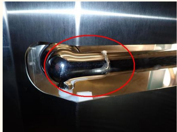
Leaking Fittings on Sink Drain Piping
