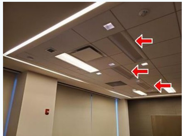
Non-functional Recessed Lighting
