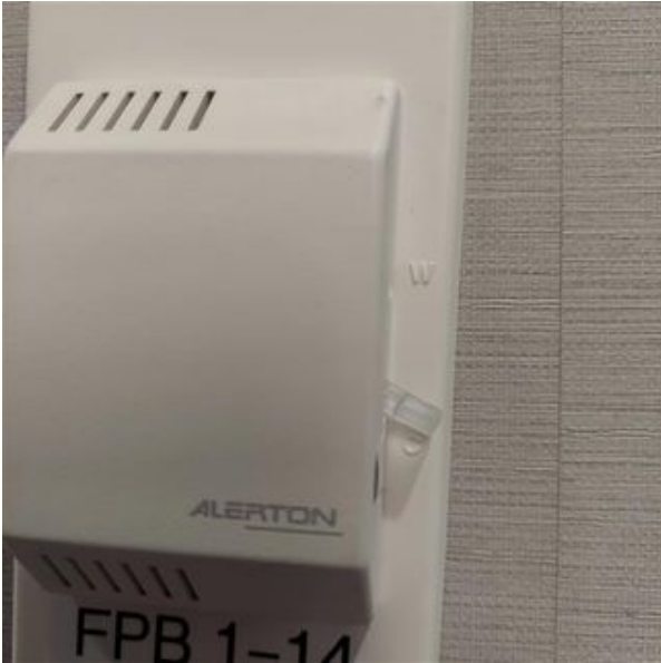
Fan Powered VAV Box Temperature Sensor
