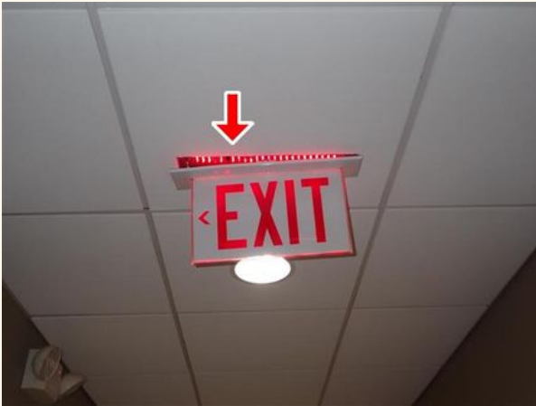
Loose Exit Sign
