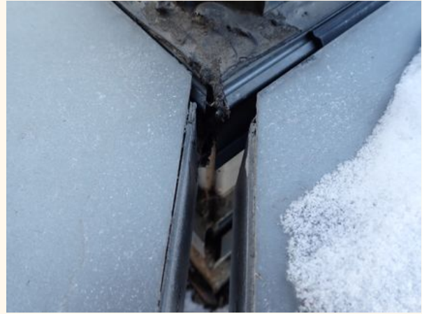
Multiple Layers of Materials in Difficult to Seal Corner Locations
