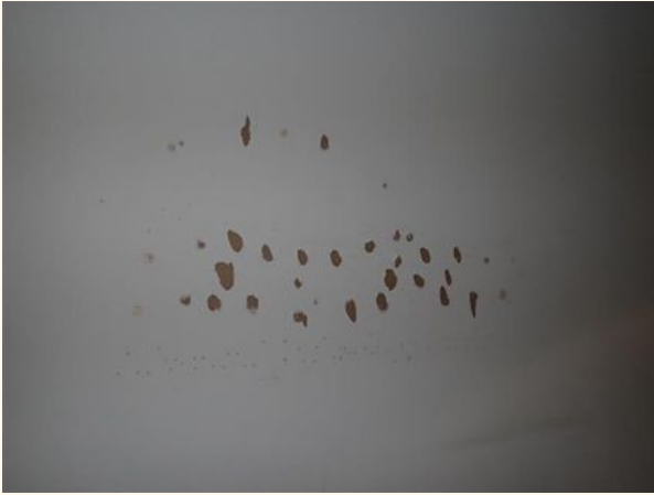
Damaged Wall Finishes
