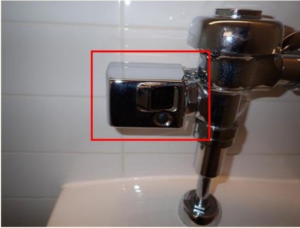
Non-functional Self Flushing Mechanisms Noted
