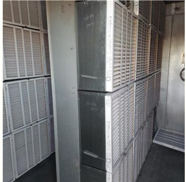
HVAC System Filter Section
