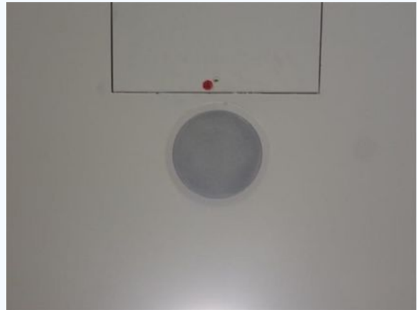
Low Voltage Audio Equipment
