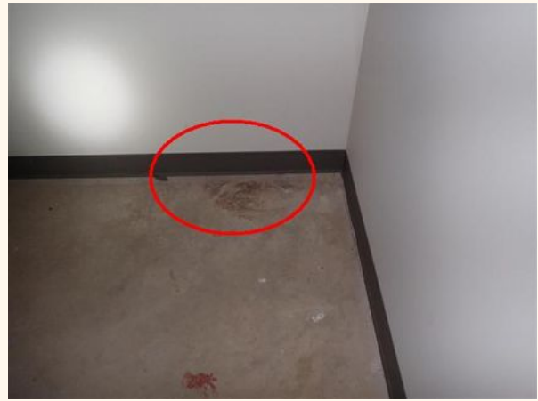
Staining on Floor Below Leakage Stains
