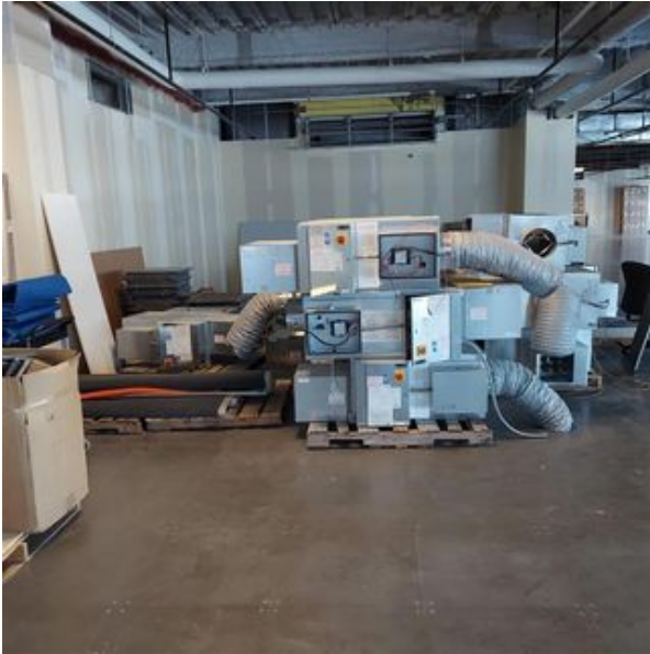
Spare Fan Powered VAV Boxes
