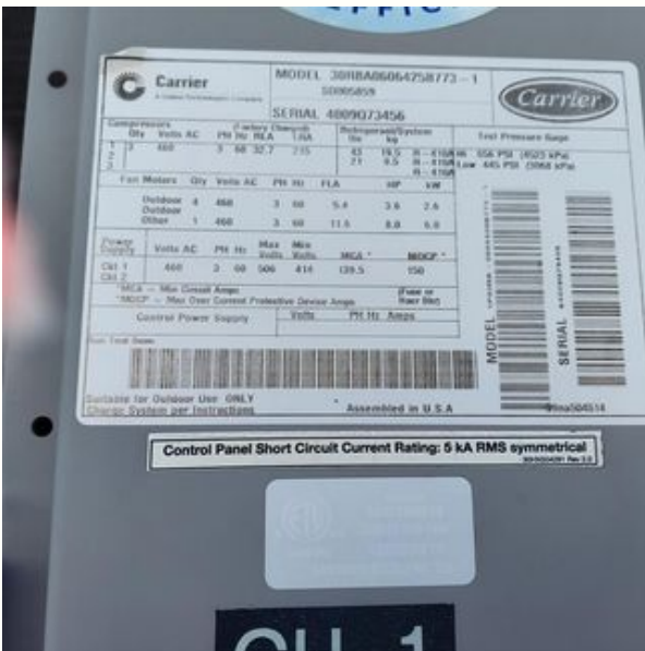
Chiller Data Plate
