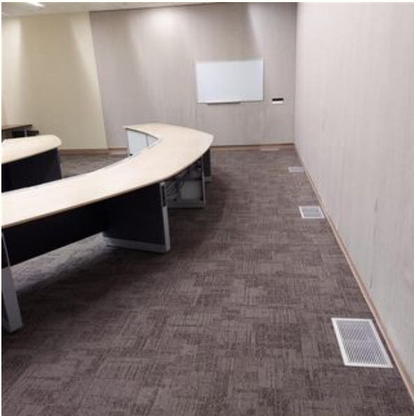
Typical Linear Floor Diffusers
