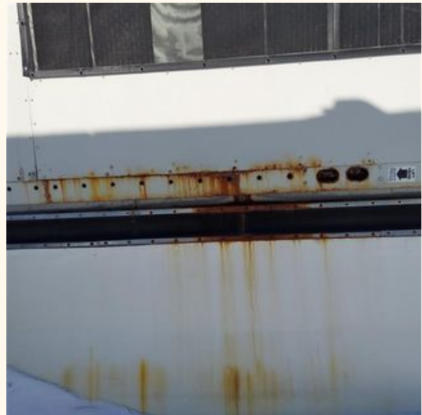
Rust and Corrosion on Evaporative Condensing Section (East unit)
