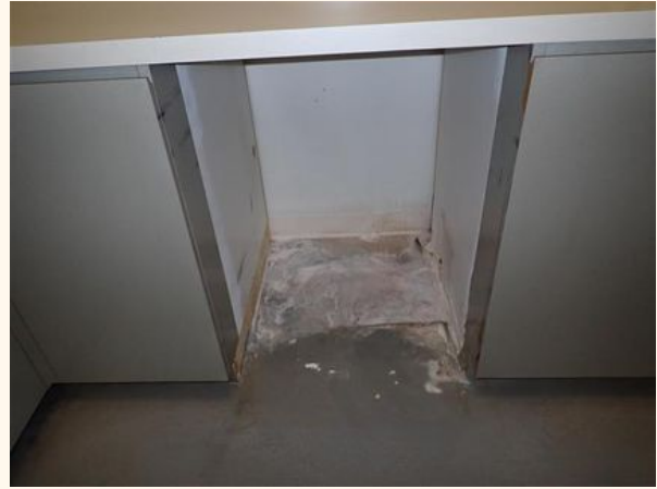
Damaged Finishes Adjacent to Removed Dishwasher
