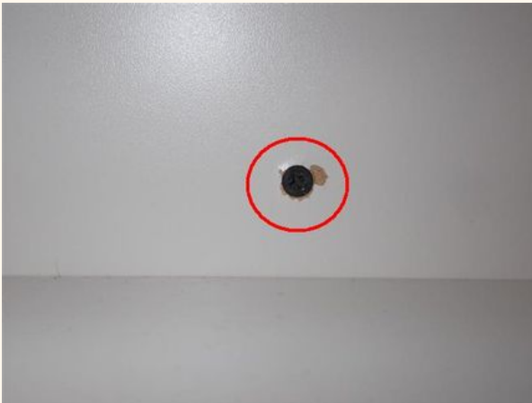
Drywall Screws Used to Secure Some Cabinets
