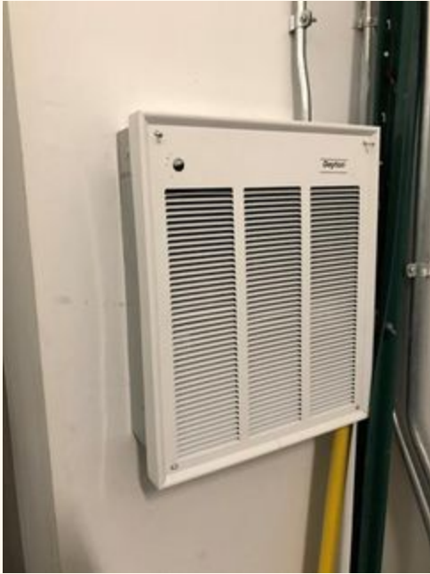
Loose Covers Noted on Heaters
