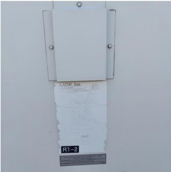
AAON Rooftop HVAC Data Plate Illegible
