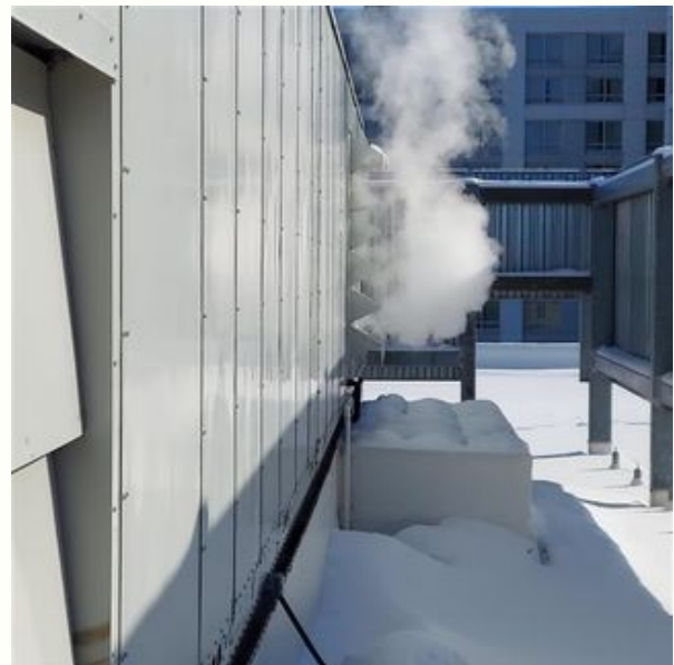
HVAC System Heating Section in Operation
