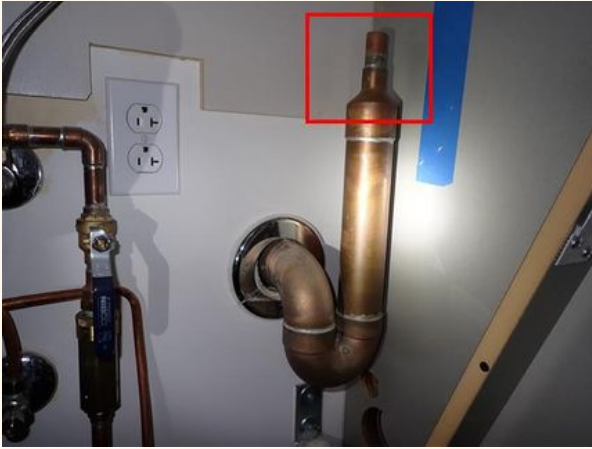
Uncapped Dishwasher Drain
