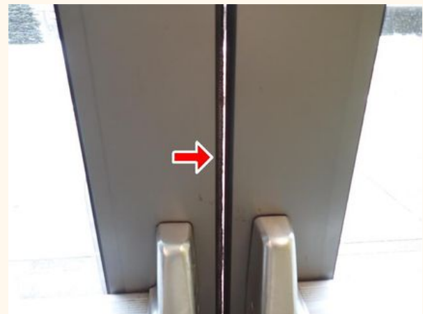
Gaps Noted Between Doors
