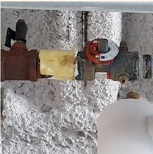
Missing Pipe Insulation.
