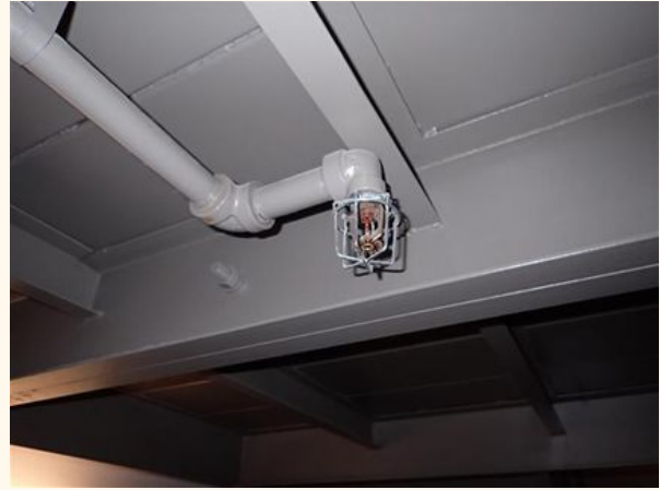
Protective Cover on Sprinkler Head
