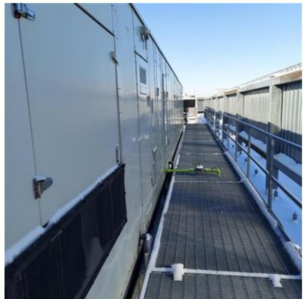
AAON HVAC Unit with Evaporative Condenser
