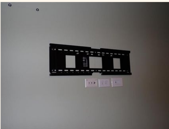
Numerous Wall Mounts Noted
