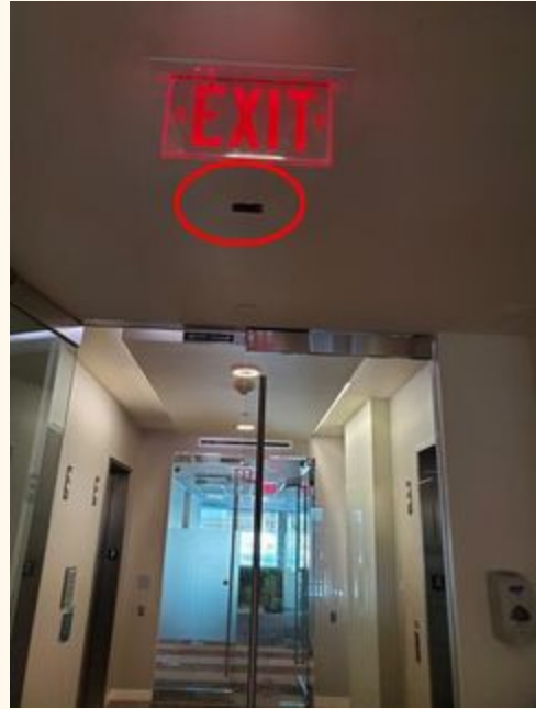
Open Ceiling Boxes Noted
