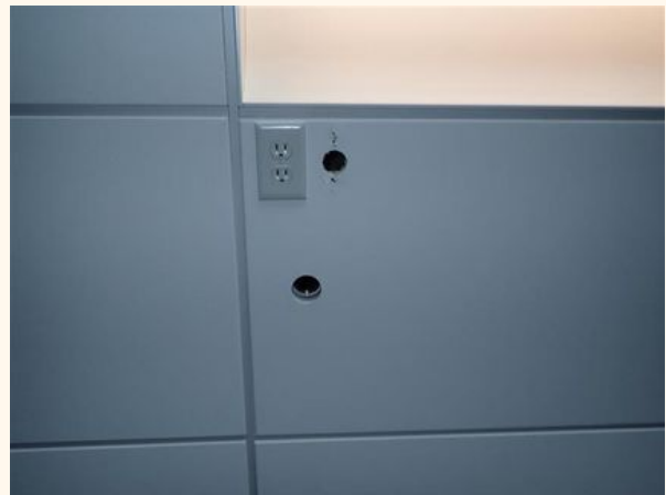
Holes in Wall
