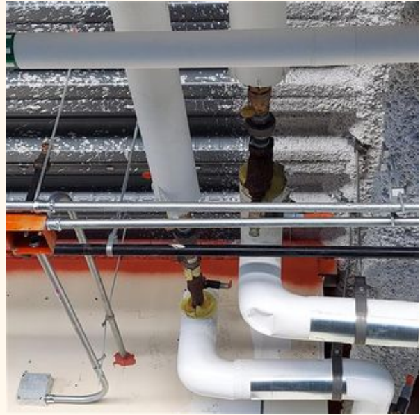
Missing Pipe Insulation.
