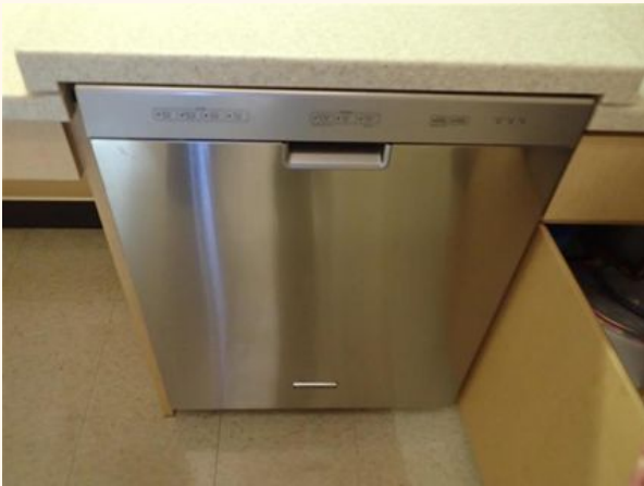
Shut-off Switch Missing on Dishwasher
