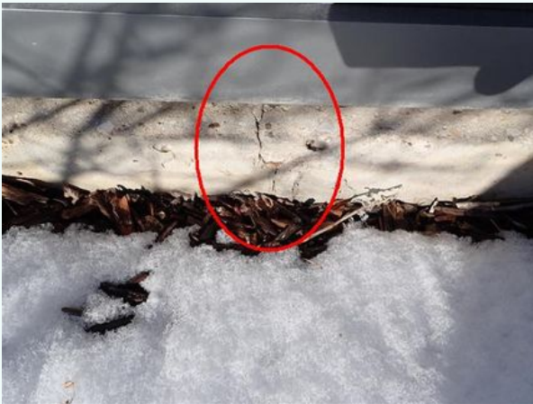
Minor Cracks Noted on Exterior of Foundation
