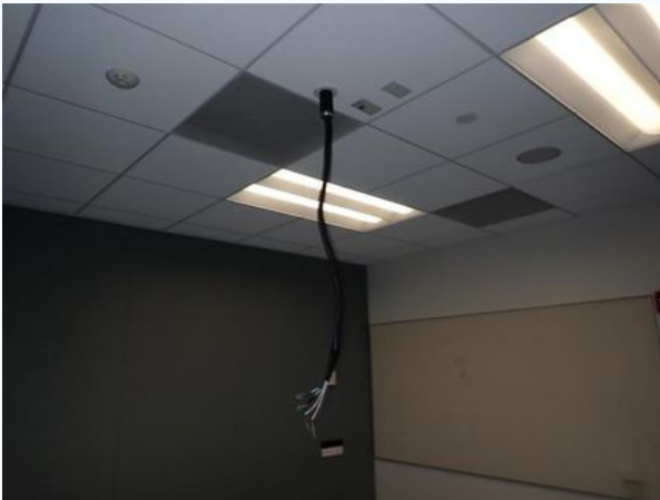
Low Voltage Cables Dangling From Ceiling
