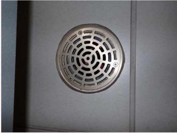
Open Floor Drains in All Bathrooms
