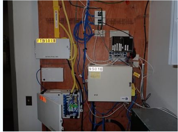
Low Voltage Communication Equipment
