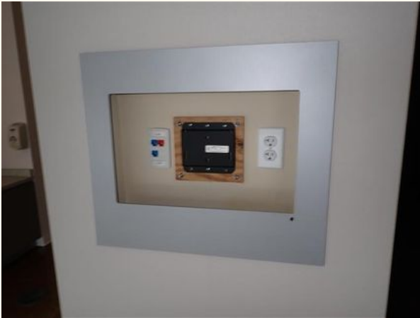
Numerous Abandoned Wall Mounts
