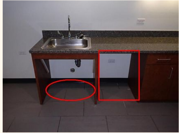
Removed Dishwasher Space and Moisture and Staining Below Sink
