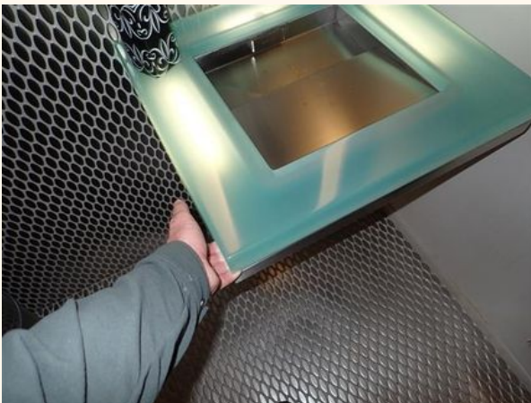
Loose Counter on Bathroom Sink
