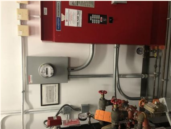
No Grounding Observed on Fire Pumping System
