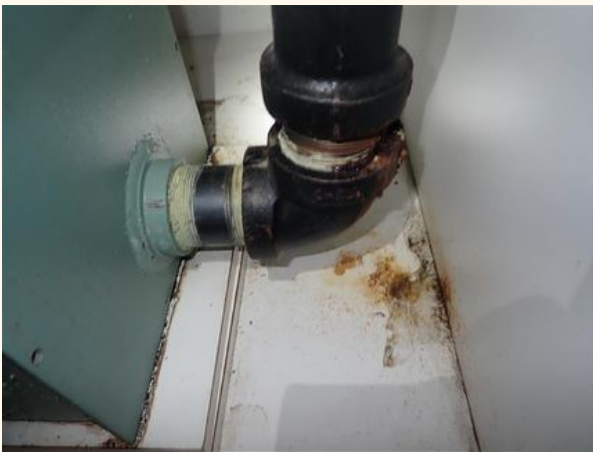
Leaking Grease Trap Below Sink
