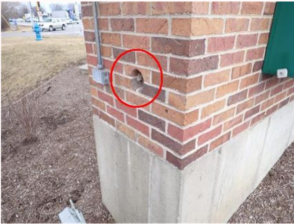
Open Hole on Sign
