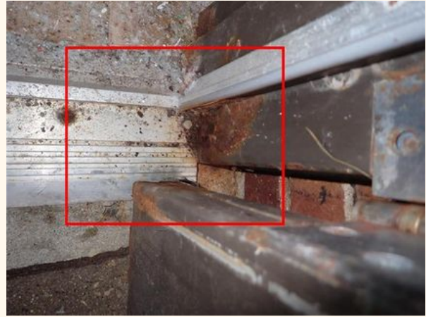
Corroded Doorframe on Rear Entry
