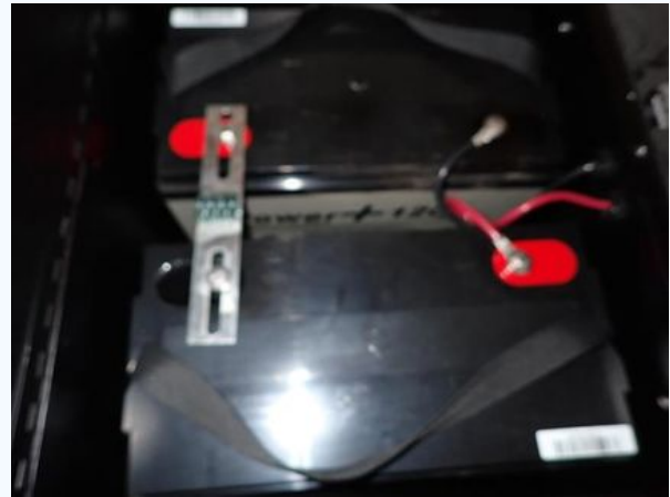
Batteries Inside Unit
