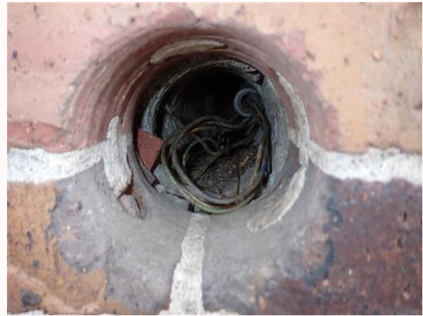
Exposed Wiring in Sign
