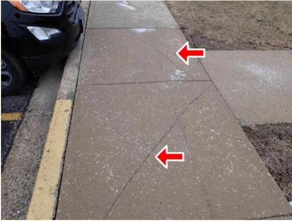
Cracks in Walks
