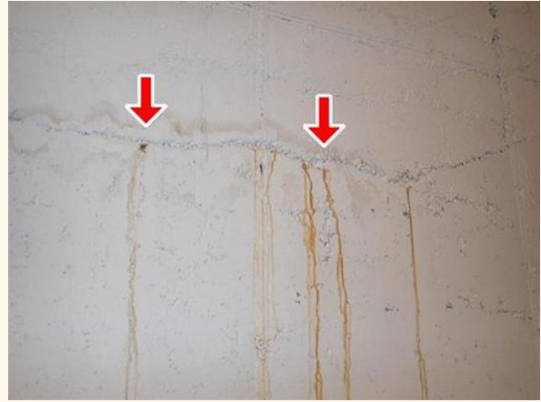
Leakage Along Cold Joint
