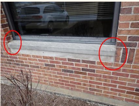
Mortar Joints in Corners of Stone Sills
