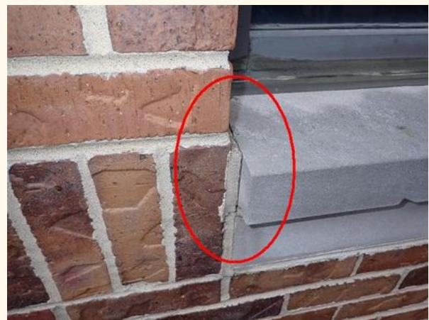
Hairline Cracking Observed in Mortar Joints
