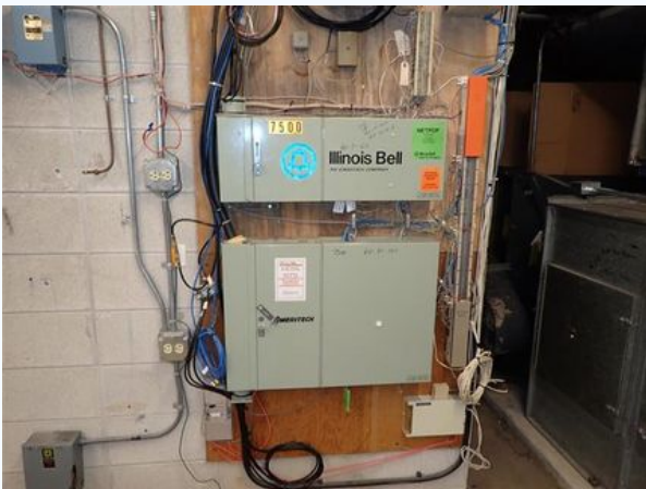
Low Voltage Communication Equipment
