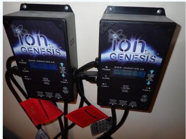
Back-up System Controllers
