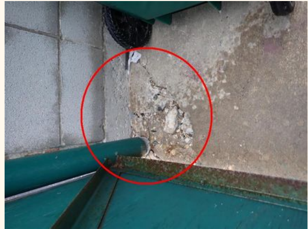
Cracked Areas by Posts
