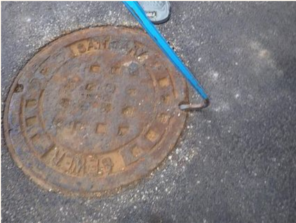
Corroded Manhole Cover
