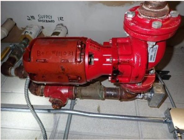
Excessive Oil on Circulating Pump
