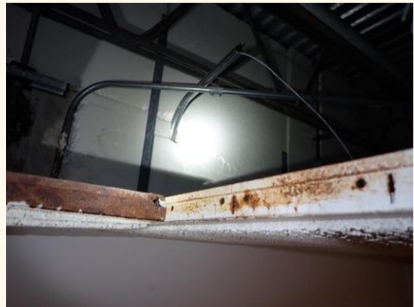
Damaged Ceiling Tile System
