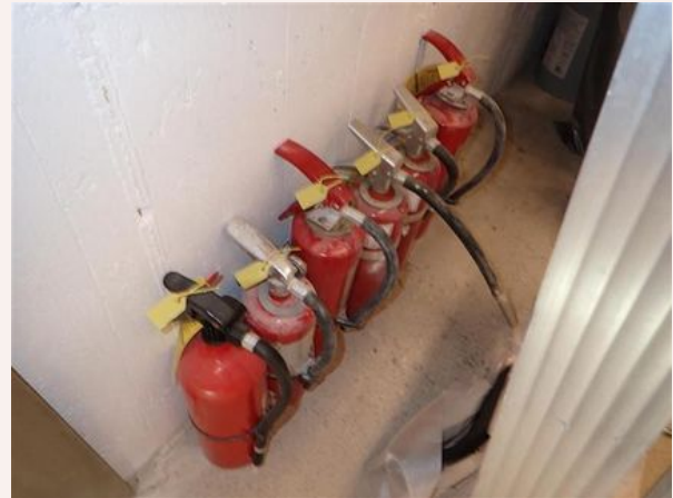
Stored Extinguishers in Bank Vault
