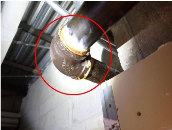
Oil Observed on Pipe by Elevator
