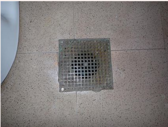
Open Floor Drains in Every Bathroom
