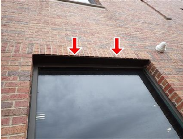
No Drip Edge Observed Above Windows
