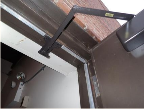
Gap in Weatherstripping Around Rear Entrance Door
