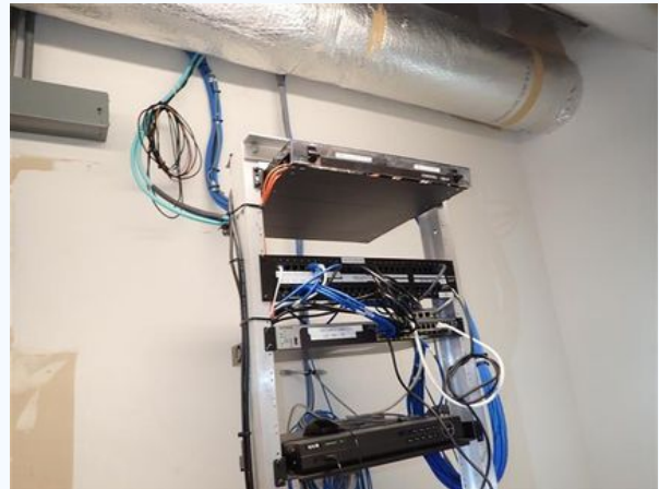
Low Voltage Communication Equipment
