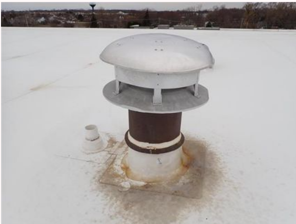
Moisture Stains Around Boiler Vent Pipe
