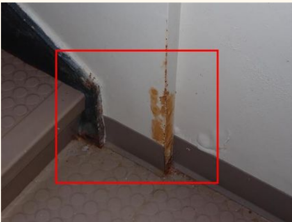
Moisture Stains and Damage on Stairwell Walls
