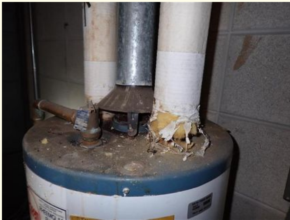
Corrosion and Staining on Water Heater
