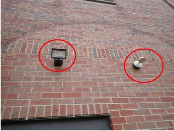
Extinguished Bulbs on Exterior
