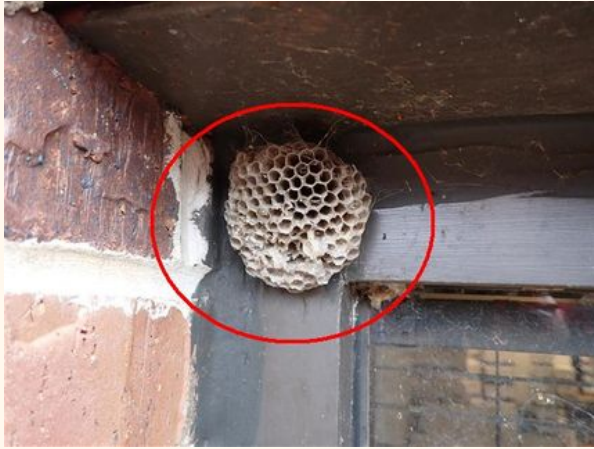
Numerous Nests Noted on Exterior of Structure
