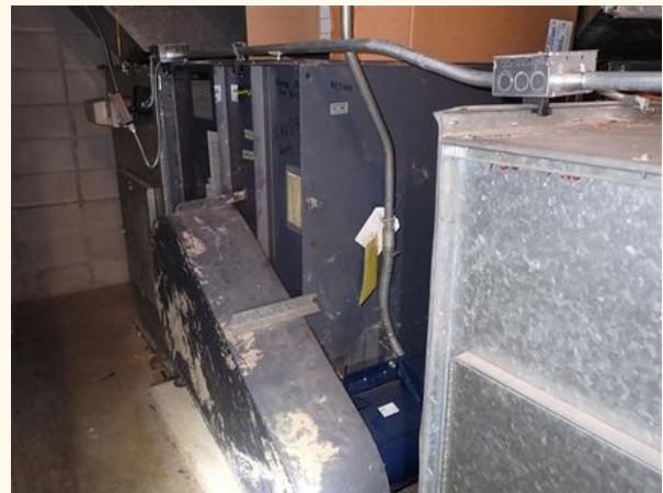
One of Two Air Handlers in Mechanical
