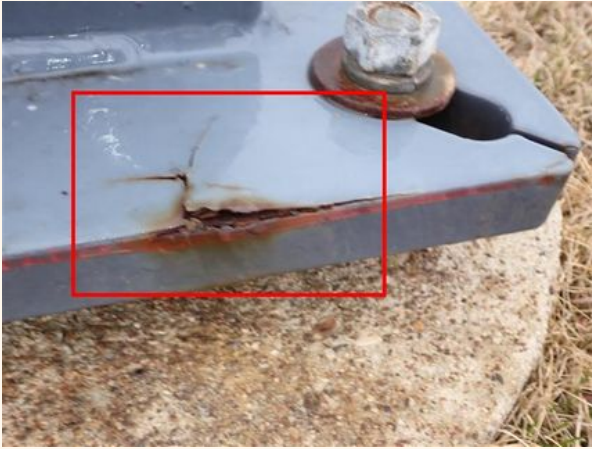
Corrosion on Light Pole Base
