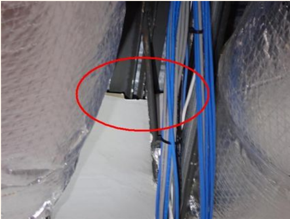
Holes in Walls of Server Room
