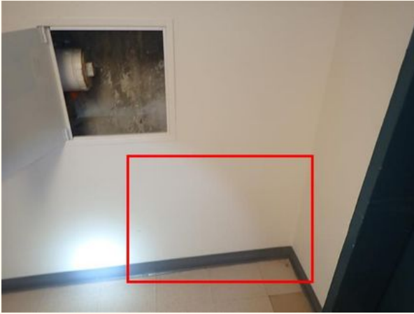
Moisture Related Damage by Elevator
