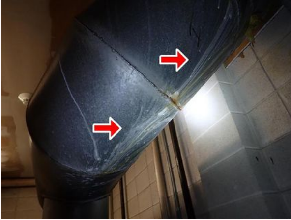
Moisture Stains and Corrosion on Vent Pipe
