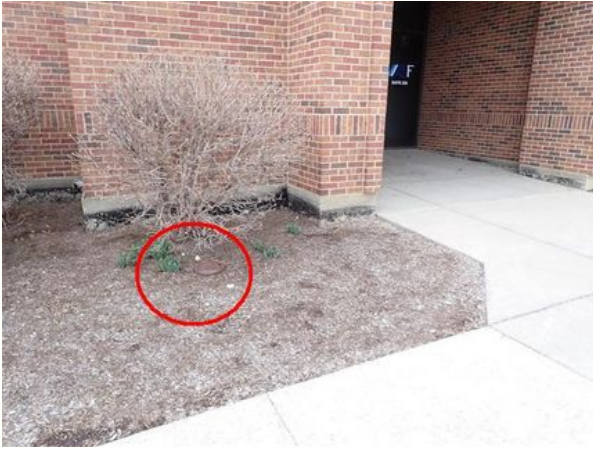
Exterior Shut-off Valve Location
