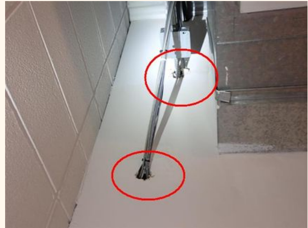
Holes in Wall of Server Room
