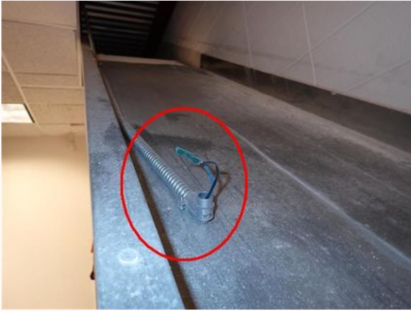
Live Wiring by Former Mail Chute
