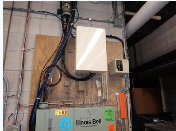
Low Voltage Communication Equipment
