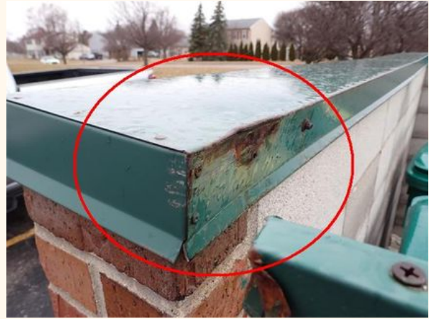
Damage and Corrosion on Cap
