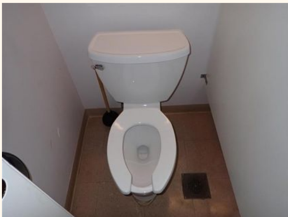
Loose Toilets in Nearly Every Bathroom
