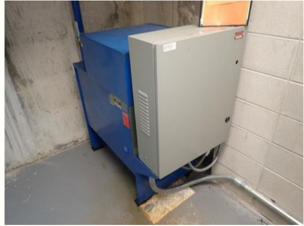
Elevator Mechanical Unit
