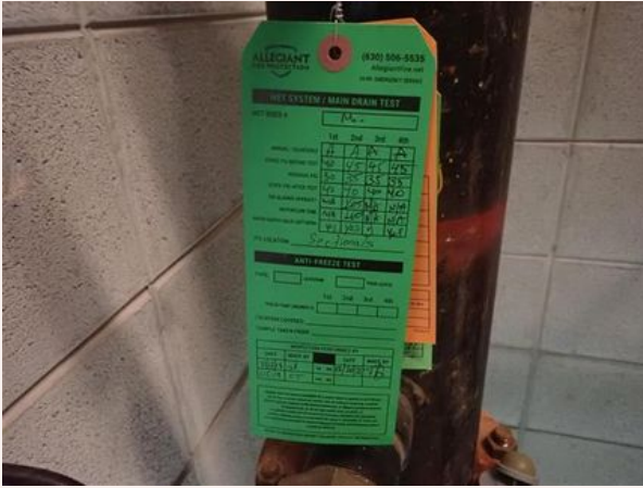
Service Tag Shows Recent Servicing
