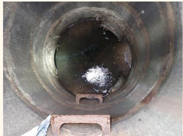
Standing Water in Inlet in Parking Lot
