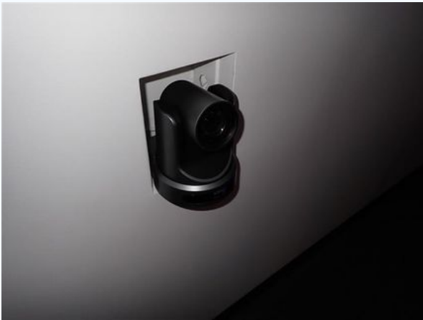
Low Voltage A/V Equipment
