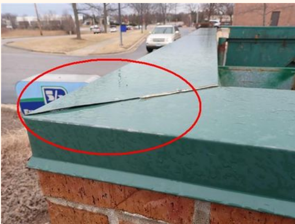
Unsealed Corner Joints on Caps
