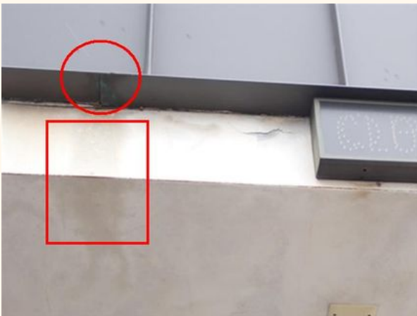
Moisture Stains on Façade Shelf and Damaged Fascia Below
