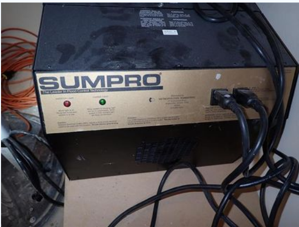
Battery Back-up System for Sump Pump
