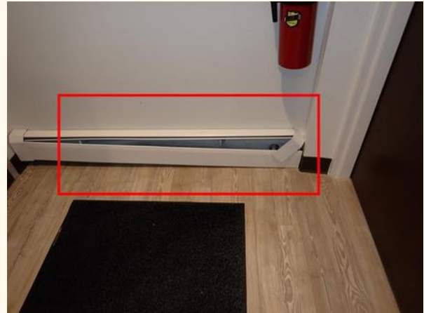
Damaged Radiator Cover
