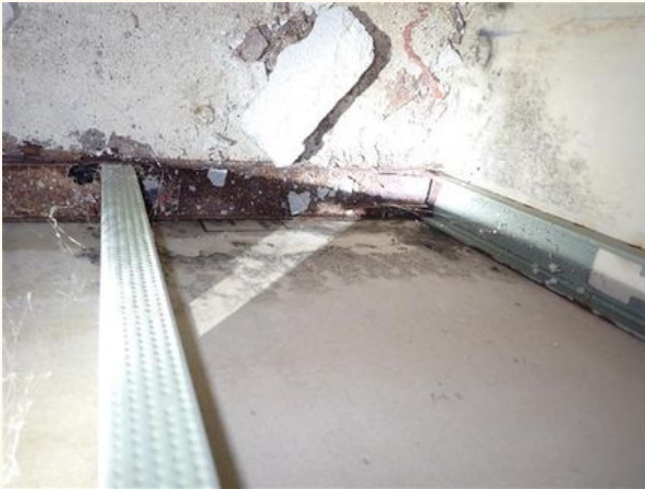
Corrosion on Framing by Elevator
