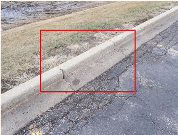
Cracked Curb Sections
