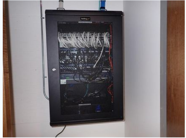
Low Voltage Communication Equipment
