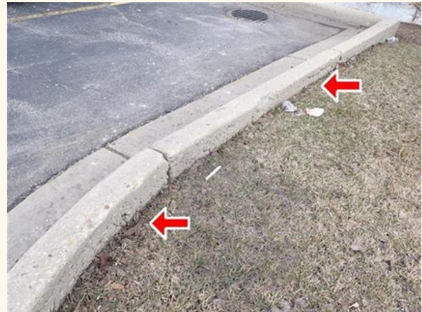
Unsupported Curb Backs
