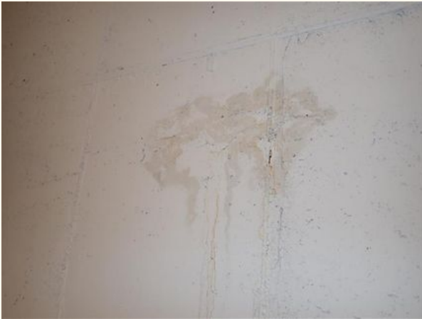
Leakage Through Honeycombed Area
