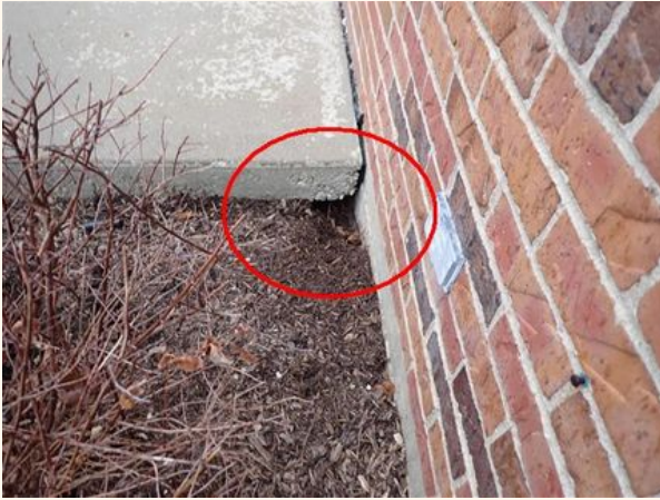
Hole Beneath Rear Sidewalk
