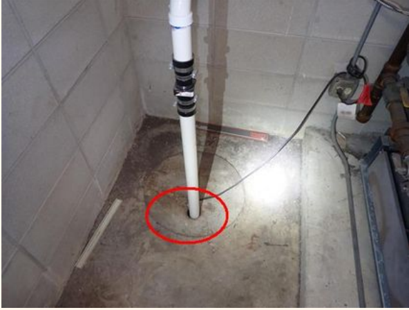
Unsealed Sump Pit
