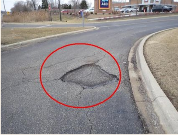
Large Hole in Apron by Grand Ave
