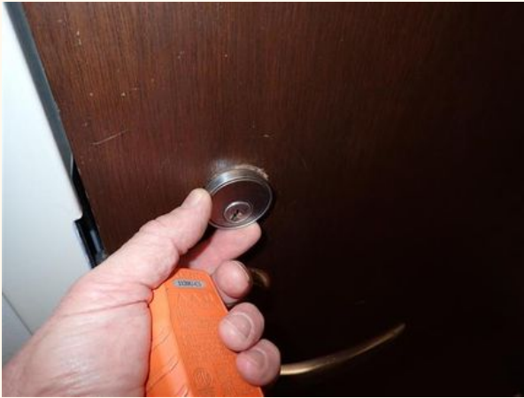
Loose Lock Mechanism on Basement Closet
