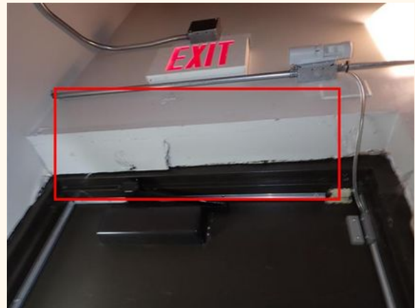
Damage Noted Above Rear Entry Door
