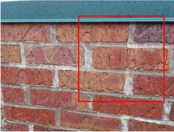
Cracks Noted in Masonry Below Cap
