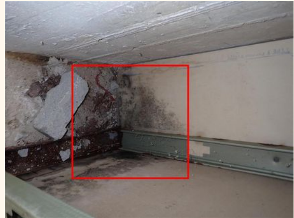
Mold-like Substance Noted in Wall Areas
