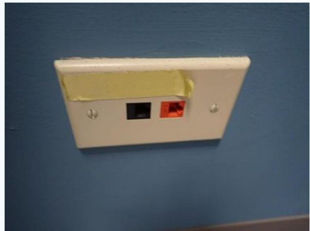
Low Voltage Communication Equipment
