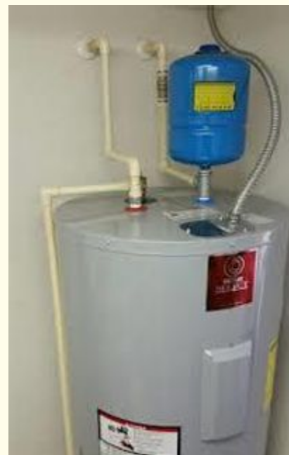
Water Heater Expansion Tank
