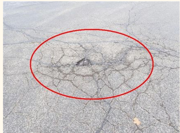
Severely Deteriorated Asphalt Areas Noted
