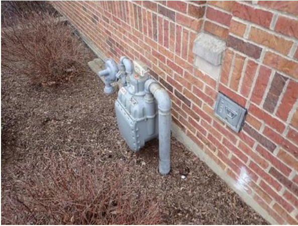
Natural Gas Supply and Shut-off
