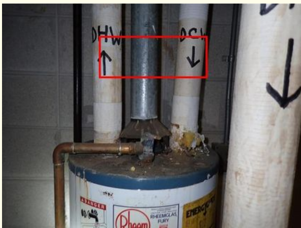
Expansion Tank Needed on Water Heater
