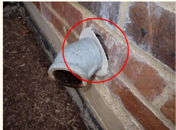
Unsealed Wall Penetration by Sprinkler Drain
