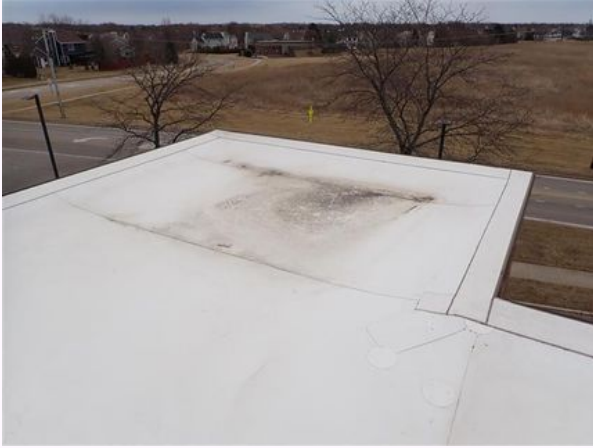
Small Ponding Area on Roof
