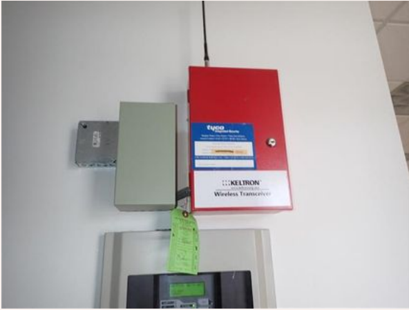
Fire Alarm System
