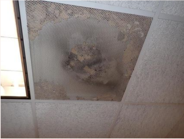
Heavy Dust Build-up on Diffusers
