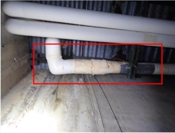
Leakage Stains on Pipe in Ceiling of Elevator Mechanical Closet
