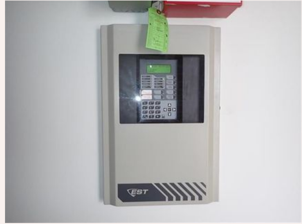
Fire Alarm System
