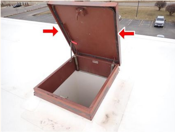
Older Seals on Edges of Roof Hatch
