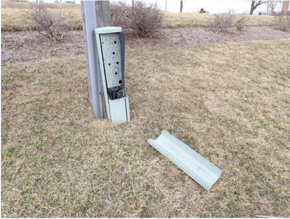
Loose Cover on Communication Pedestal in Front of Property
