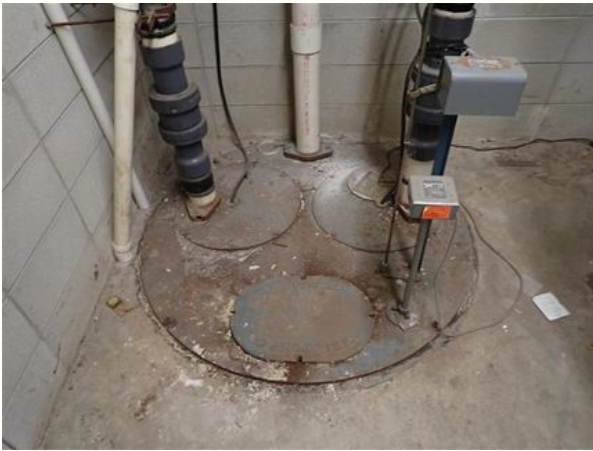
Ejector Pumps in Basement
