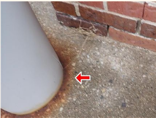
Corrosion Noted Around Bases of Bollards
