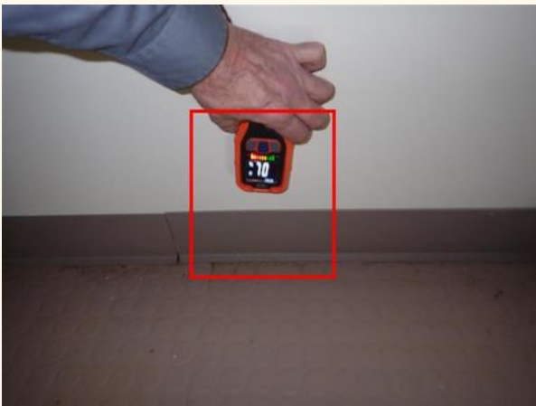
Elevated Humidity Measured in Areas with No Damage
