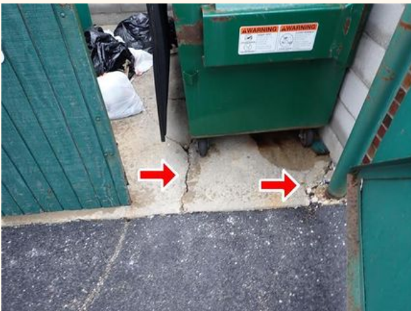
Cracked and Damaged Slab
