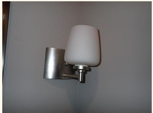
Extinguished Bulbs on Wall Fixtures
