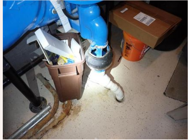
Drain for Fire System
