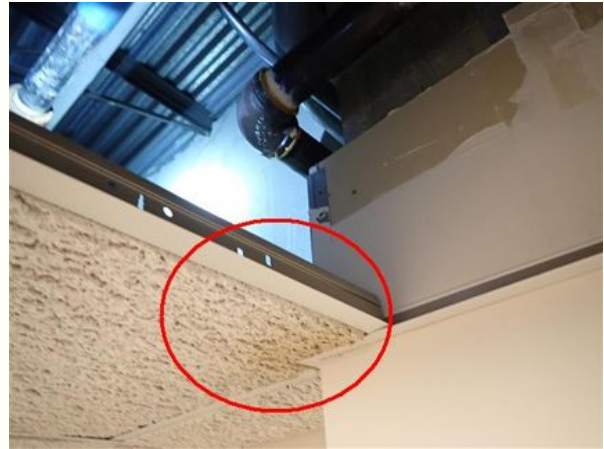
Stained Ceiling Tile by Elevator
