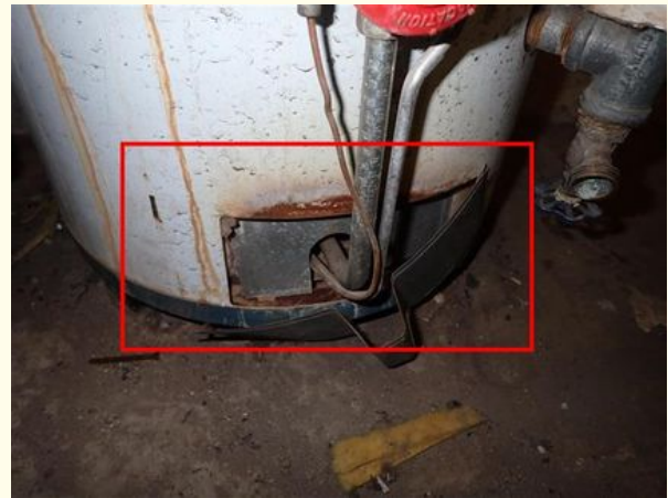
Displaced Cover on Burner and Corrosion on Unit
