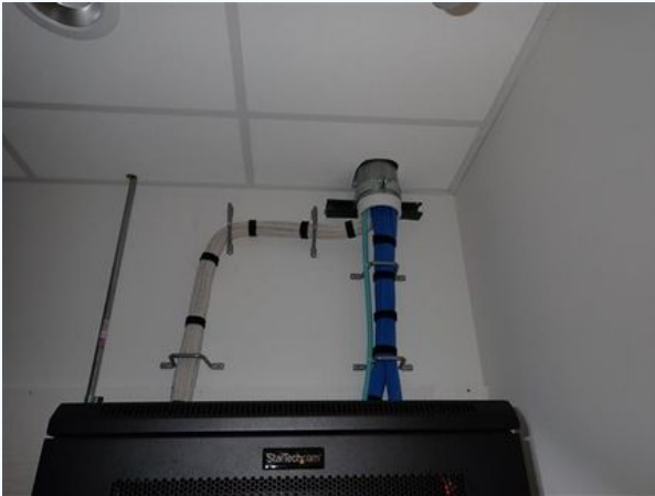
Low Voltage Communication Wiring
