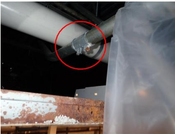
Corrosion on Conduits Connected to Junction Box
