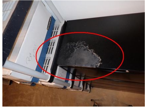
Moisture Stains on Cabinet Below
