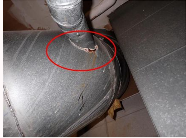
Corrosion and Staining by Water Heater Vent
