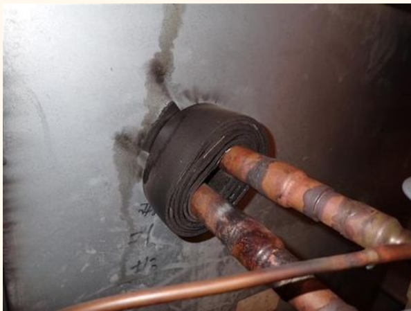
Leakage by Evaporator Coil Casing Penetrations
