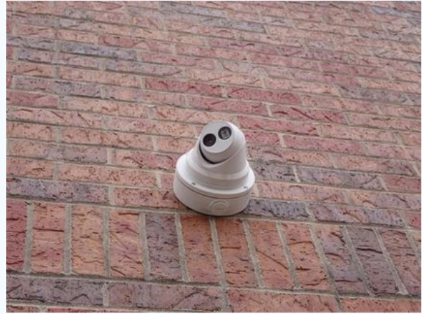
Low Voltage Surveillance Equipment
