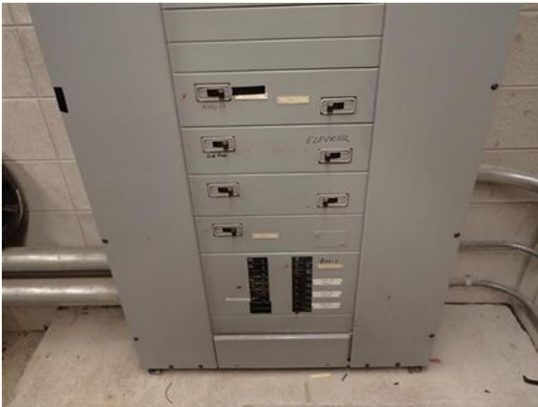
Main Service Panel
