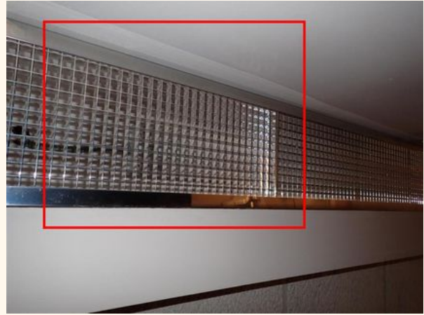
Extinguished Bulbs in Upper Level Bathrooms
