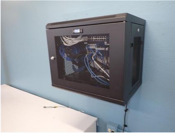
Low Voltage Communication Equipment
