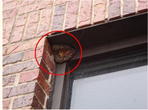
Numerous Nests Noted on Exterior of Structure
