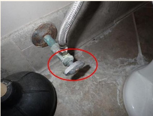
Gate Valves on Toilet Supplies
