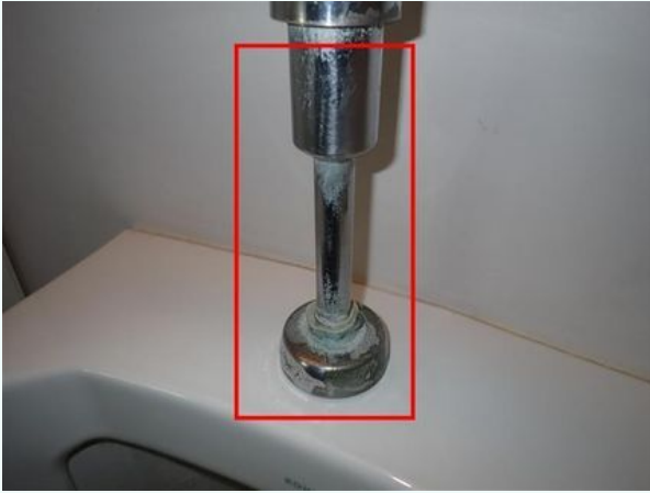
Incipient Leakage on Urinal Supply Piping
