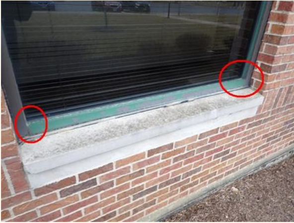
Unsealed Corners on Windows
