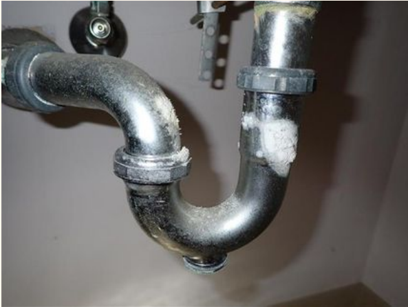
Corrosion on Drain Trap Piping
