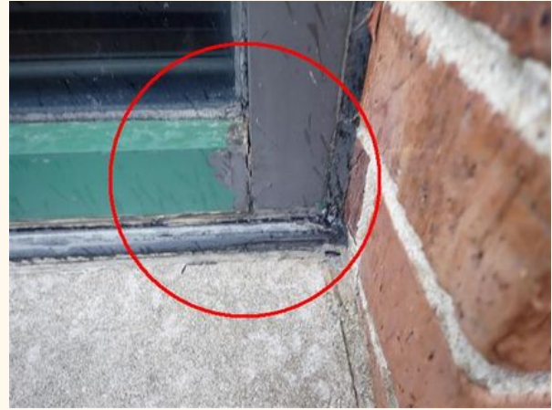
Cracks and Gaps in Window Corners
