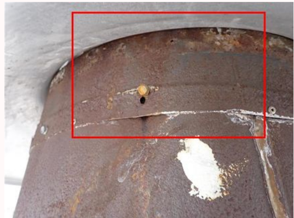
Corrosion and Open Holes on Vent Pipe
