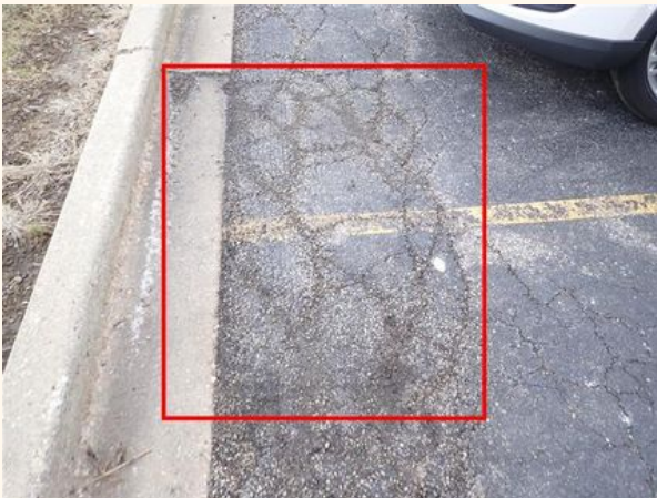
Cracked Paving by Curb
