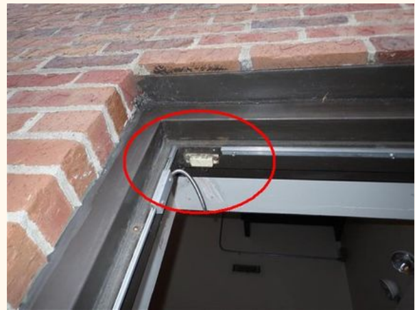
Gap in Weatherstripping Around Rear Entrance Door
