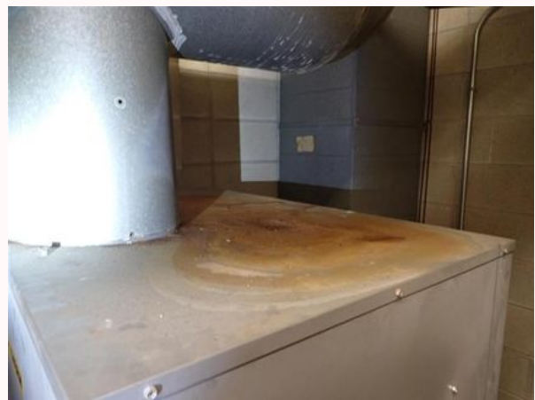
Staining and Corrosion on Top of Boiler
