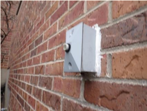
Extinguished Bulb on Exterior Wall
