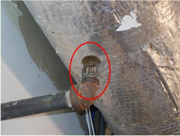
Fire Sprinkler Safety Heads Throughout Structure
