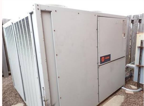
Large Older Condensing Unit
