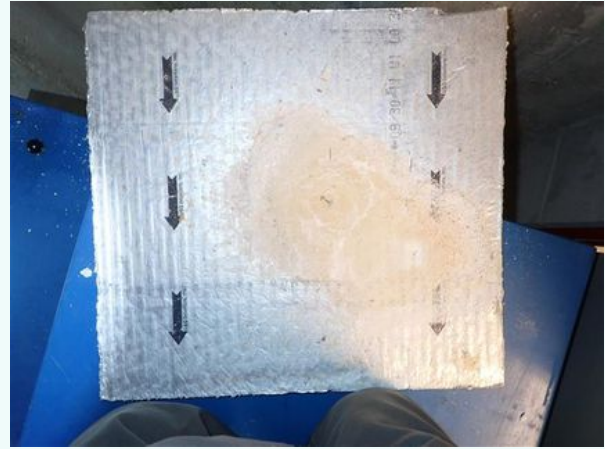
Stains on Panel Below Piping
