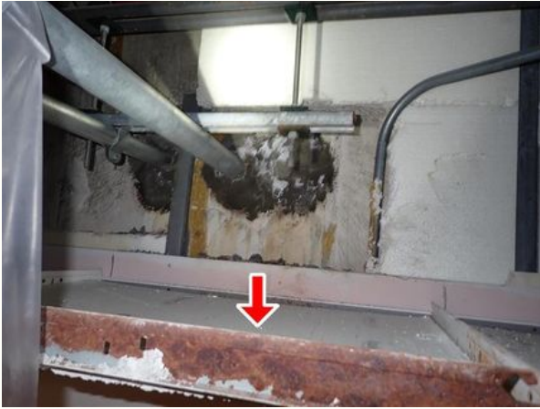
Corrosion on Ceiling Grid
