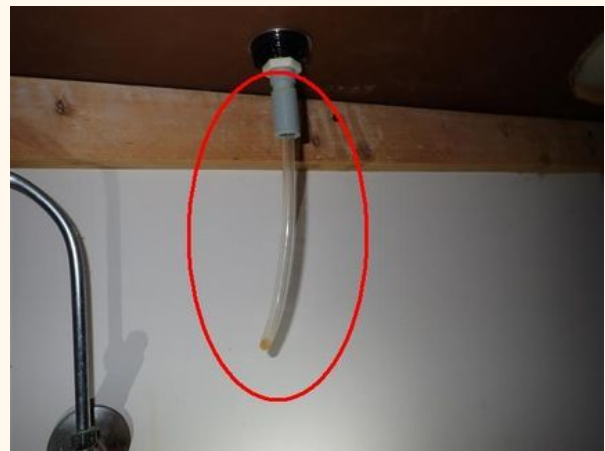
Missing Containers on Dispensers
