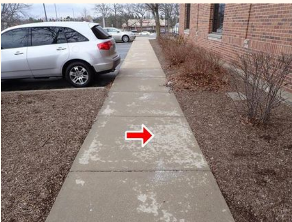
Sidewalk Slopes Towards Building
