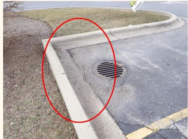
Curb Area by Inlet Holding Water
