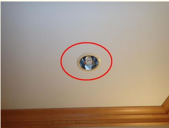
Extinguished Bulbs in Bathrooms
