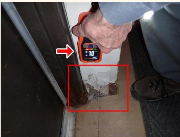
Damaged Wall Finishes and Elevated Humidity Around Rear Entry Door
