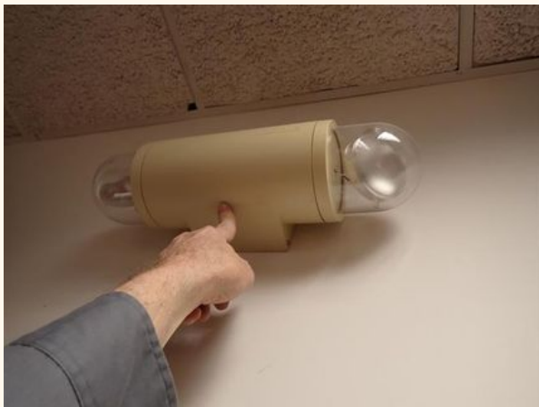
Non-functional Emergency Lighting in Former Unoccupied Mail Area
