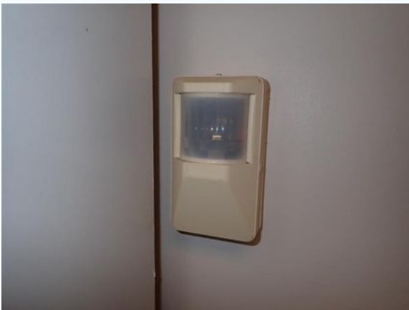
Low Voltage Alarm System
