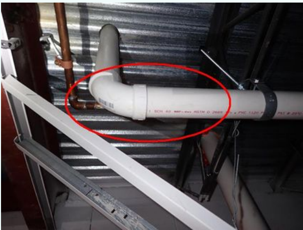
Stains on Piping Above Stained Tiles
