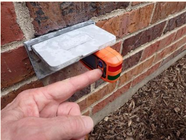
Non-GFCI Receptacles on Exterior of Structure
