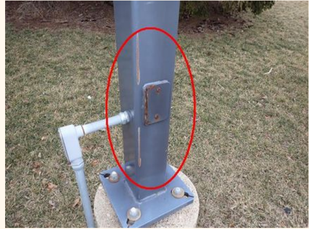
Corrosion on Light Pole
