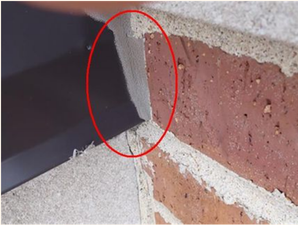
Weathered and Cracked Caulking on Roof Flashing Joints
