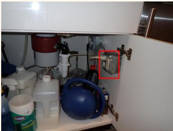
Switch for Disposer in Upper Level Kitchen
