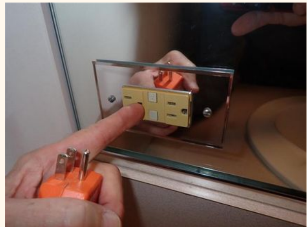
Non-functional GFCI Receptacle in Bathroom
