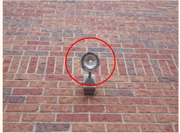
Extinguished Bulb on Exterior
