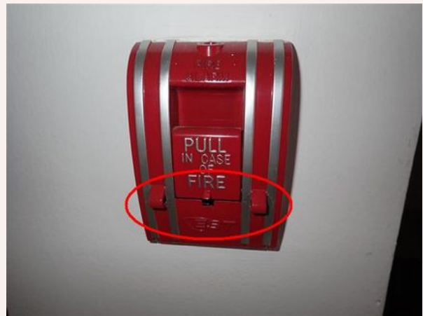
Missing Glass Indicator on Alarm Pull
