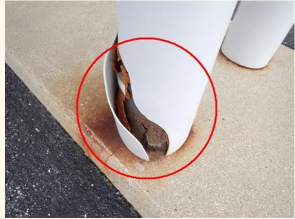
Corroded Bollard in Drive-thru
