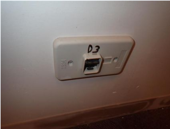
Low Voltage Communication Equipment
