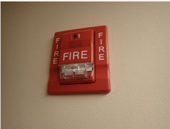
Fire Alarm System in Structure
