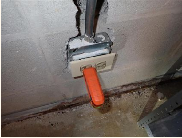
Loose Receptacles in Document Storage Room
