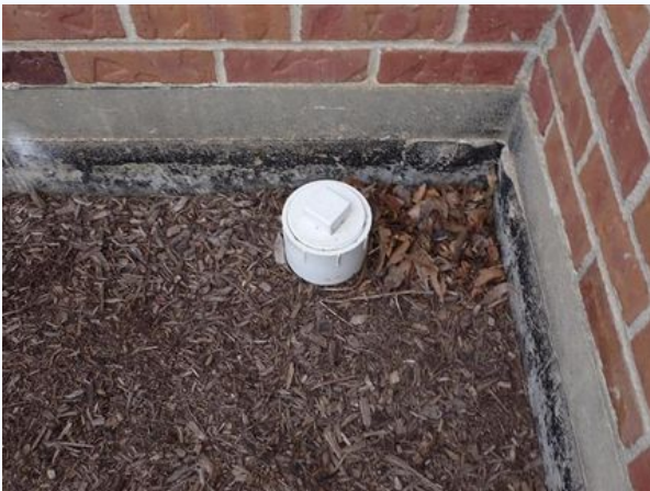
Clean-out in Corner
