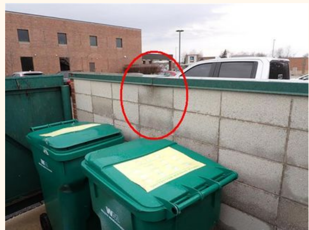
Moisture Stains Below Cap Joint
