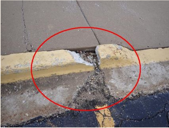
Damaged Curb by Handicapped Ramp
