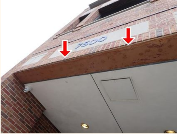
Corrosion on Lintel
