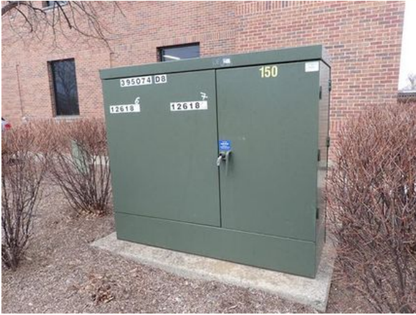
Transformer on East Side of Structure
