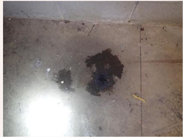
Oil on Floor Below Pump
