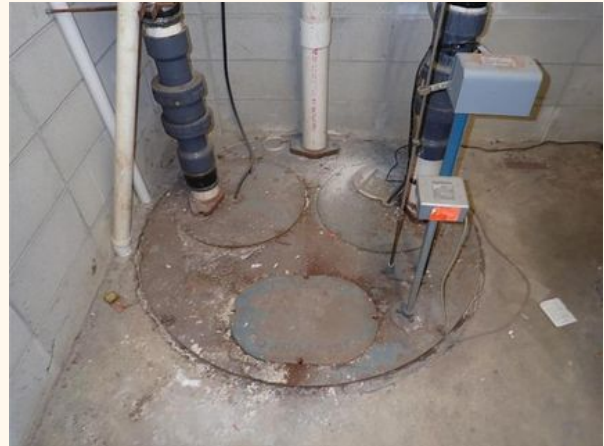
Waste Ejector Pumps in Mechanical Room
