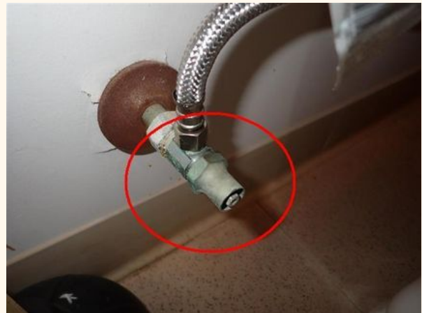
Missing Shut-off on Toilet Supply
