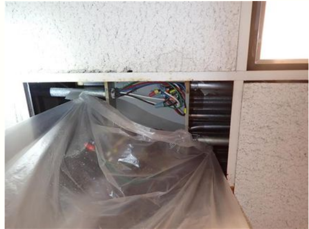
Leakage Stains on Junction Box in Ceiling
