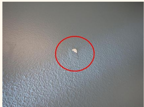
Paint Missing on Walls
