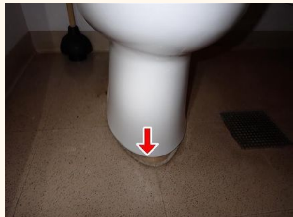
Unsealed Bases on Toilets
