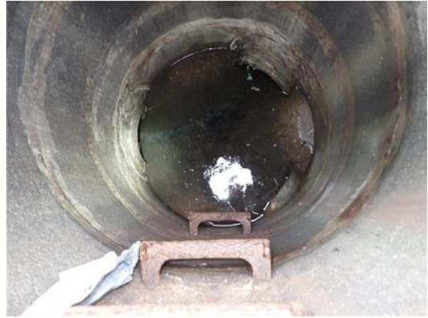
Standing Water in Manhole in Parking Lot
