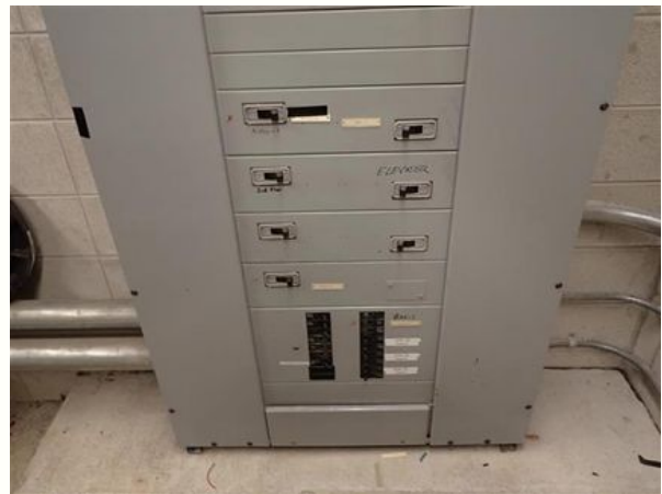
Main Shut-off in Basement
