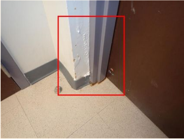
Moisture Stains and Damage by Lower Level Doors
