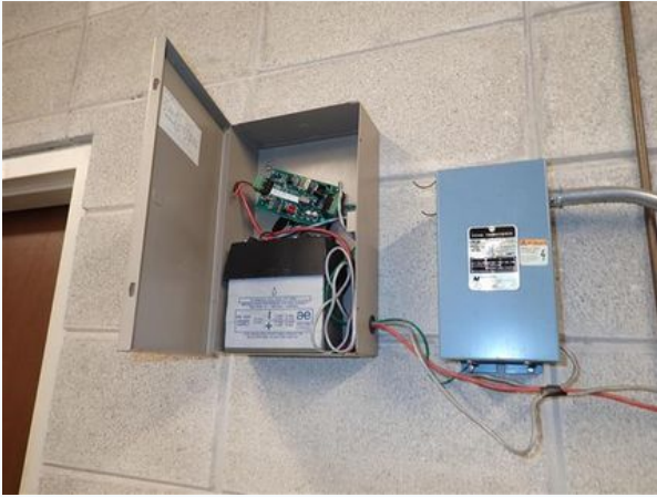
Low Voltage Alarm System
