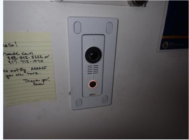
Low Voltage Communication Equipment
