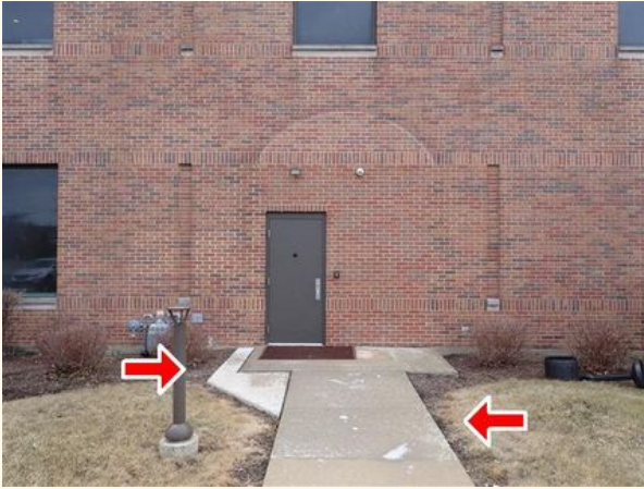
Drop-offs Near Rear Entrance
