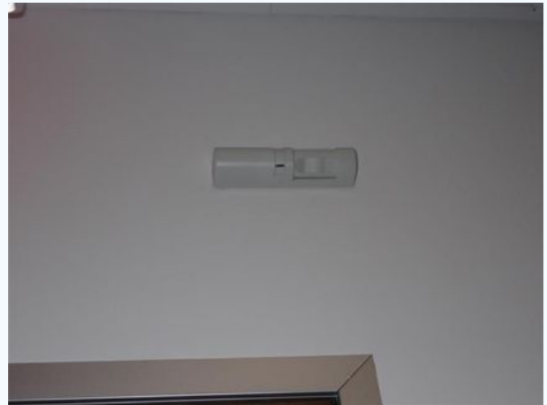
Low Voltage Alarm System
