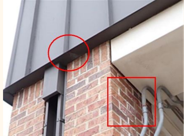
Moisture Stains on Joint
