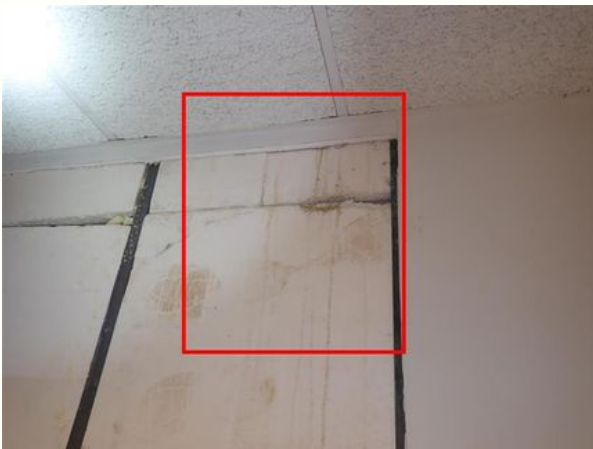
Leakage Stains on Walls
