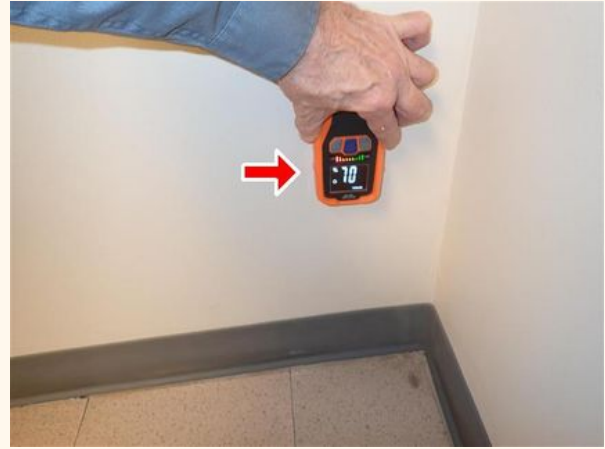
Elevated Humidity in Wall Areas by Elevator
