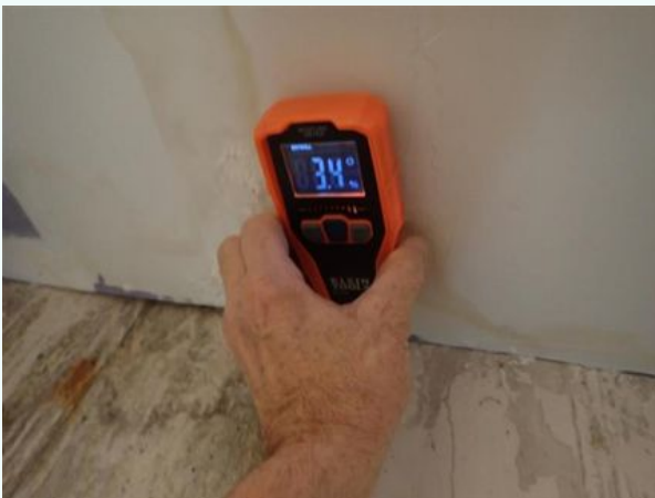
No Moisture by Wall Stain Below Pipe
