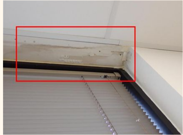
Moisture Stains and Damage Above Windows Noted
