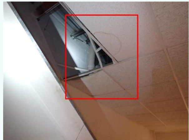
Stains on Ceiling Tile in Former Mail Room
