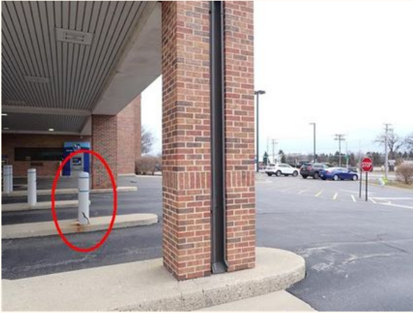
Damaged and Corroded Bollard
