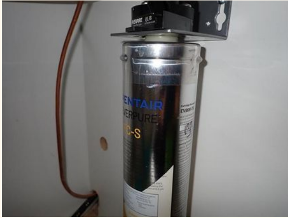
Filtration System in Basement Break Room
