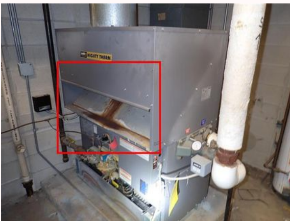
Corrosion on Boiler
