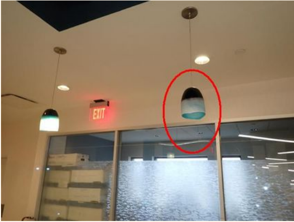
Extinguished Bulb in Light Fixture
