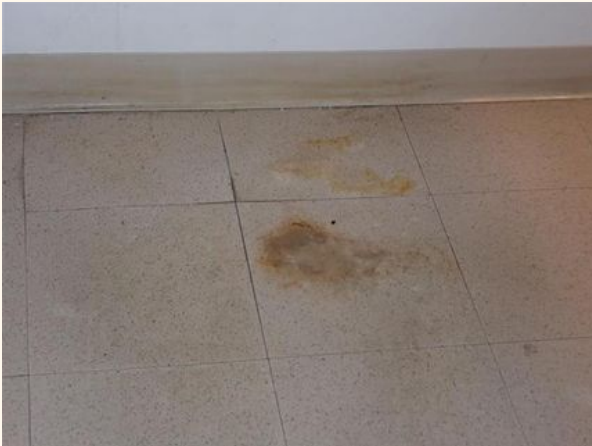
Stains and Warped Tile in Bathroom Tiles Below Urinal
