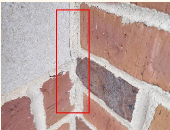
Hairline Cracks in Corner Masonry
