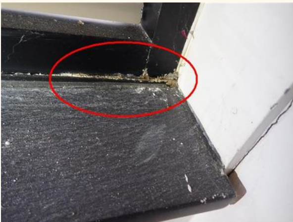
Moisture Related Damage Noted in Corners of Windows
