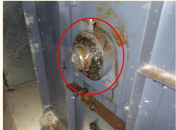
Grease Build-up on Bearings
