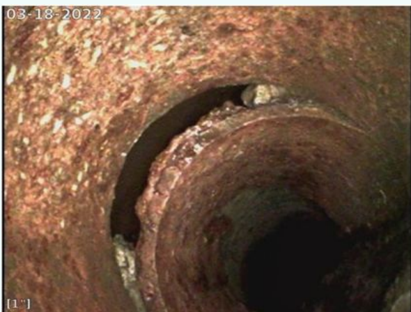
Pipe Separation on Sanitary Main
