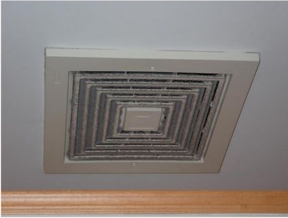
Clogged Vent Fan in Upper Level Bathroom
