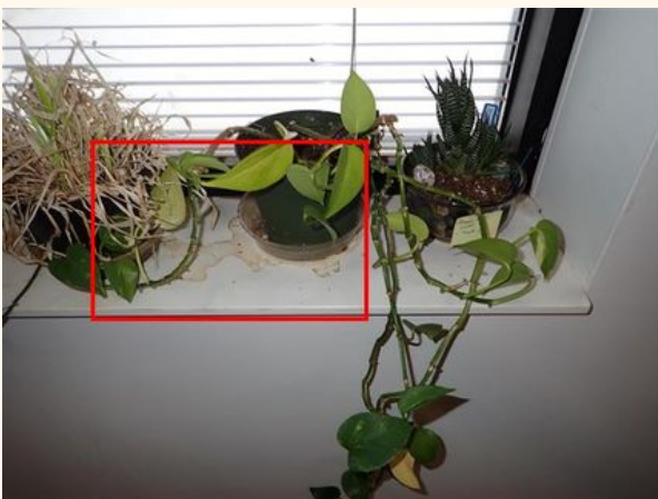
Water Stains on Window Sills from Plants
