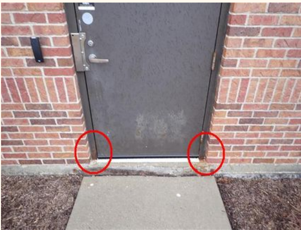
Corrosion on Bottom of Doorframe
