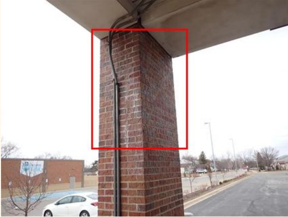
Efflorescent Stains on Column
