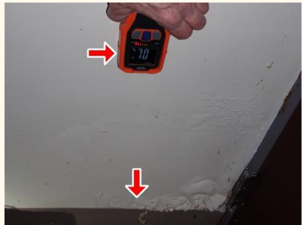
Elevated Humidity Measured Well Above Floor
