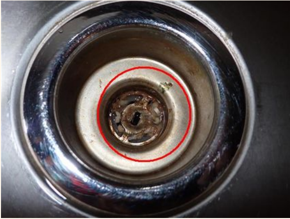
Food Waste Clogging Drain
